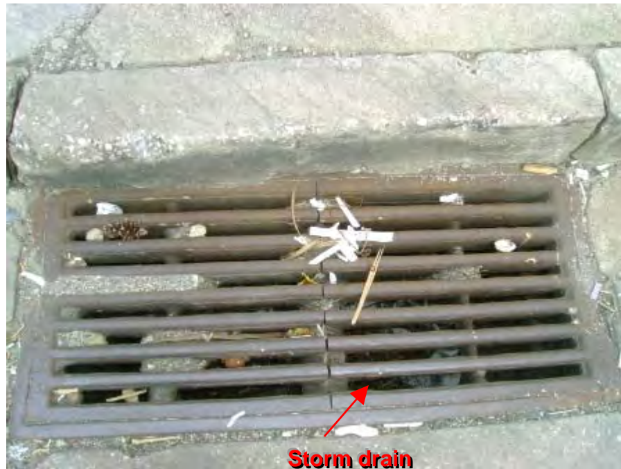
Photograph 58. Northwest Transfer Station – Close up of storm drain in previous photo. (NOTE: Debris and sediment within storm drain)
