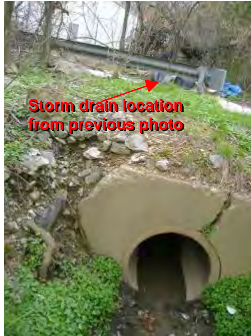
Photograph 9. Clipper Mill Monitoring Location – View of sediment in outfall pipe and channel leading to stream bank. Sediment could be a result of dirt and debris near storm drain in previous photo.
