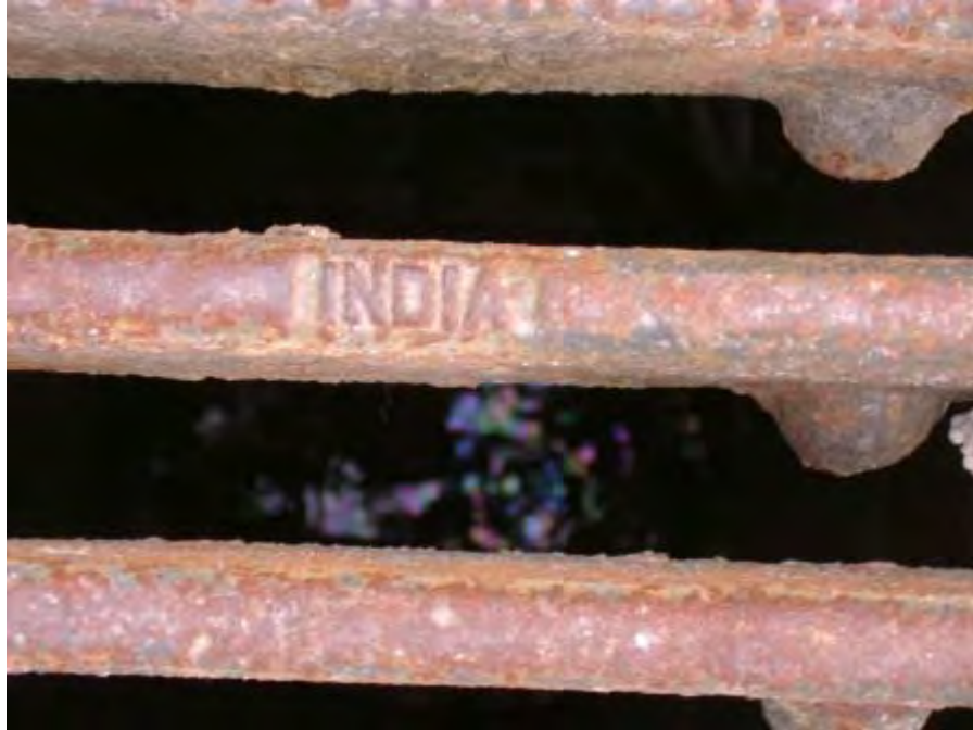
Photograph 67. Northwest Transfer Station – View of sheen on flowing water inside storm drain downstream of larger spill.
