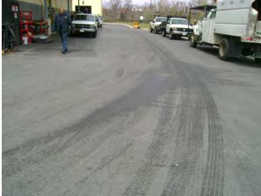
Photograph 31. Central Garage – Example of staining on paved area.
