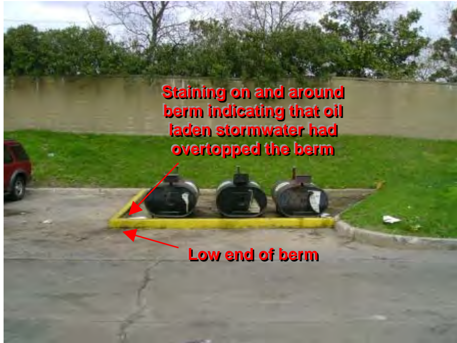
Photograph 47. Northwest Transfer Station – View of waste oil tanks with small berm to contain a spill and there are no BMPs to prevent stormwater contact with the tanks. It appears that a good sized rain event would result in stormwater overtopping the berm as evidenced in next photo.
