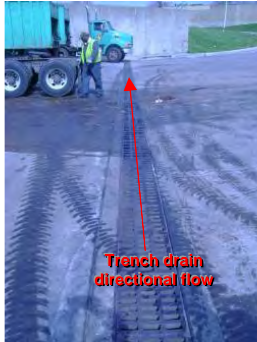
Photograph 63. Northwest Transfer Station – Another view of the larger spill to a trench drain.
