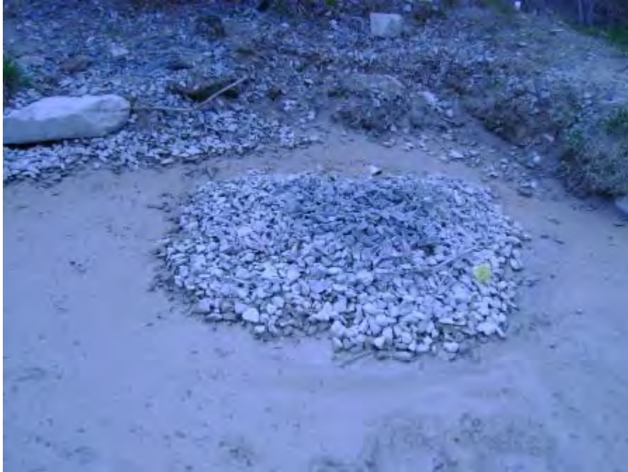
Photograph 13. S&G Concrete – Another view of drain covered with filter fabric and stone.
