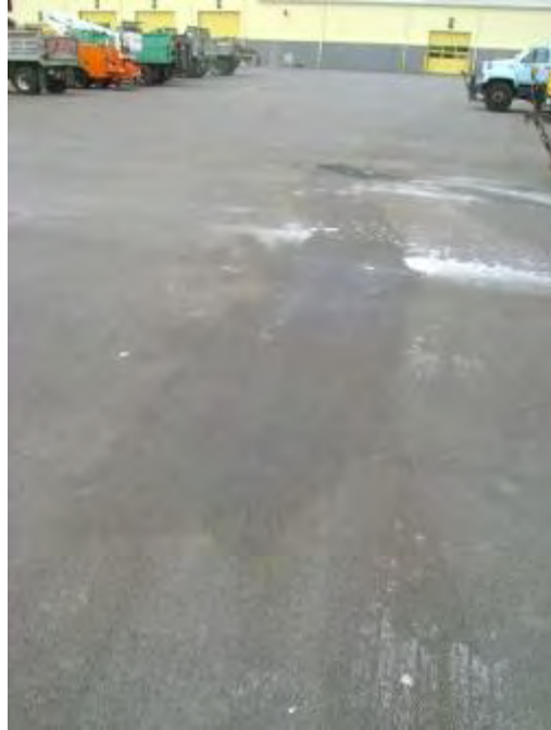
Photograph 25. Central Garage – Example of staining on paved area.
