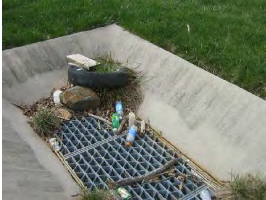
Photograph 5. Girl Scouts of America (SWM Nos. 56 and 180) – View of trash and debris accumulation at inlet structure appurtenant to detention facility.
