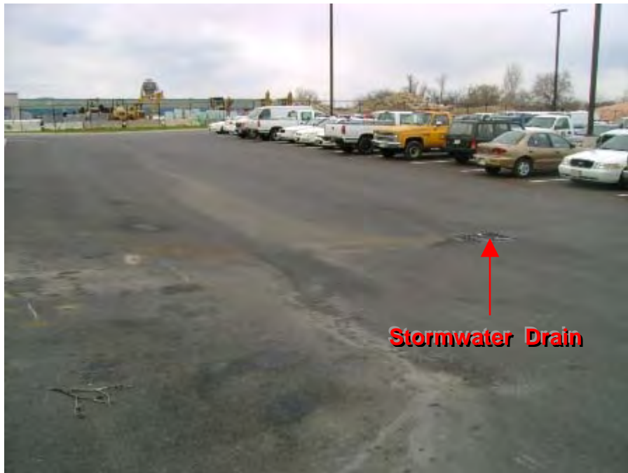
Photograph 32. Central Garage – Example of staining on paved area with stains evident into storm drain.
