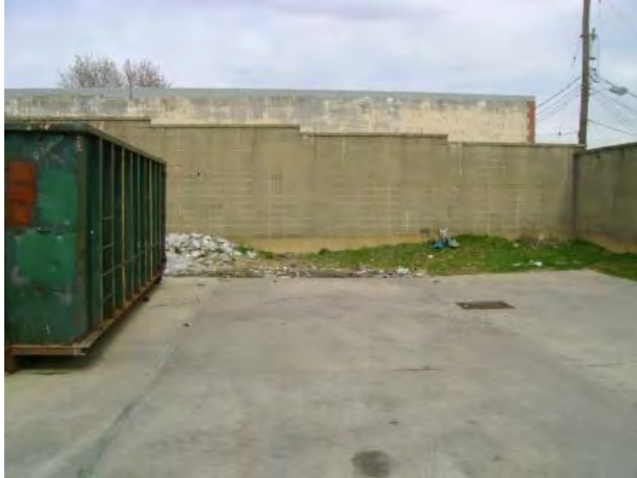
Photograph 69. Northwest Transfer Station – Another view of storm drain from previous photos noted downstream of larger spill. According to City personnel, the dumpster to left was previously used for the collection of tailings from street sweepers which would potentially result in an illicit discharge to the City’s storm sewer system. No street sweeping storage was noted during the visit.
