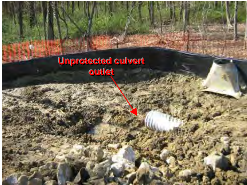
Photograph 6. Cylburn Arboretum – The approved ESC plan specified the implementation of culvert outlet protection, but flow dissipation BMPs were not in place below the culvert outlets.
