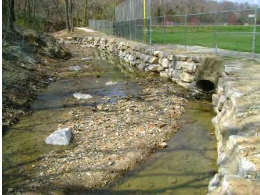
Photograph 77. Maiden's Choice Stream Restoration Project – View of stream restoration activities. (NOTE: Retaining wall and new outfall along bank)
