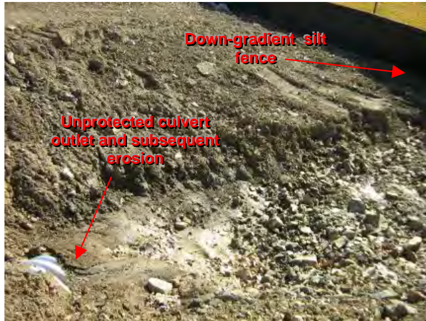
Photograph 7. Cylburn Arboretum – Silt fence BMPs had been improperly selected and implemented in an area of concentrated flow down-gradient of the culvert outlets.
