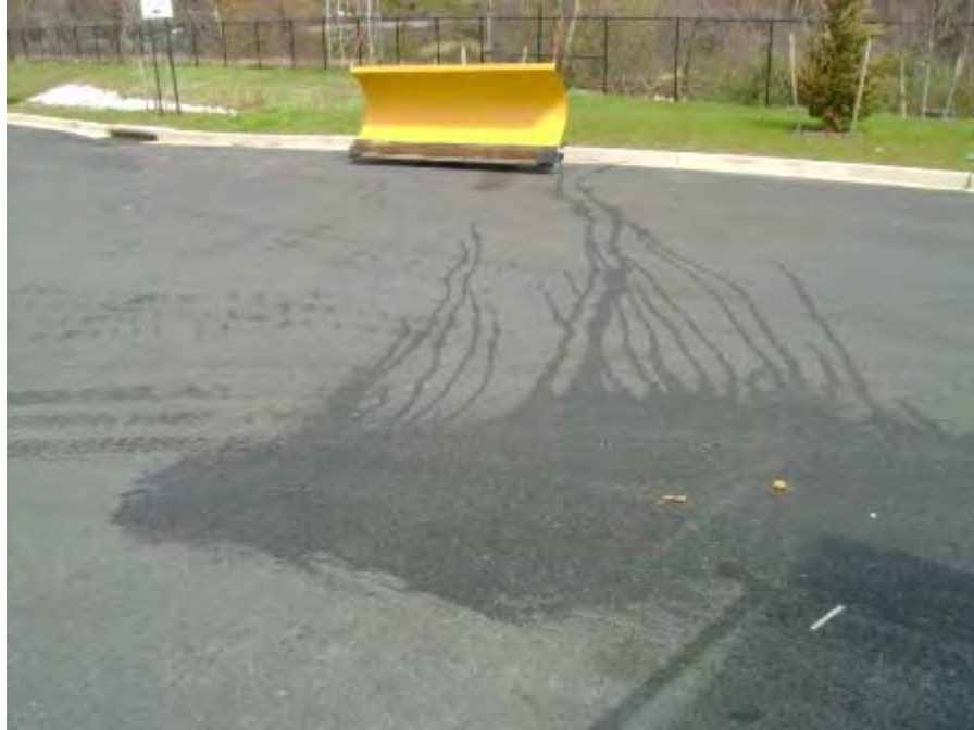
Photograph 29. Central Garage – Example of staining on paved area.
