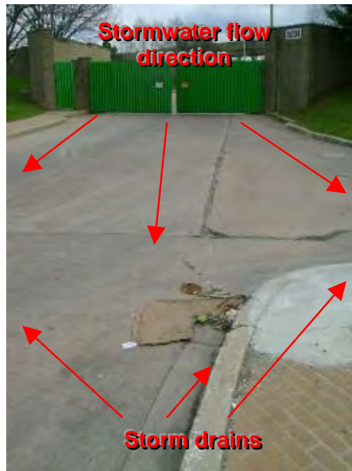
Photograph 56. Northwest Transfer Station – Facility entrance. (NOTE: Debris and sediment within storm drains)
