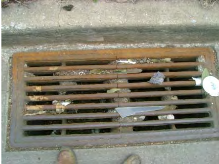
Northwest Transfer Station – Close up of storm drain in previous photo approximately 75% full of debris and sediment.
