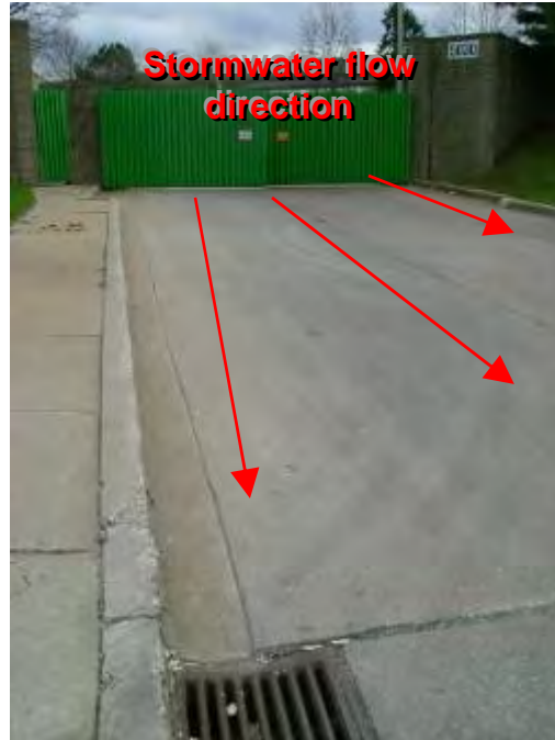
Photograph 57. Northwest Transfer Station – Facility entrance. (NOTE: Debris and sediment within storm drain)
