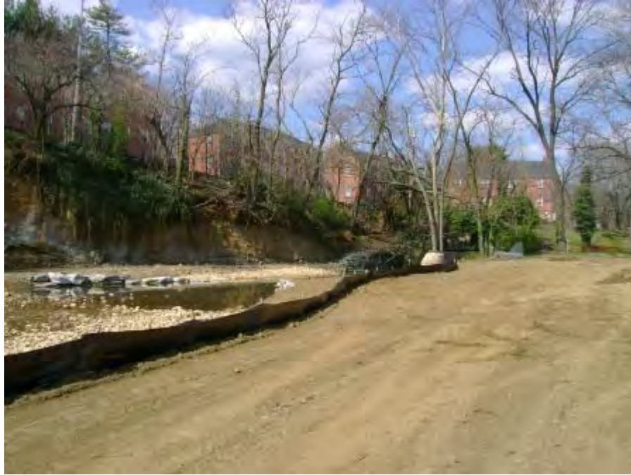
Photograph 75. Maiden's Choice Stream Restoration Project – View of silt fence along stream restoration project.
