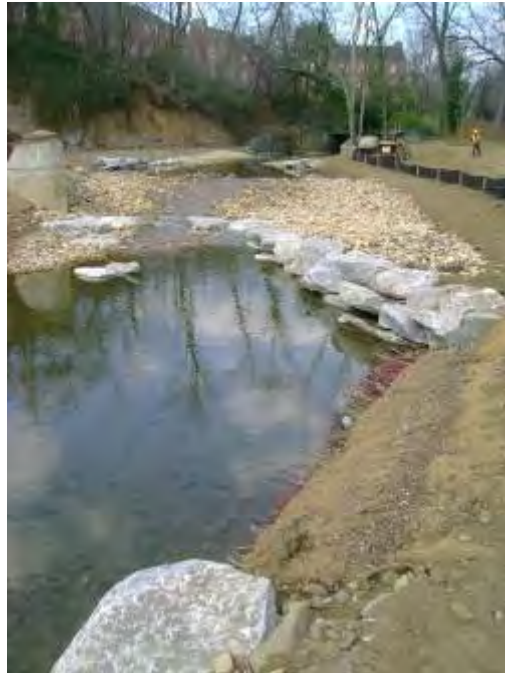
Photograph 76. Maiden's Choice Stream Restoration Project – View of stream restoration activities. (NOTE: Boulders and vegetation along bank)
