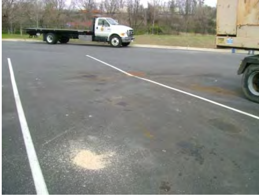
Photograph 27. Central Garage – Example of staining on paved area and absorbent left on spill.
