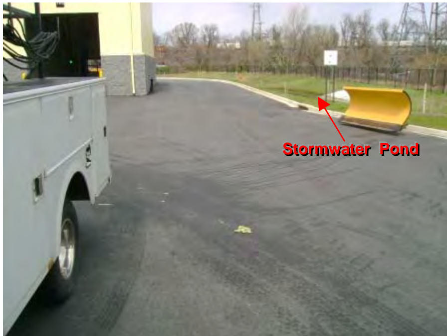
Photograph 30. Central Garage – Example of staining on paved area.
