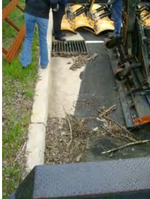
Photograph 37. Central Garage – View of debris around around storm drain.
