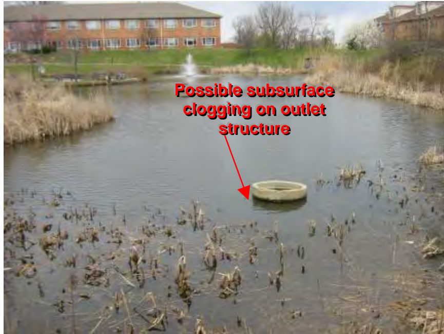
Photograph 3. Good Samaritan Nursing Center – Review of as-built plans indicated the potential for prolonged water storage.
