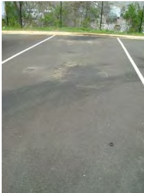
Photograph 36. Central Garage – Example of staining on paved area.
