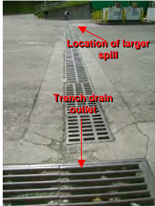
Photograph 65. Northwest Transfer Station – View of the trench drain and trench drain outlet.
