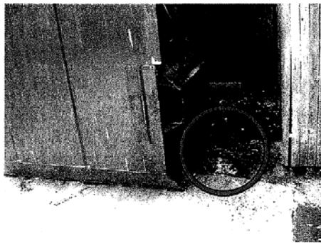
“Dumpster juice” has direct access to the storm drain
