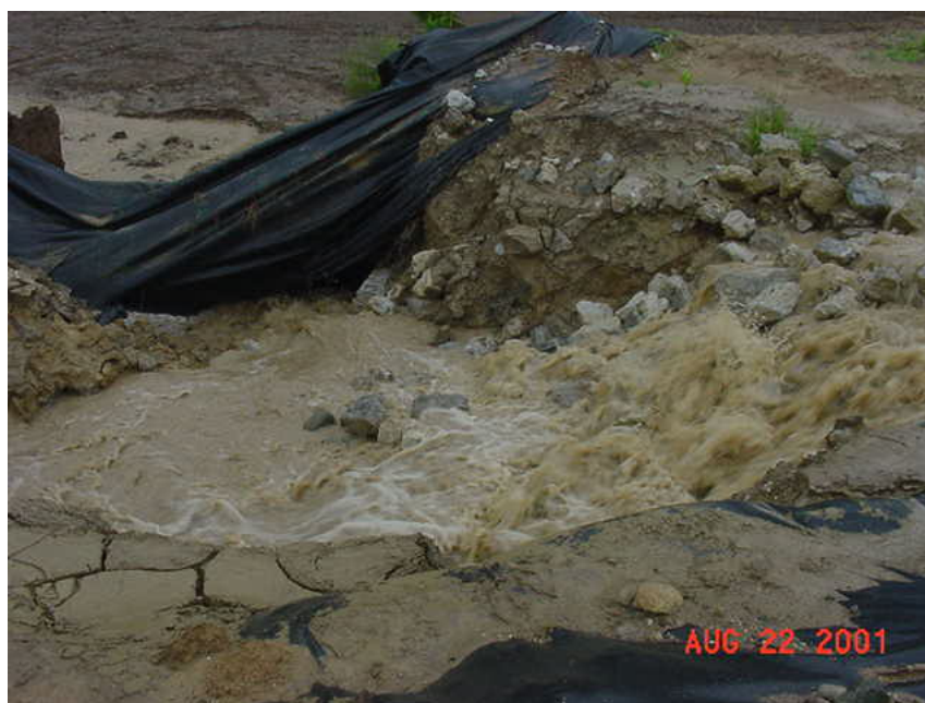
Photo 1: Improperly installed silt fence
