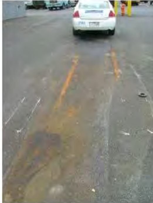
Photograph 15. Central Garage – Example of staining on paved area.
