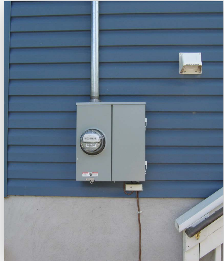
Elevated utilities in Yardley Borough, Bucks County, PA (from PEMA)
