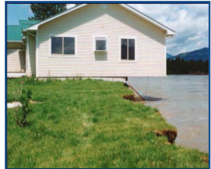
Clark Fork River, outside of Plains, Montana. Originally house was 30-40 feet from river bank and 1" above BFE.
