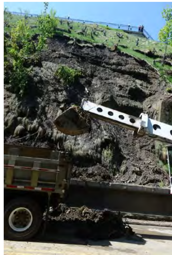
Figure 4.3.5-3 2014 Landslide Damage on PJ McArdle Roadway.
