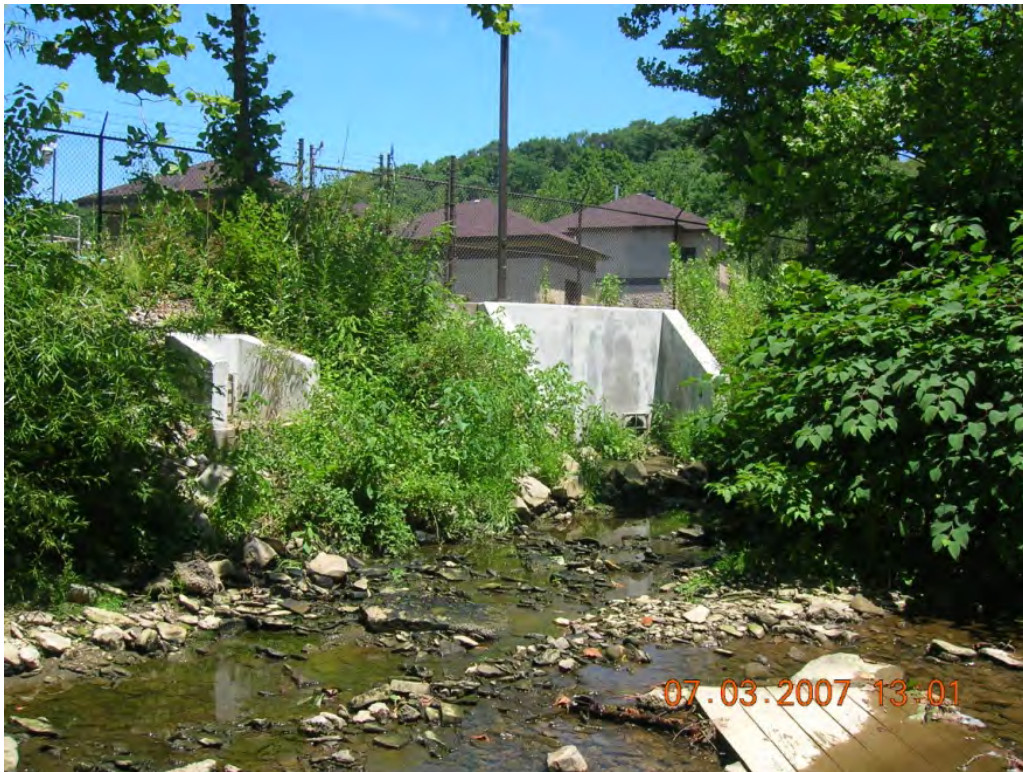
Photo 2: Sewage treatment plant. (BSC-36)
