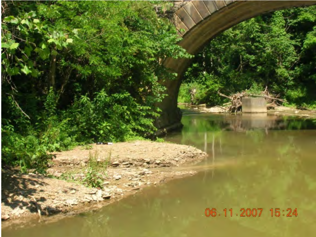
Photo 2: More evidence of debris piling up on concrete in the stream. (BSC-26)
