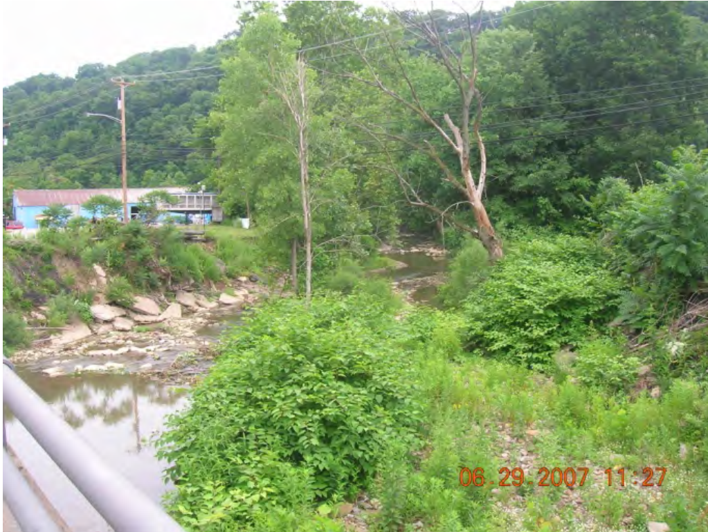
Photo 2: Right side of bridge by Zassick's Auto is silted in. (BSC-33)
