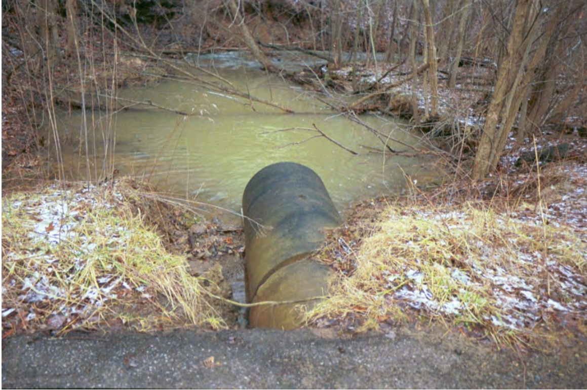
Photo 3: Severe erosion around concrete pipe that is improperly sized. (NF-T5W7)
