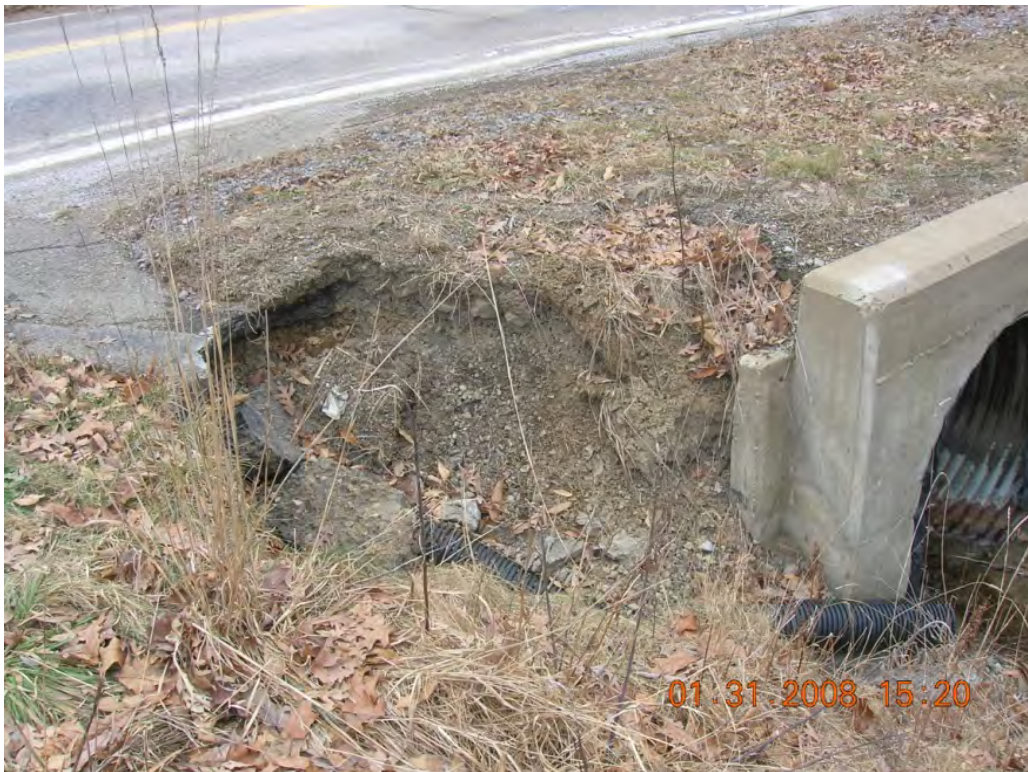
Photo 1: Roadside cave-in that is causing excess sedimentation in the stream during rain events. (NF-40)
