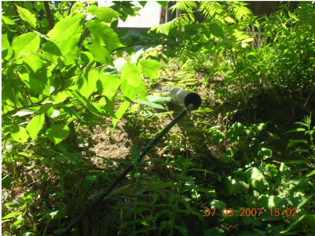
Photo 1: Black pipe with hose coming off of Chem-Dry property. (BSC-46)
