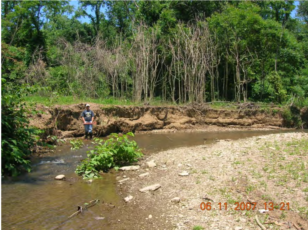
Photo 1: A six foot high by 100 foot long section of streambank erosion. (BSC-12)
