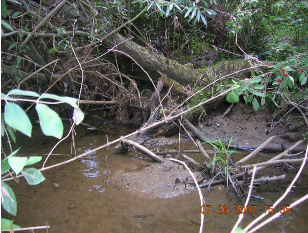
Photo 2: The confluence of Rippling Run with the East Branch is jammed with debris and excess sedimentation. (EF-06)
