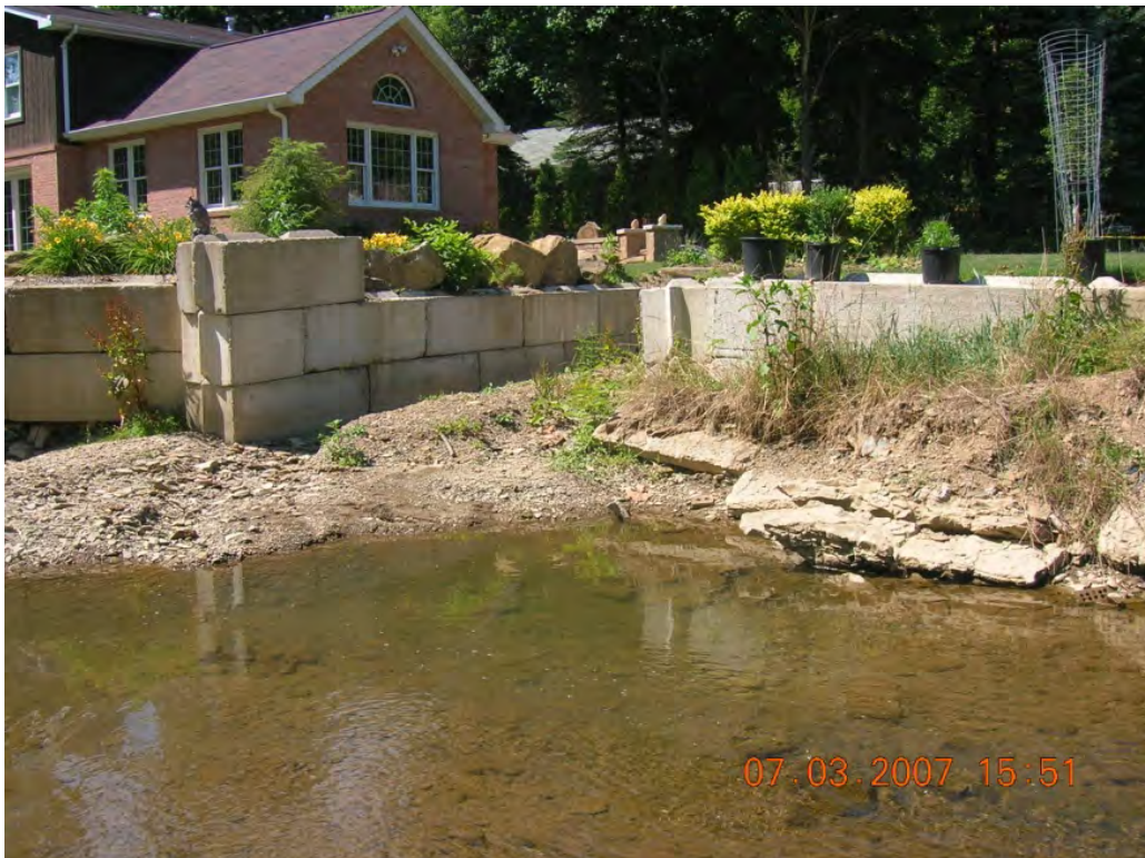
Photo 5: Location of the mouth of Cooney Hollow. Homeowners are encroaching the stream with concrete blocks. (BSC-50)
