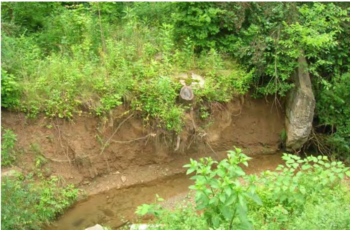
Photo 4: Bank erosion occurring across the road from Beadnell Drive. (BSC-T1E4)
