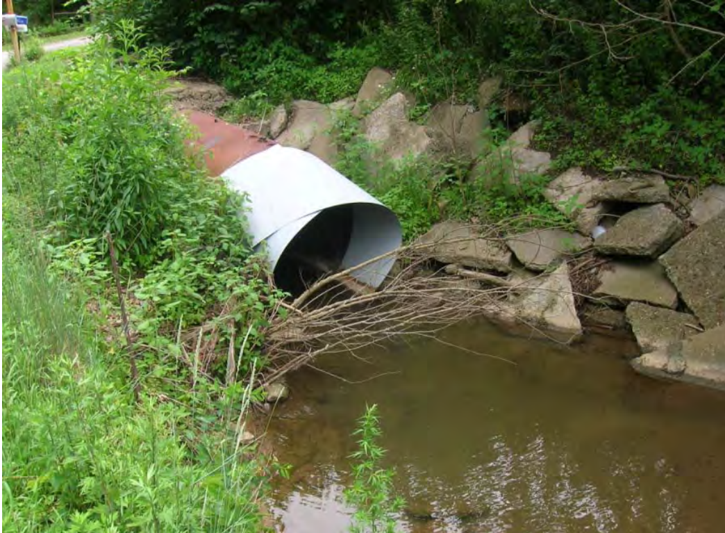
Photo 1: Here, an old tank was improperly used as a driveway culvert on a tributary that runs along Turkeyfoot Road. (BSC-T1E3)
