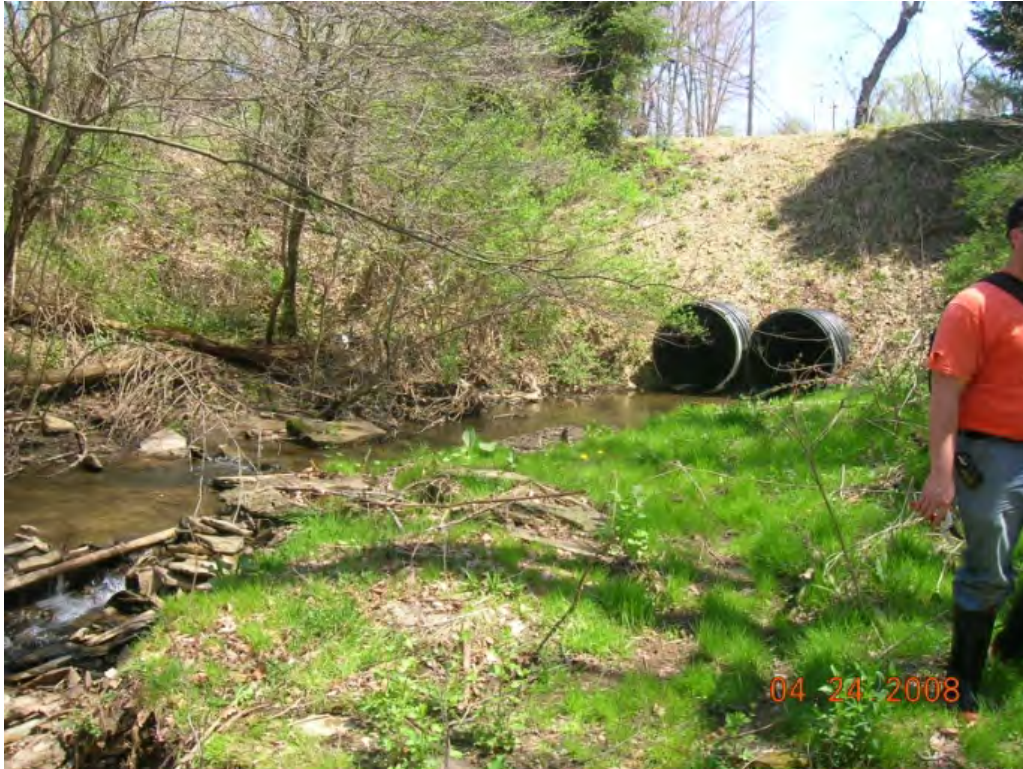
Photo 1: Culverts under a driveway that seem properly sized on Rippling Run. (RR-06)
