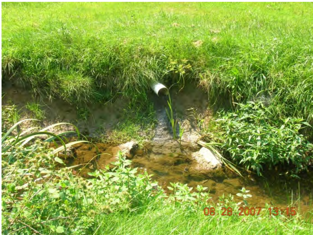
Photo 1: A white pipe discharging fluids with white precipitate out of a front yard. (EF-26)
