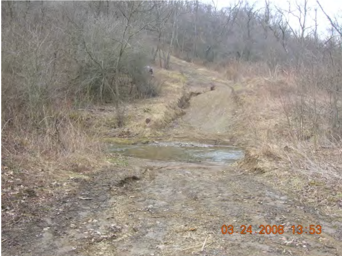
Photo 2: Another instance of erosion just upstream from a large gully on ATV trail. (NF- T2W8)
