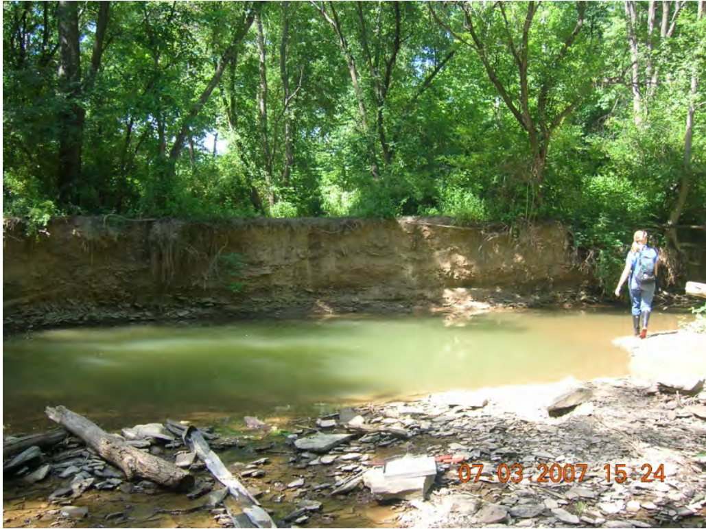
Photo 4: Seven foot high bank erosion and a deep greenish colored pool. (BSC-48)
