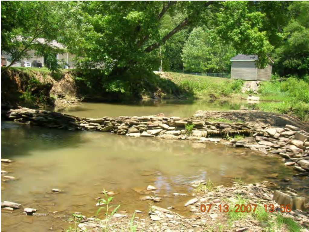
Photo 1: Man-made rock dam creating bank erosion in the bend on the left. (BSC-64)
