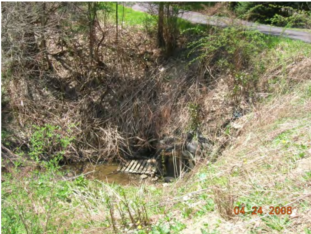
Photo 2: However, the inlets to these culverts are jammed with debris. (RR-06)
