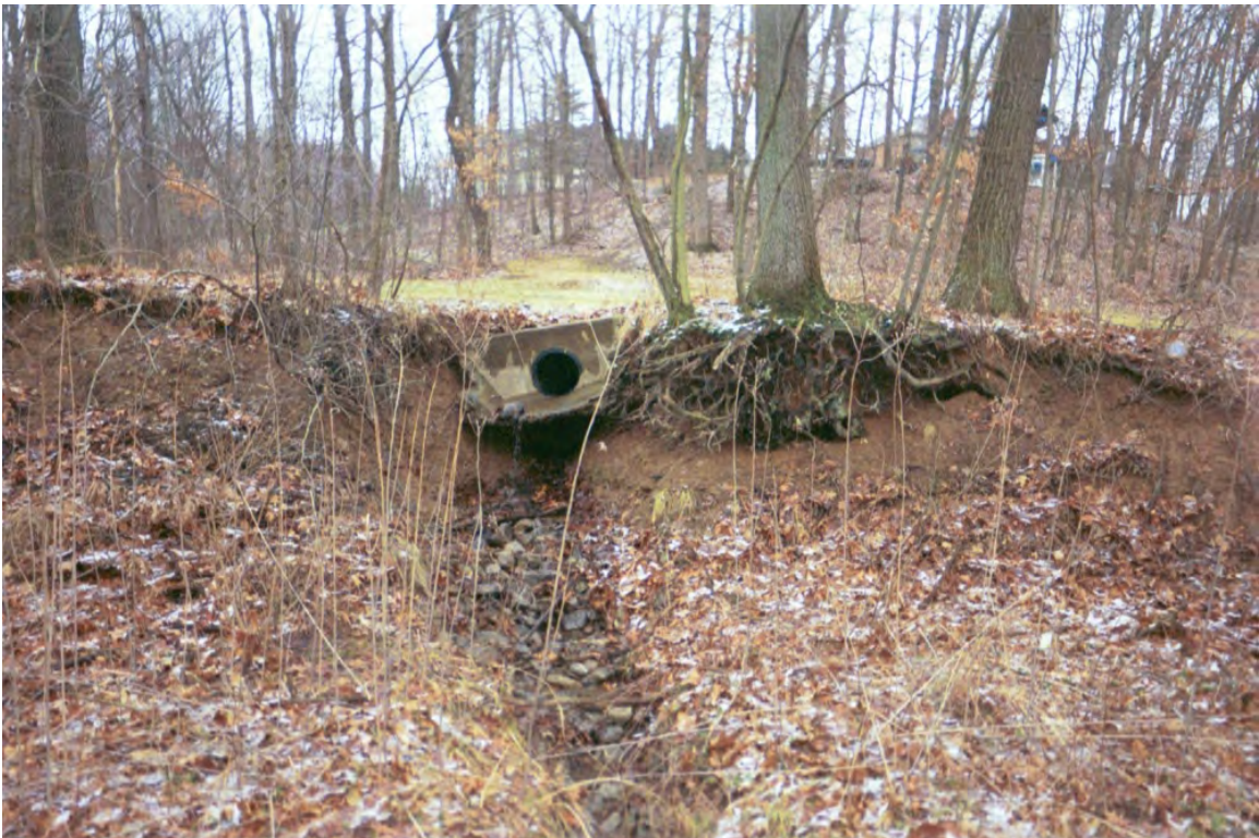
Photo 2: A storm water outlet that needs reconstructed. (NF-T5W6)
