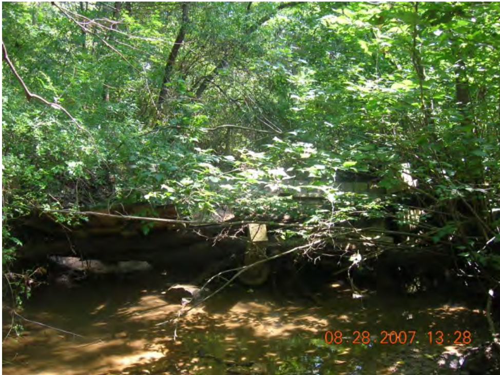
Photo 1: A collapsed wooden bridge creating a debris jam. (EF-29)
