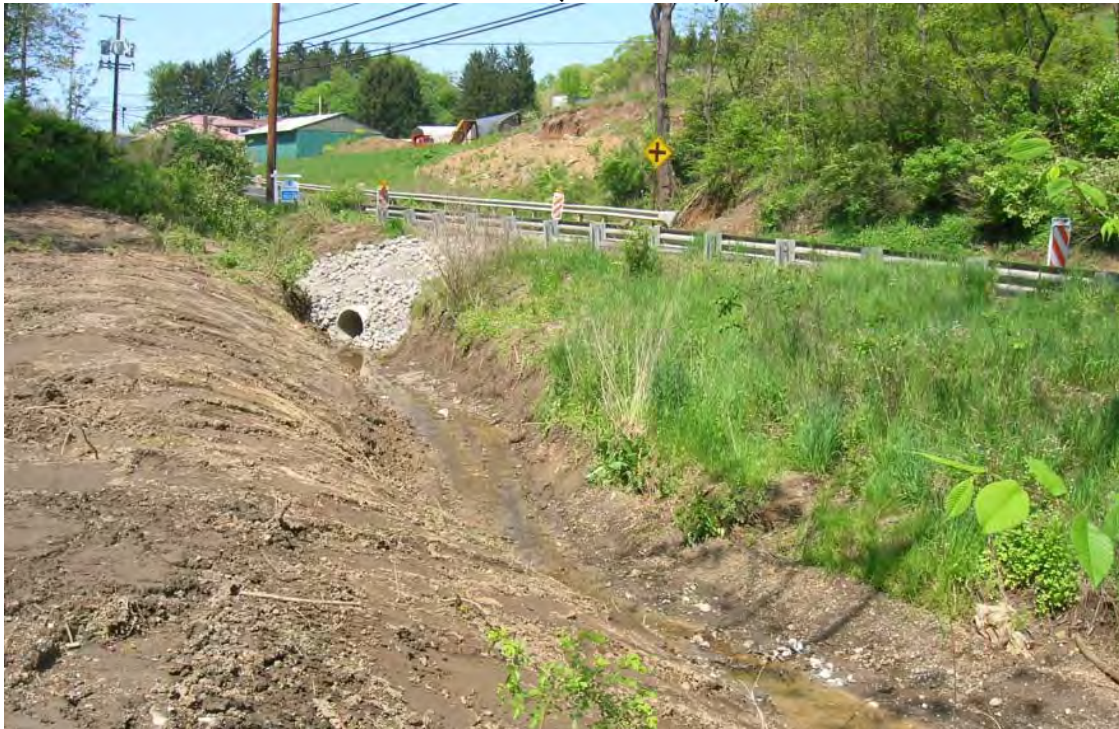
Photo 2: Culvert across Conway-Wallrose Road, leading to headwaters. Recent construction near the Economy VFW was leading to excess sedimentation in the tributary. (BSC-T4W3) ( Eastern Tributaries )
