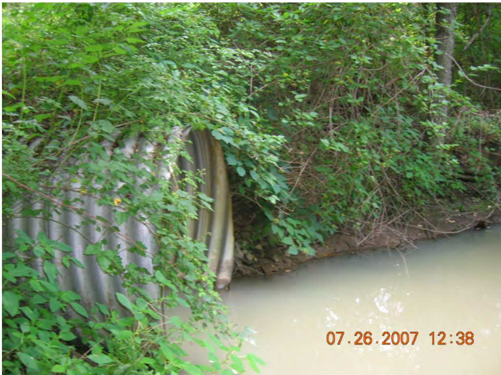
Photo 5: Improperly sized culvert squeezing the channel. (BSC-94)
