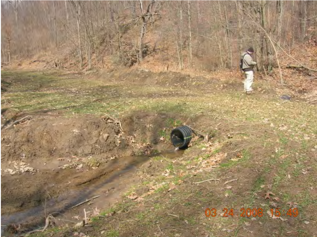
Photo 1: A stream crossing culvert causing down cutting and erosion. (NF-T3W2)
