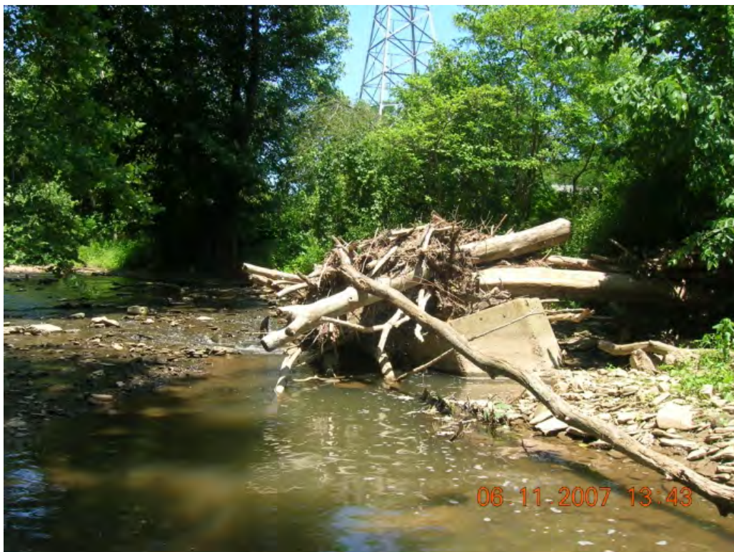
Photo 2: Debris piling up on concrete in stream. (BSC-14)
