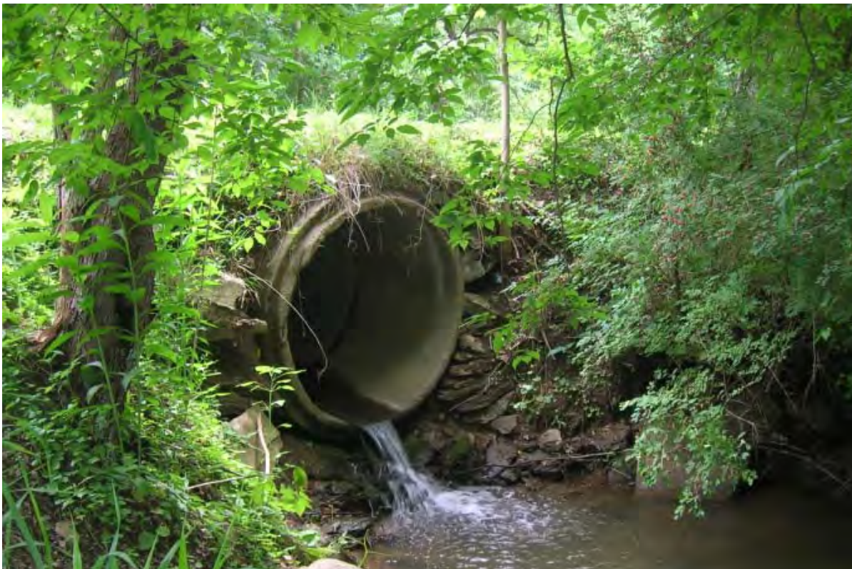
Photo 6: Culvert under Sevin Road at intersection with Turkeyfoot Road placed too high. This creates a passage fish barrier. (BSC-T1E6)
