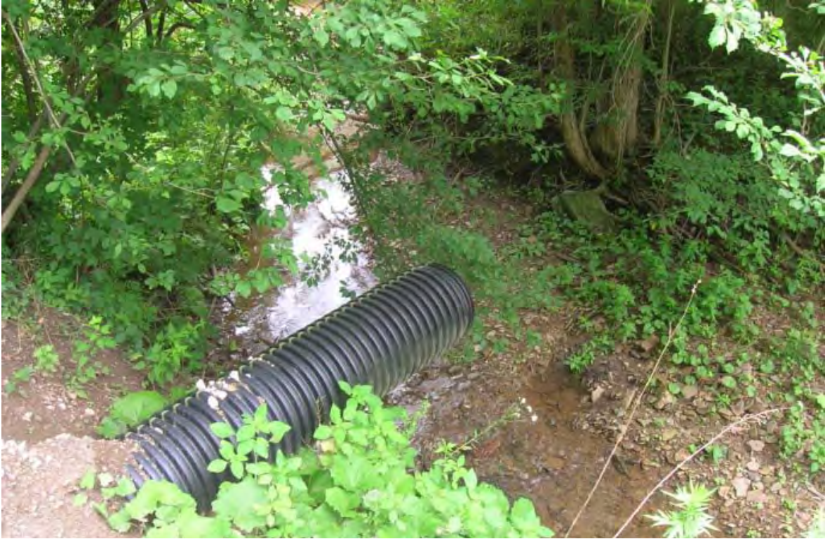
Photo 5: Storm water outfall that is sticking out too far into the stream channel. (BSC-T1E4)
