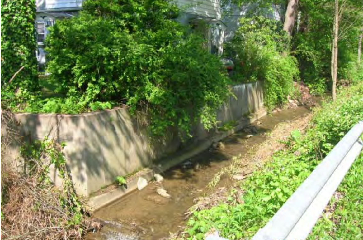
Photo 1: Tributary along Shaffer Road squeezed by the road and a concrete retaining wall. (BSC-T3W2)
