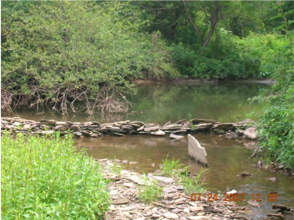
Photo 2: Rock dam contributing to sediment bar problem due to reduced water flow. This has been removed as of 10/05/10 field check (BSC-69).
