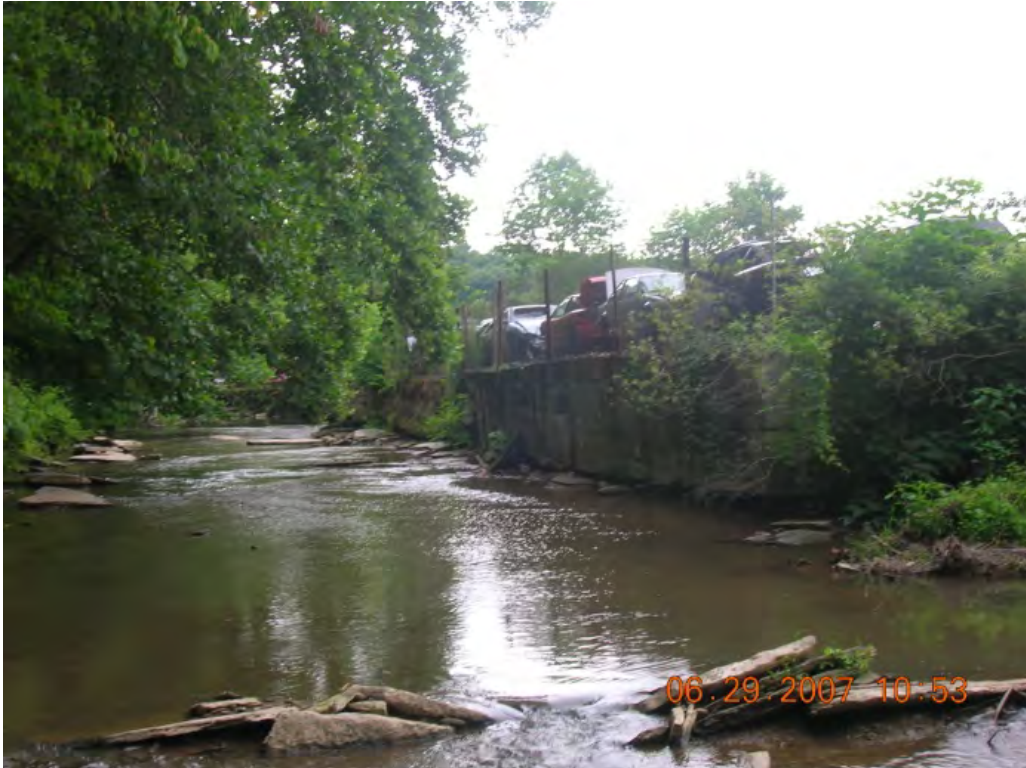
Photo 1: Concrete wall at Ed Wagner Auto Salvage constricting channel. (BSC-30)
