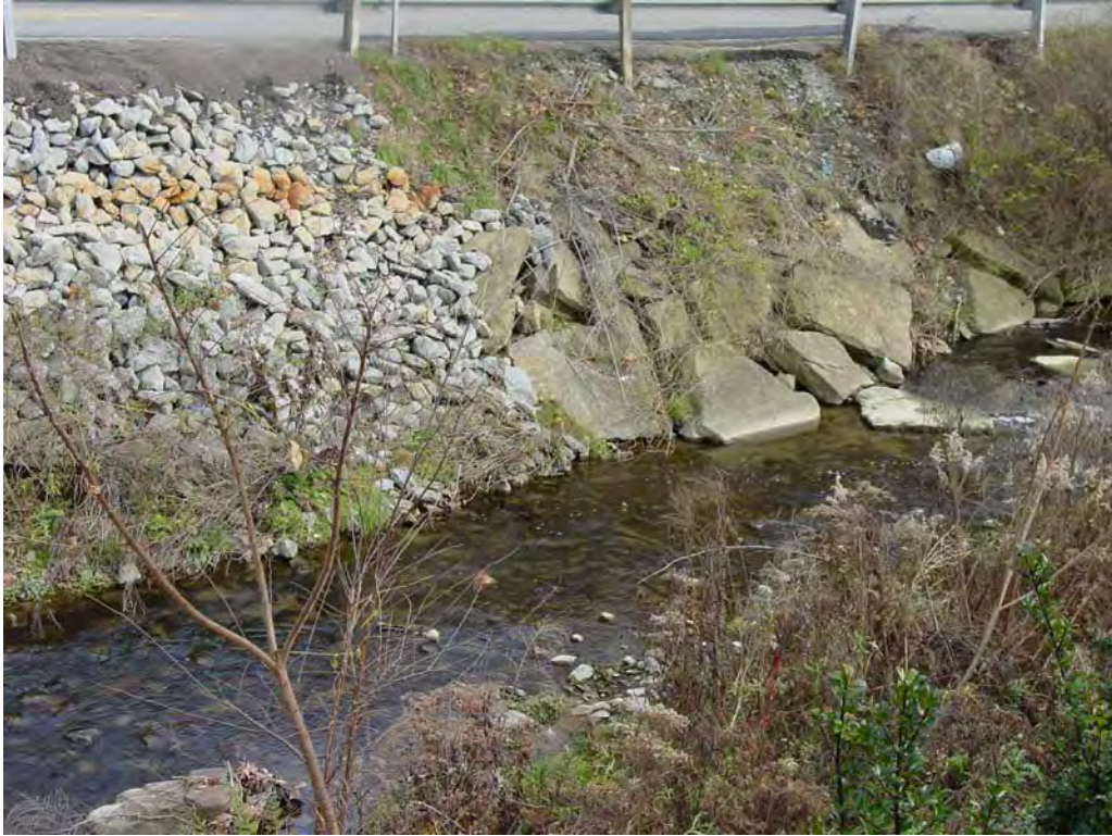
Figure 6 - Typical of the armored banks necessary to convey high water events without causing damage to roads.
