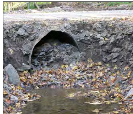
An inadequately designed culvert and endwall from a Buck Run tributary filled with sediment after a flood in 2004.
