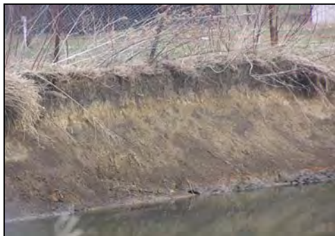
Severe erosion along a section of Buffalo Creek, resulting in significant loss of streambank each year
