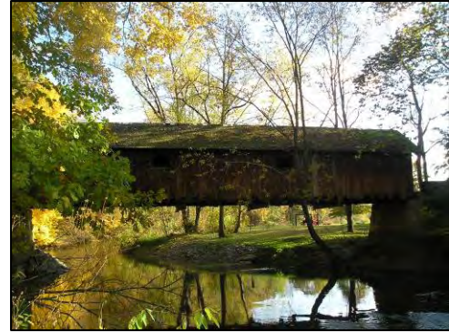
Woolslayer Bridge extends 75 feet across Brush Creek in New Sewickley Township, Beaver County
