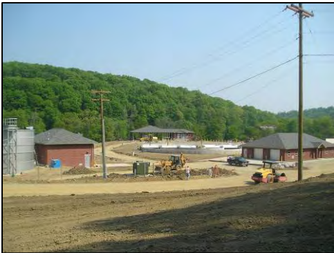
Saxonburg Area Sewage Treatment Plant
