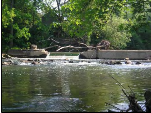
Breached dam on Connoquenessing Creek
