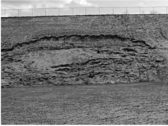
Figure 13. Small slump in the cut portion of a recent cut-and-fill slope. The slumped material is a thick claystone between layers of stronger rock.
