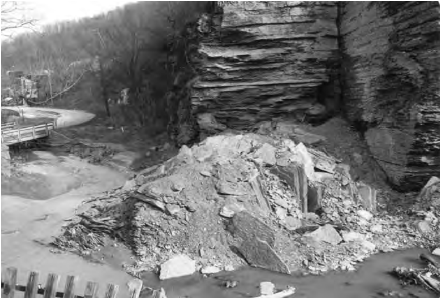
Figure 19. Rockfall from a cliff face into a stream channel. Note how the rock has fallen away along near-vertical joints, forming fresh cliff faces. Photograph by J. L. Craft.
