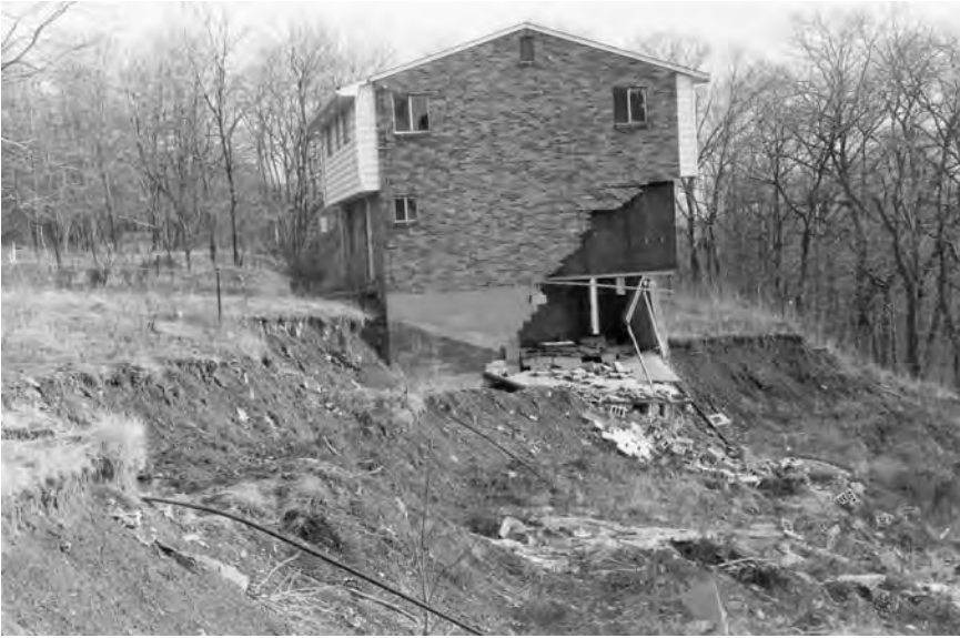
Figure 22. A new home that was severely damaged, and eventually totally destroyed, by slope failure. The remains of the home (since demolished) are at the head of an active slide developed in fill material placed on top of old landslide materials. Photograph by J. L. Craft.
