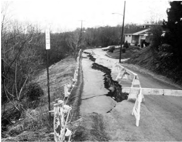
Figure 20. Slump failure of a road on a cut-and-fill slope.
