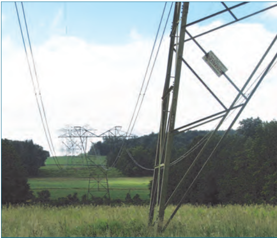
Figure 4.27: Transmission lines, Brush Valley Township
