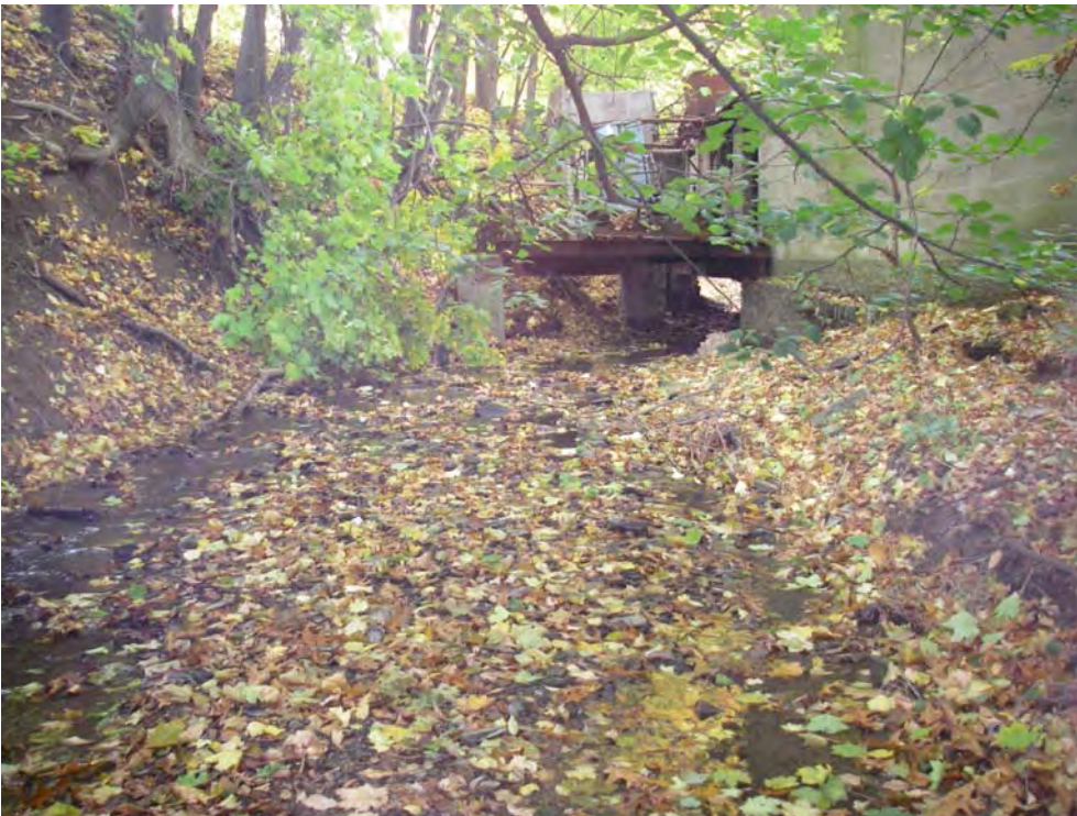
Photo 12: Sherrick Run – Bank erosion
