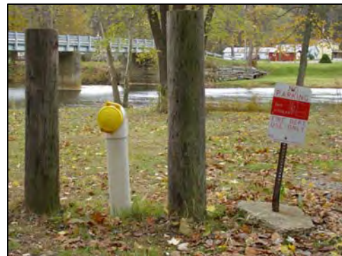
Dry hydrant located at Putneyville Park is used by firemen needing access to water in emergency situations where there is no public water system and a lack of fire hydrants
