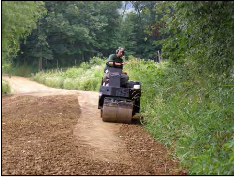
Mottarn road dirt and gravel road project during construction phase in July 2008, where 11 culverts were installed and the roadway was re-graded
