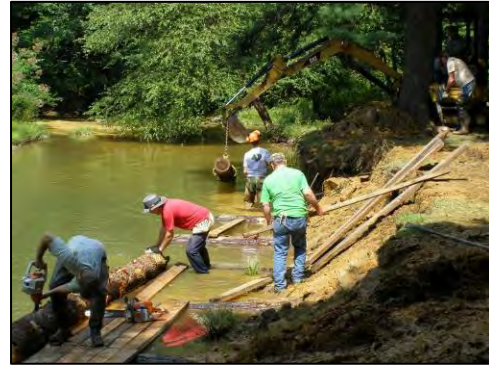
WPC and volunteers installing streambank stabilization and habitat structures on a tributary to Little Mahoning Creek
