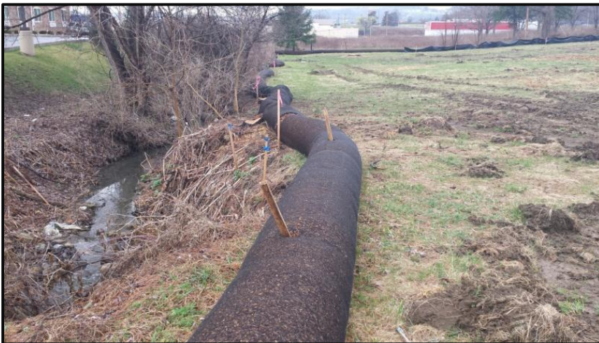
Figure 7: Filter sock used to provide erosion and sediment control (Source: Westmoreland Conservation District)
