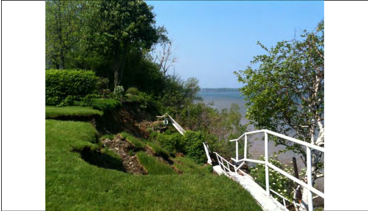
Figure 4.3.1-4 Photograph of Collapsed Retaining Wall Structure along the Lake Erie, PA Shoreline (PA DEP, 2011).
