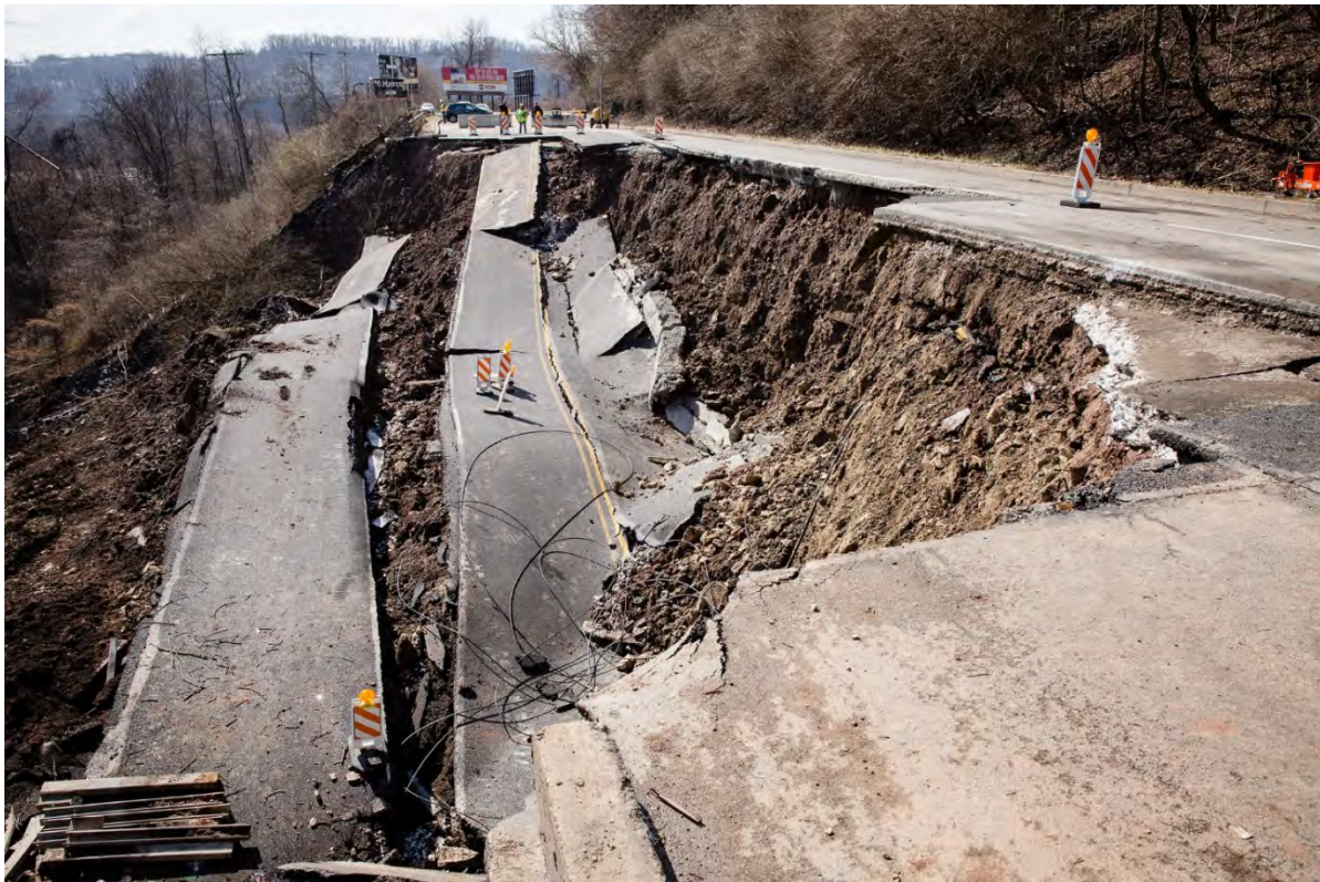
Figure 4.3.9-3 Photos showing damage to a private home (left) and PA Route 51 (right) due to landslide incidents.
