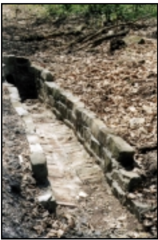
Decaying and inadequate drainage infrastructure, like this channel, are not sufficient to handle modern demands.
