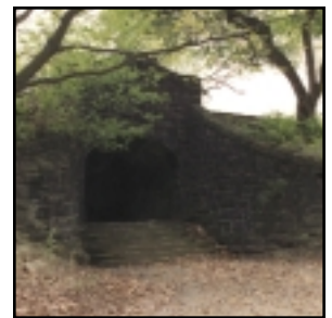
The Pedestrian Underpass today - unfortunately many wonderful elements are in need of repair.
