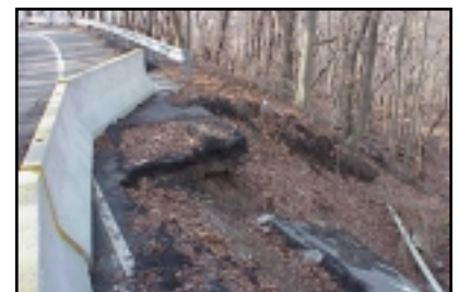
Portions of Riverview Drive are crumbling, probably due to inadequate drainage. Great effort and expense is required to maintain this road. This could be remedied by converting the road to a trail.
