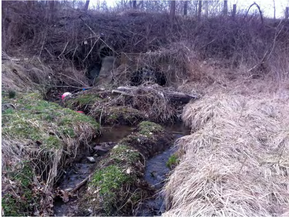
SH67 – A stormwater culvert in need of maintenance and an undersized culvert carrying Sleepy Hollow Run under Kings School Rd meets a debris jam at culvert exit and results in excess erosion both downstream and upstream of the culvert.
