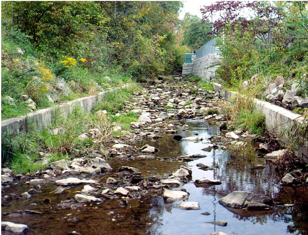
CRB03 – The Clifton Road branch of Piney Fork is channelized for approximately 120 feet at the lower end of Simmons Park. Severe bank erosion occurs downstream of the culvert.
