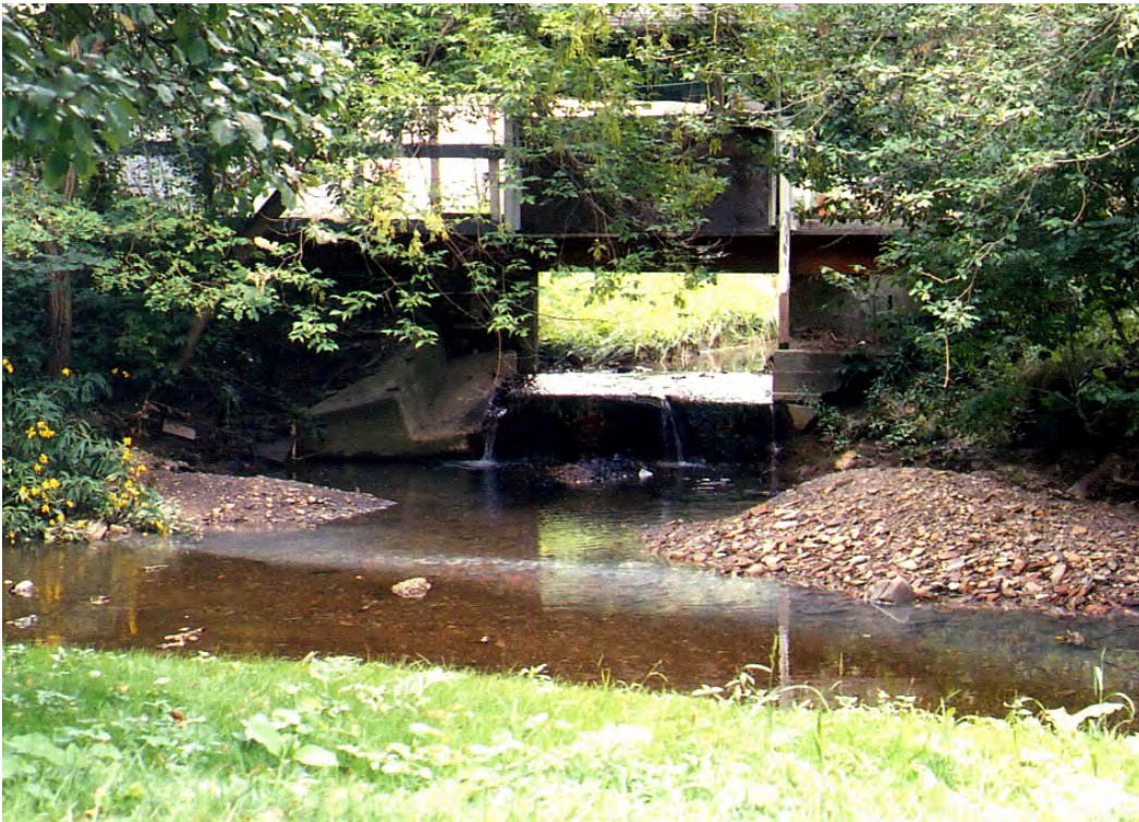
LR40 - Mineral Run Tributary enters Lick Run's right ascending bank just west of Cochran Mill Rd near its junction with Stilley Rd. This tributary is impacted by several AMD discharges depicted below.
