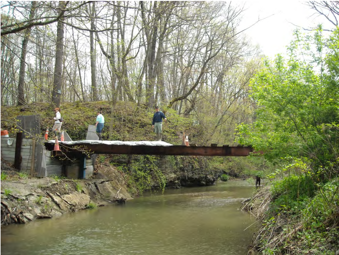
PCU037 – Homeowner bridge crossing of Peters Creek. Concrete poured along stream eroding into creek. Non-functional vehicles and other debris within floodplain of stream.
