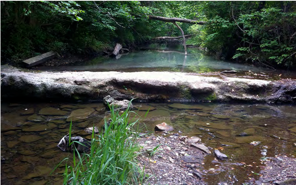
PF65 – a low dam across Piney Fork just below an AMD discharge near Cardox Road's junction with Brownsville Rd. The dam is most likely remnants of infrastructure associated with the Montour 10 Mine.
