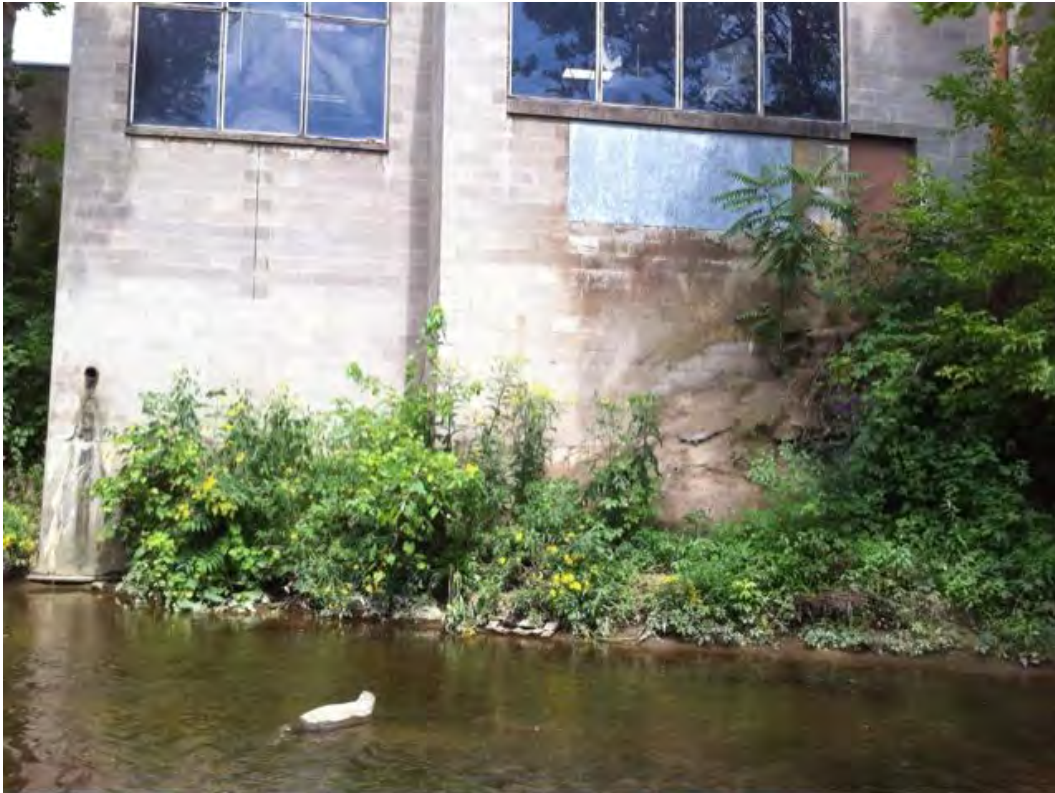
PCM05 - Dick Corporation Building encroaches on Peters Creek's channel at the eastern end of the Middle sub-watershed. A number of outfalls also drain from the building directly into the creek.
