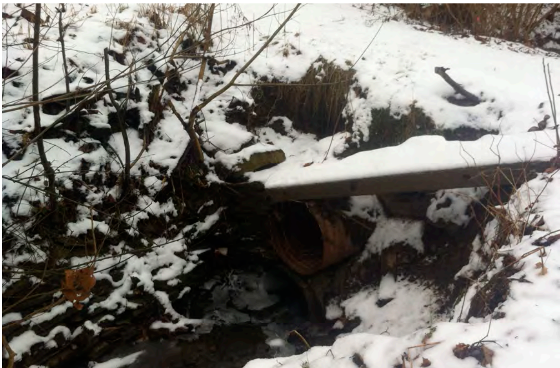
SCR11 – Scotia Run is culverted under a pedestrian access trail to a billboard along Route 51. Two culverts are placed one on top of the other. They are incorrectly sized for the given flow during rain events and are causing the trail to erode and are also creating bank erosion upstream.
