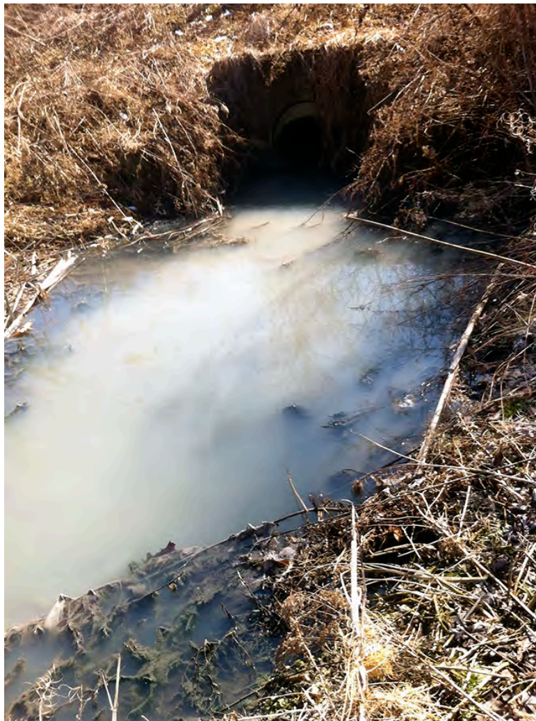
BR64 – Input into a stormwater detention basin along Beam Run Rd appears to be impacted by sewage.
