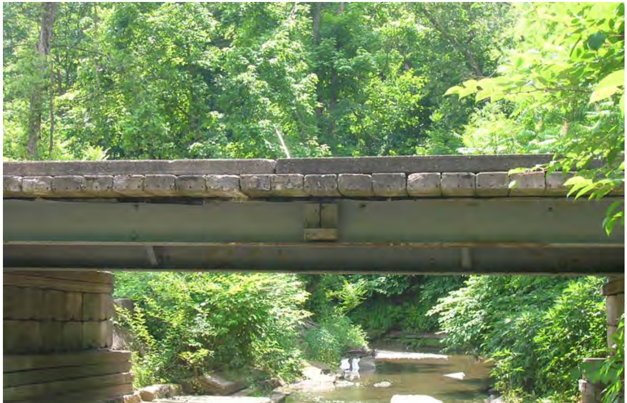
LR44 - A homeowner bridge crossing of Lick Run along a section of stream that runs primarily along bedrock. The bridge restricts the stream channel.
