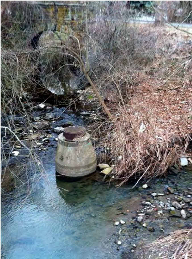
JMT01 - Sanitary sewer manhole in Lick Run's channel at confluence of Jefferson Memorial Tributary just downstream of Wilson Rd bridge.
