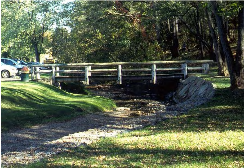
CRB06 – The Clifton Rd branch of Piney Fork at Simmon's Park. Much of the stream bank is modified within the park and the stream is detached from the floodplain.
