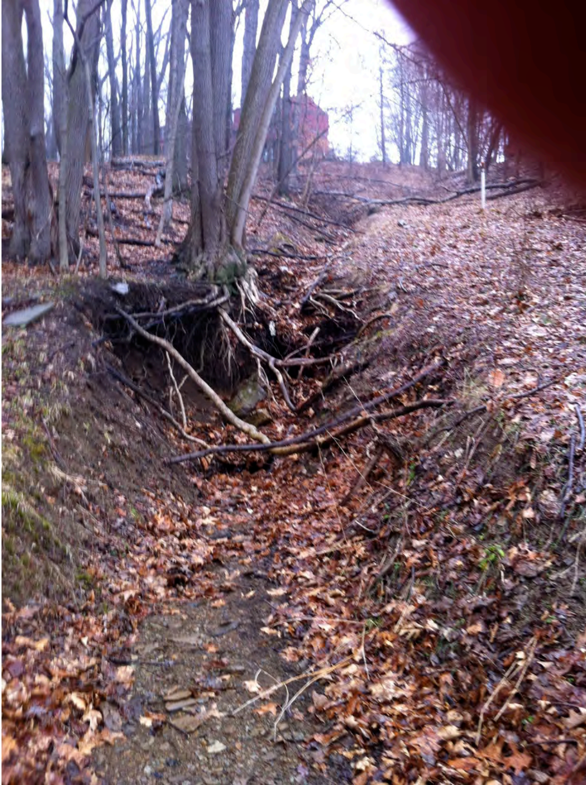
SH10 & SH15 – Inadequate stormwater controls have created deeply incised, eroding stormwater drainage channels from an apartment complex on Shelley Dr.
