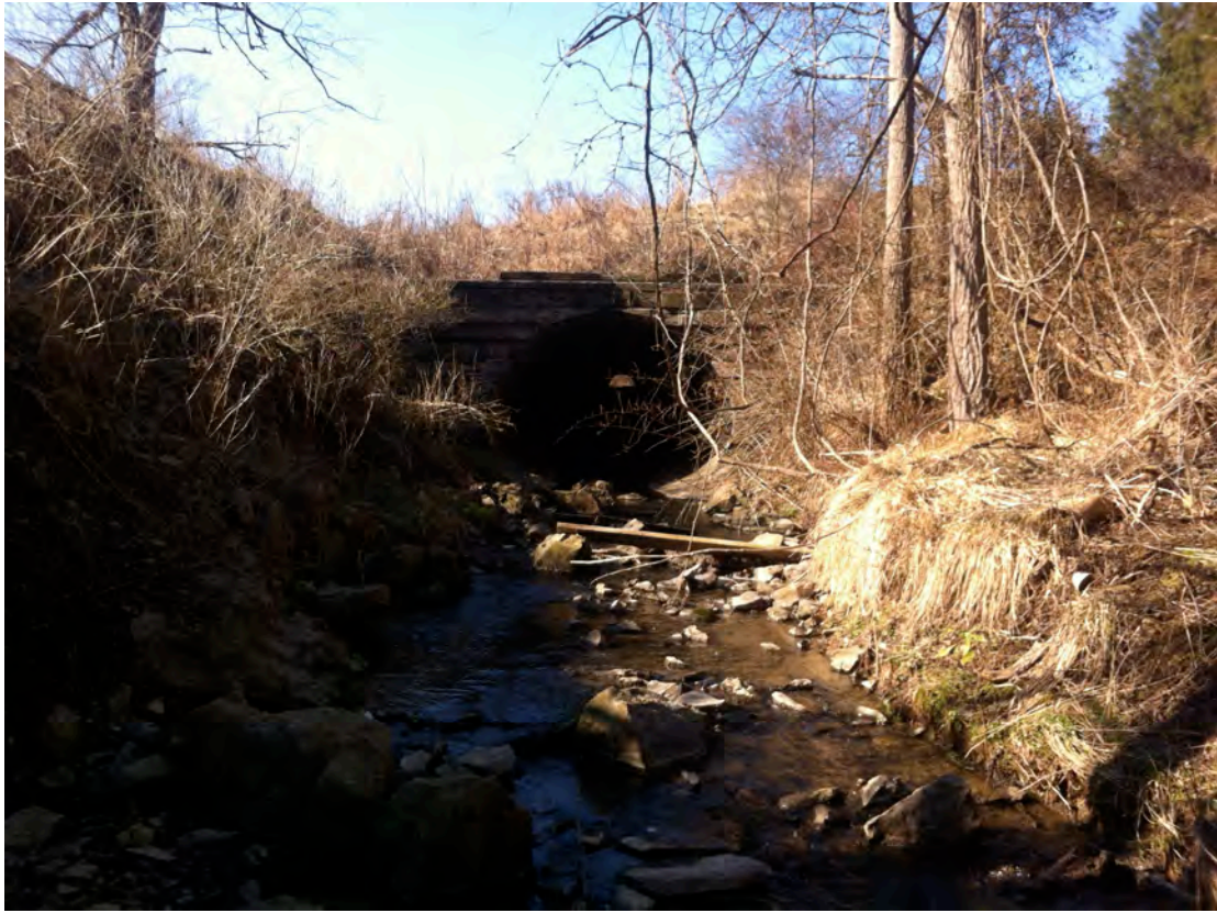
SH40 – Sleepy Hollow Run is culverted for approximately 400 ft at the tennis club along Sleepy Hollow Rd. There is a debris jam that is blocking about \frac{1}{4} of the entrance to the culvert and causing pooling behind it. Sleepy Hollow Run is seen exiting the culvert.
