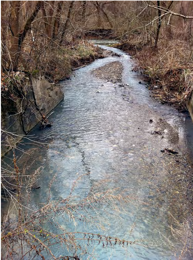
BR02 – Beam Run below Peters Creek Rd to Peters Creek. The culvert carrying Beam Run under Peters Creek Road is eroding and appears to be too small for the flow it carries. The stream channel is eroded upstream of the culvert and concrete debris in the channel is obstructing flow. This stream crossing is in need of replacement.
