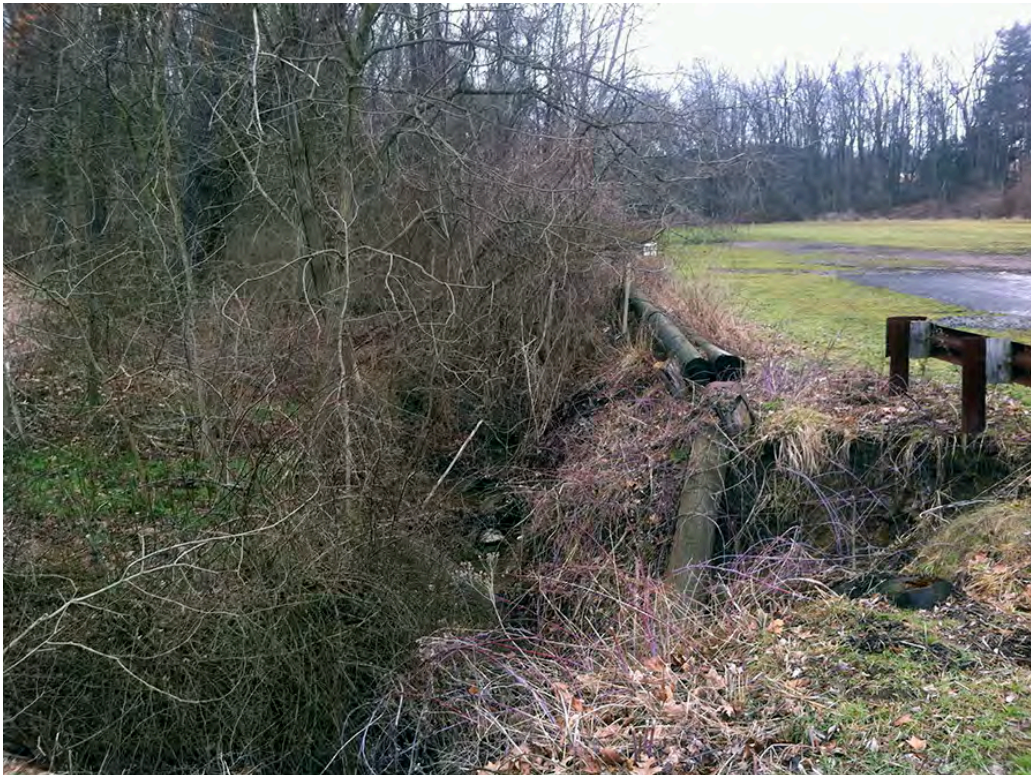
CRT29 – A fairly typical view of the East Branch Tributary and surrounding floodplain north of Hundred Acre Rd. The floodplain is choked with invasive plants and vines and the stream banks are eroding.
