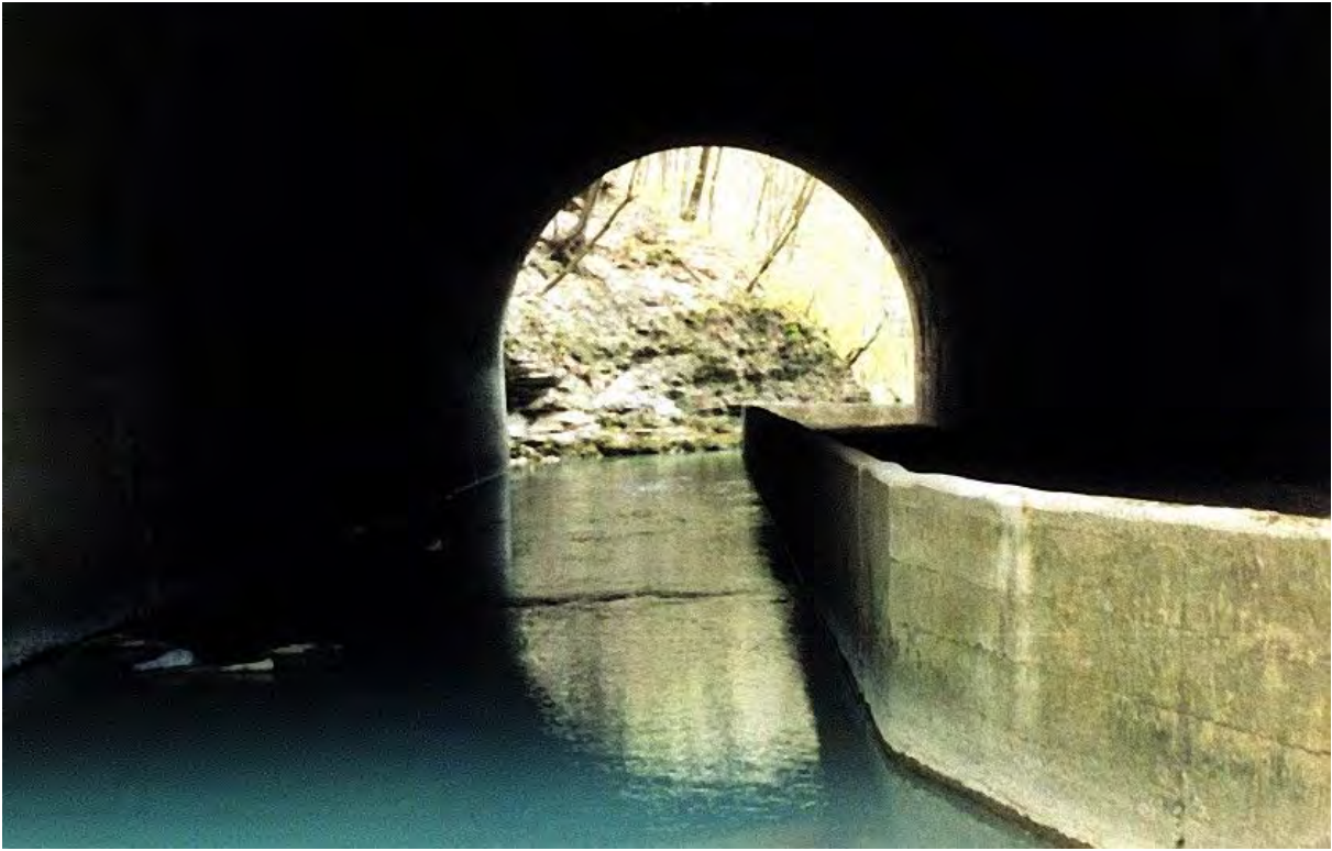
PCU029 – Peters Creek is channelized through a tunnel under the Allegheny Valley Railroad at the Allegheny and Washington County border. An undeveloped road runs along side the stream.
