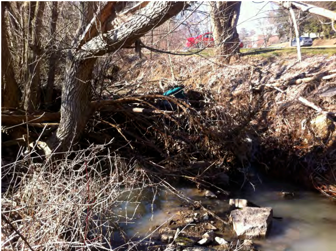
SH45 – A debris jam that is blocking the entire channel increases probability of flooding the adjacent parking lot and commercial buildings during significant rain events.
