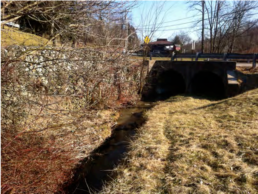
SH46 - One side of the double culvert under Sleepy Hollow Rd is clogged. Severe erosion is occurring on the left ascending bank below this culvert and on the right ascending bank above the culvert. A large section of gabioned riprap is being used to protect the bank above the culvert from eroding.
