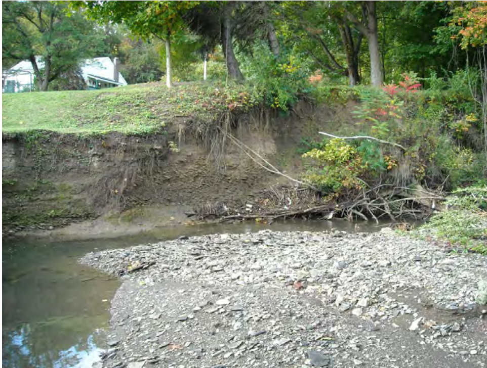
LW07 – Severe outer bank erosion and inner bank deposition along a tight S-bend near the Mon-Fayette Expressway Rt51 entrance ramp. Stream bank erosion is a problem at numerous locations along the Rt51 portion of the stream due to large quantities of storm water entering Lewis Run from the large commercial district in Lewis Run's headwaters.
