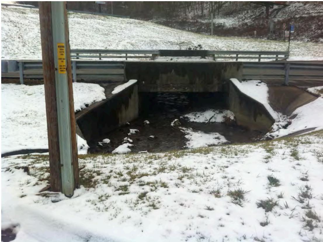
SCR04 - Scotia Run flows under Worthington Avenue. Sediment is being deposited along the right ascending wall of the culvert.
