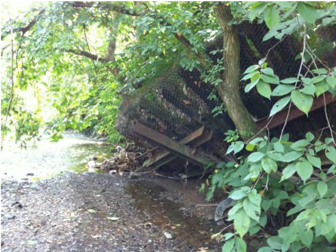
PCL43 – A collapsing retaining wall that appears to be part of a defunct railroad siding operation encroaches on Peters Creek’s left ascending bank across from the Large Park & Ride Lot. The Wheeling & Lake Erie tracks follow and encroach on Peters Creek’s southern shore from this point to the western portal of the Ravensburg Tunnel.
