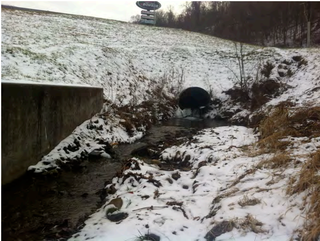
SCR05 – Scotia Run exits the culvert under Bowser Auto and storm water enters Scotia Run from the right ascending bank. The stream is culverted for approximately 700 feet under Bowser Auto's building and lot and then immediately flows under Worthington Avenue.
