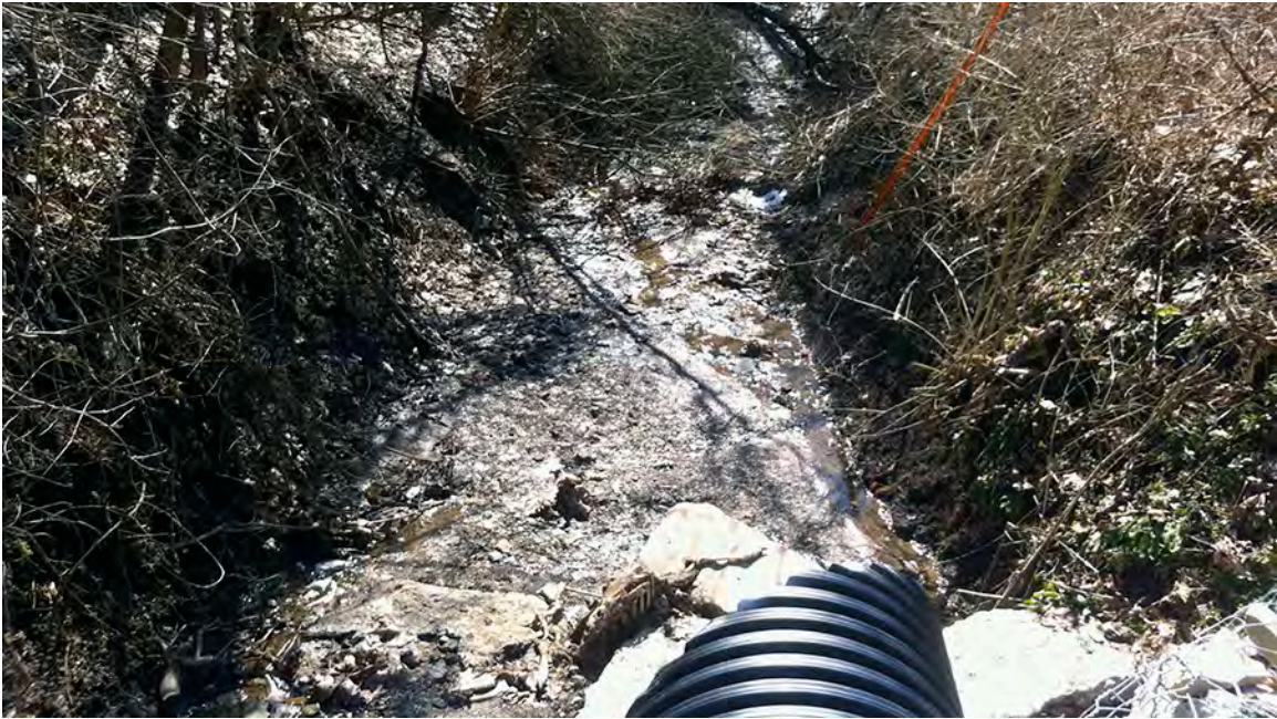
BR61 – The culvert carrying the Wakefield Road Tributary under Wakefield Road is not adequately sized. Severe erosion occurs both upstream and downstream of the crossing. The 002025 tributary to Beam Run flows within an enclosed channel for its entire length. Its confluence with Beam Run occurs in the culvert as the headwaters of Beam Run are piped under Beam Run Road. Beam Run then emerges from the culvert just downstream of the junction of Beam Run Road and Wakefield Road.
