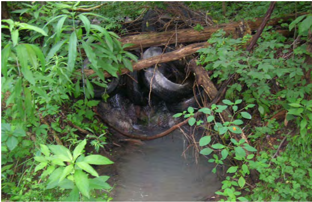
PF65 – An abandoned mine discharge enters Piney Fork just upstream of the Sebolt Rd discharge. This discharge appears to be culverted under Cardox Rd. A debris jam of tires and other assorted garbage has formed at the streams confluence with Piney Fork. Very little indication of AMD was found along Piney Fork upstream of this discharge.
