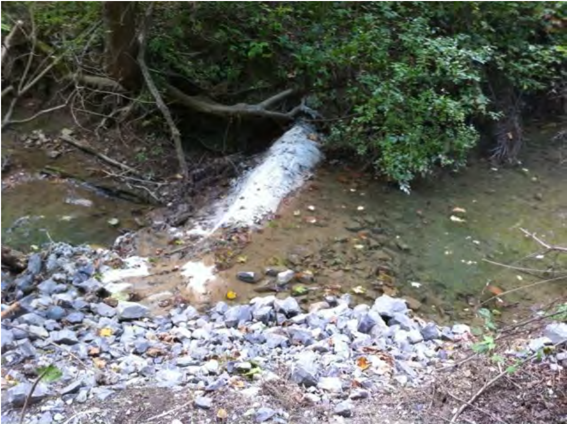
BR38 – Pipe crossing of Beam Run creates a plunge pool and totally obstructs the stream channel creating a fish barrier and erosion downstream.
