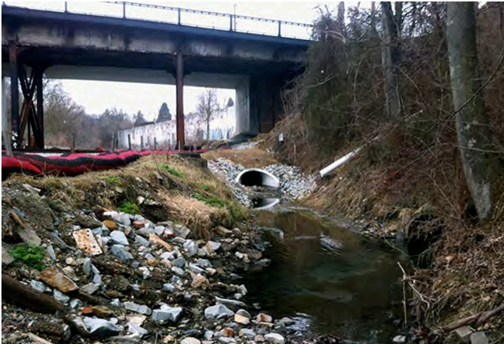
JMT20 – Numerous discharges of stormwater from the commercial district along Terence Drive enter Jefferson Memorial Tributary just downstream of the Curry Hollow Rd overpass. There are also several discharges upstream of the bridge to the headwaters near Whitehall Tunnel. Many of these discharges are choked with algae as is the stream channel itself.
