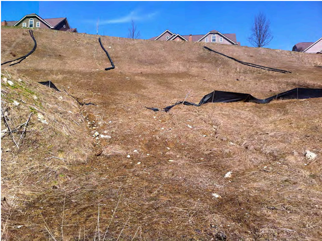
BR70 – An unstable slope along Beam Run Road at the Jefferson Pointe residential development creates a number of public and private problems. Inadequate drainage and excess stormwater are most like contributors to the problem.
