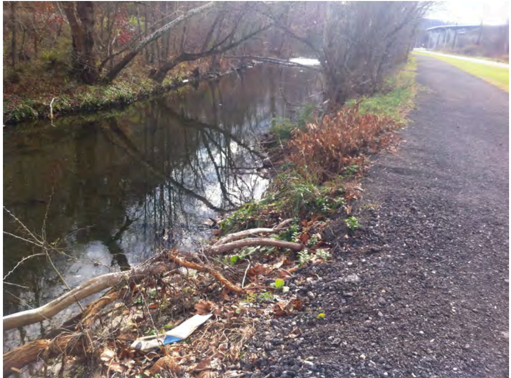
PCL33 – Severe erosion along Peters Creek’s right ascending bank downstream of the Large Park & Ride Lot is undercutting the Montour Trail and uprooting trees.
