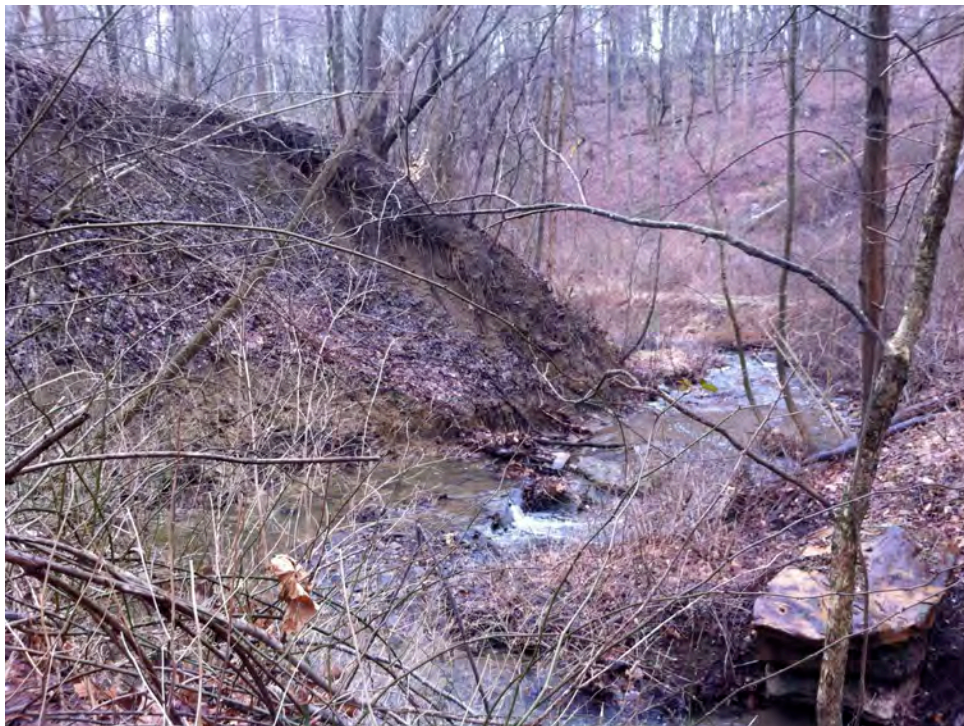
SH12 - Severely eroding right ascending bank through what appears to be some type of fill.
