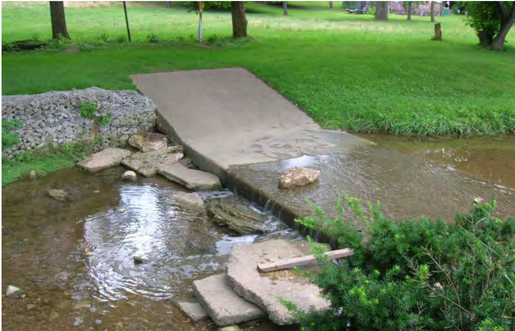
PF07 – A concrete access ramp across the Clifton Road branch of Piney Fork at Simmon's Park obstructs the stream channel, creates a fish barrier in the stream and accelerates erosion downstream of the structure. The left ascending bank of Piney Fork is gabion riprapped downstream of the ramp.
