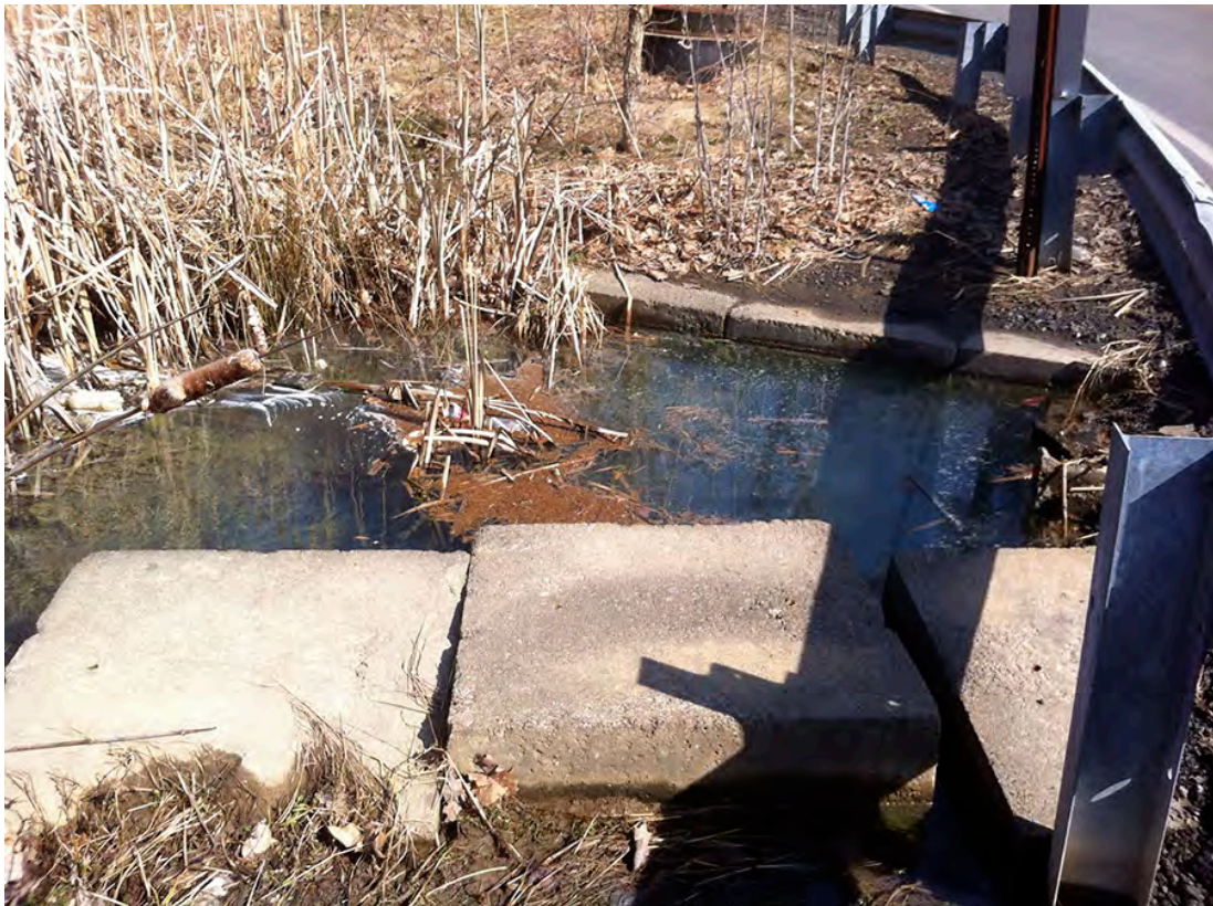
BR49 – The culvert carrying Beam Run under Chamberlain Road is either too small or clogged with debris.
