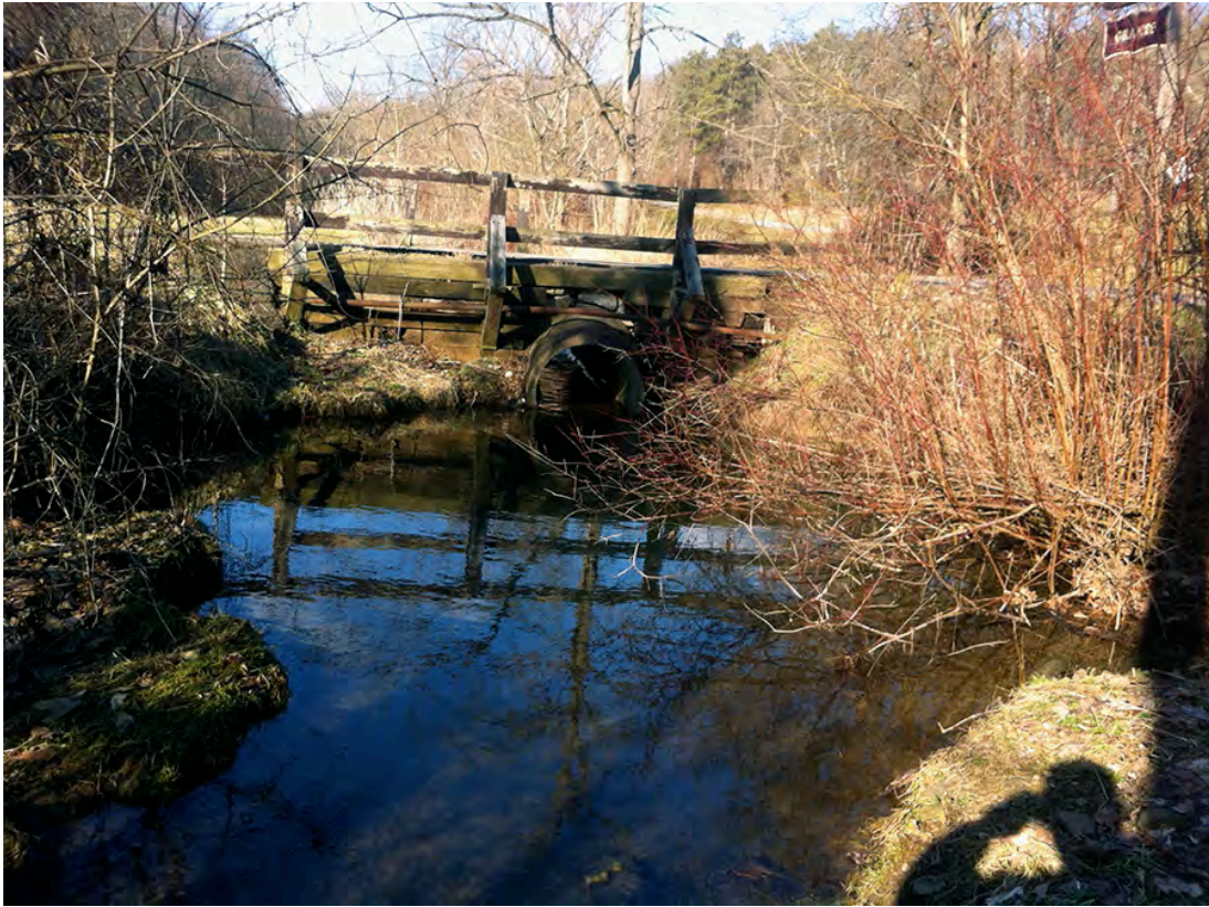
CRT03 - Improperly sized culvert at the access road to Grant Grove within the East Branch of Catfish Run is causing severe bank erosion both upstream and downstream of the culvert. This is a common problem at a number of crossings of the East Branch.
