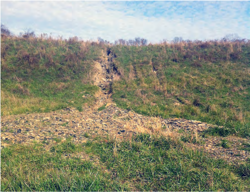
PCLT03 – An erosion gully has developed at the western end of the Rochez #2 site. Otherwise, reclamation at the site appears to be going well. The mining did not seem to affect water quality within the Rt885 tributary to a great degree. It appears that some regrading and planting at the site occurred in 2012/2013 to resolve erosion issues. This entire valley would most likely be altered dramatically if the section of the Mon-Fayette Expressway from Jefferson Hills to Pittsburgh/Monroeville is completed.
