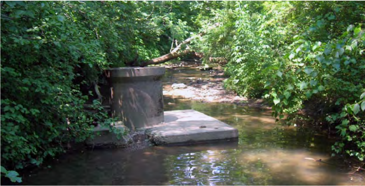
At a number of locations along the Corrigan Rd portion of the main stem of Catfish Run large concrete debris of various forms is found within the channel of Catfish Run. This particular culvert and headwall fragment is located near the off-leash dog park.
