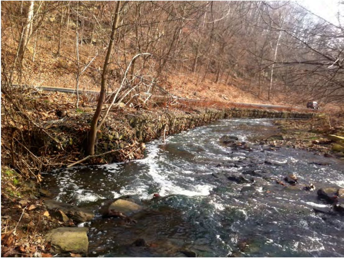
PF11 – Gabioned riprap creates right ascending bank of Piney Fork with Piney Fork Rd nearby. Japanese Knotweed infests the entire length of the gabioned riprap. Bank erosion at the head of the riprap.
