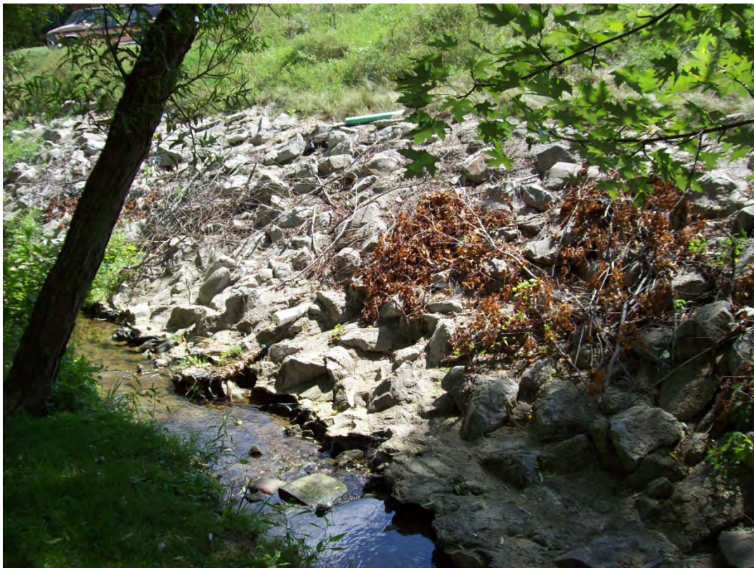
CRC28 – Grouted riprap applied to the eroding left ascending bank of the Clifton Rd Branch of Piney Fork just upstream of the Havengate Street crossing of the stream.
