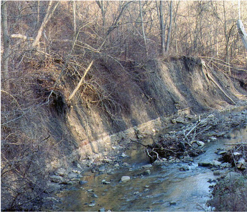
LW24 – Severe right ascending bank erosion along Lewis Run downstream of the Blue Flame Restaurant.
