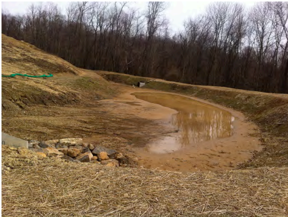
A stormwater detention basin within the Washington Square residential development along Gill Hall Road, Waterman Road and the Wheeling & Lake Erie Railroad tracks in Jefferson Hills. The lower reach of Lick Run forms the border between Jefferson Hills and South Park Township. Ordinances requiring effective stormwater control are absolutely essential in this rapidly developing sub-watershed. Retaining green infrastructure and stormwater on site and implementation of best management stormwater practices are most likely necessary to be protective of water quality in Lick Run.
