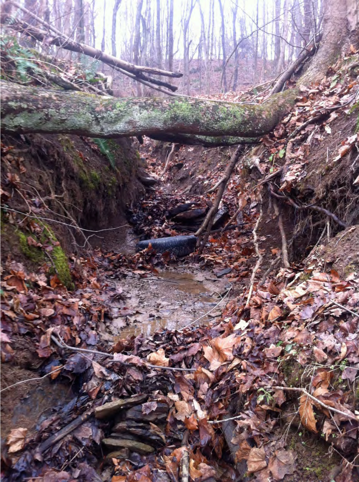
PF08 – A deeply incised tributary that conveys excessive quantities of stormwater from the old Montour Railroad right of way through Piney Fork’s left ascending floodplain to the stream. This creates severe bank erosion downstream. Heavy off-road activity along the right of way and lack of understory vegetation within the floodplain has exacerbated the problem.
