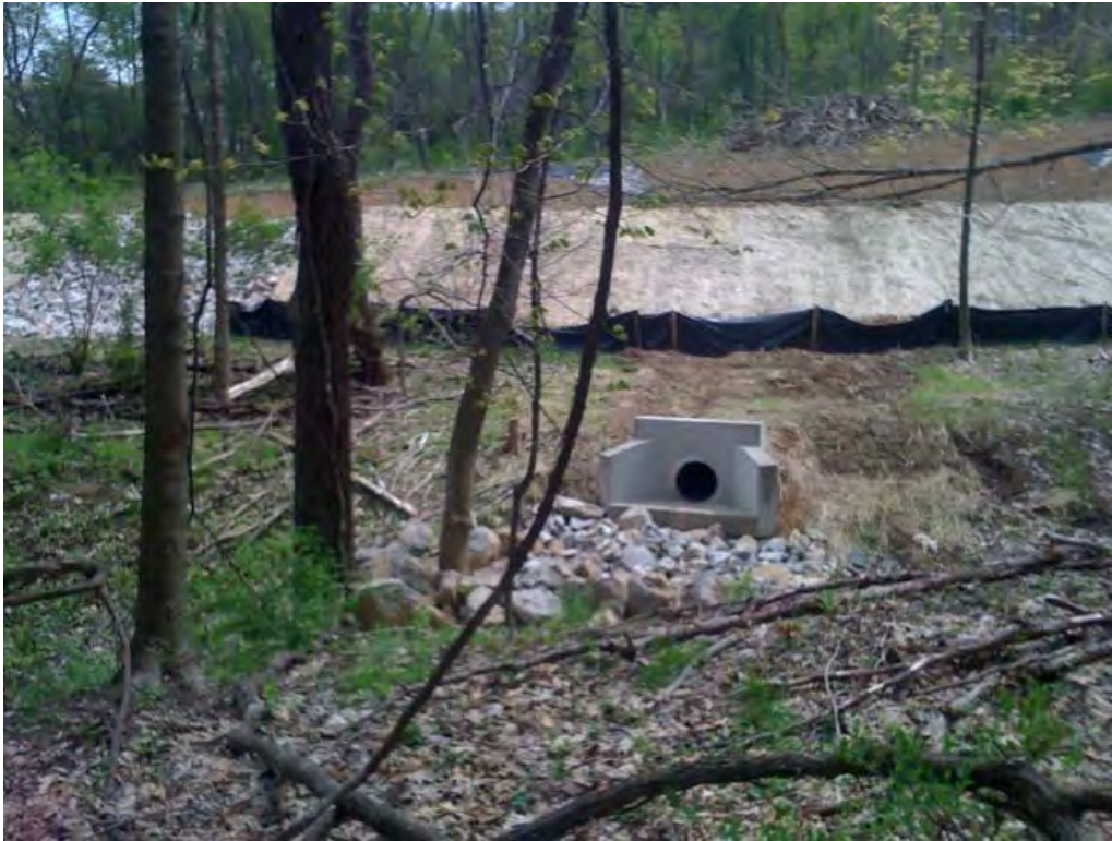
PF52 – A new stormwater detention basin off of Brownsville Road Ext discharges to a small tributary that is culverted under the Montour Trail and enters Piney fork's left ascending bank across from Georges Supply.
