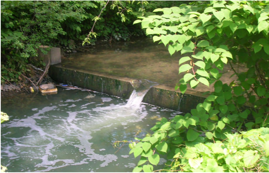
LR33 - A berm dam across Lick Run's channel creates a fish barrier within the stream.
