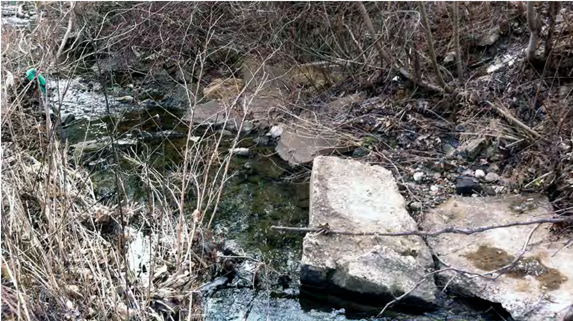
JMT05 – Concrete rubble is obstructing the channel of the Jefferson Memorial Tributary. Remnants of a concrete structure forms a low dam across the stream channel and creates a fish barrier at this location.
