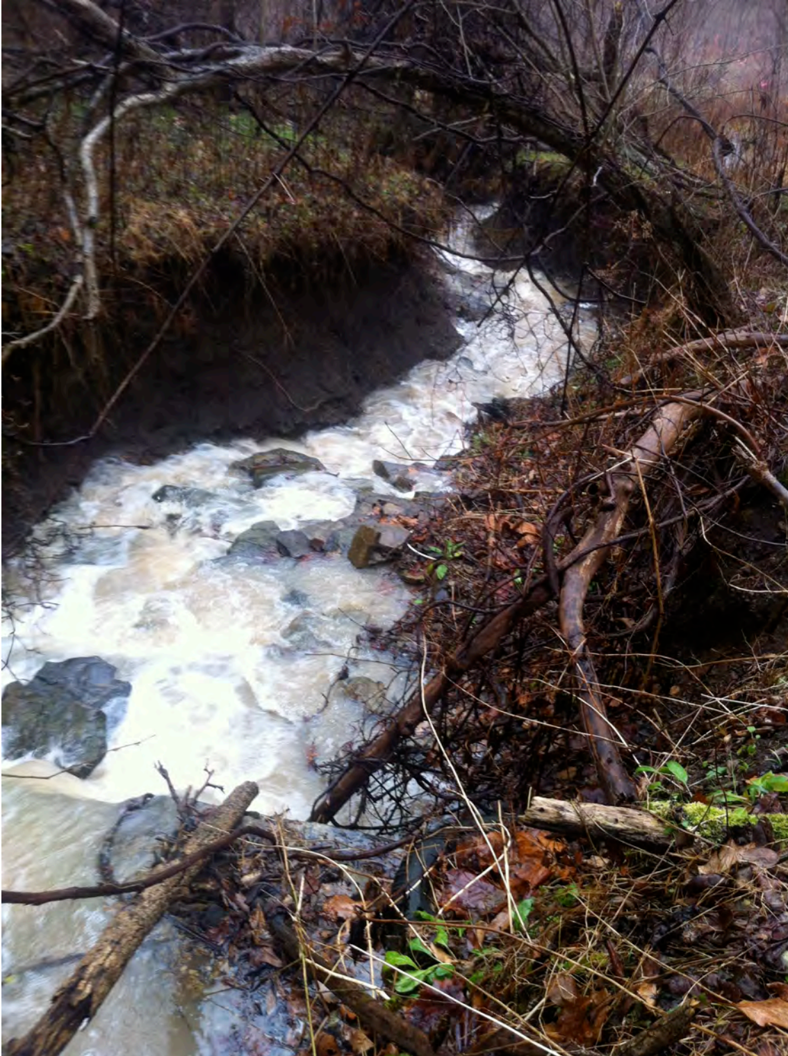
PCU020 – A deeply incised stormwater channel created by runoff from a Mon-Fayette Expressway stormwater detention basin at PCU019.
