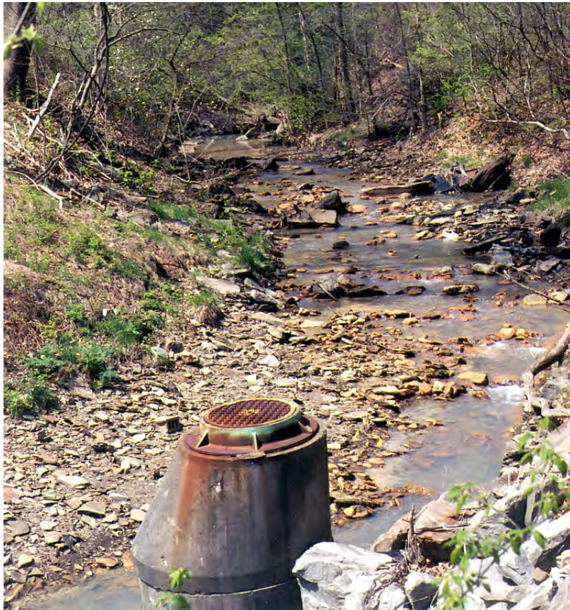
LW20 – A sanitary sewer manhole downstream of Lewis Run’s confluence with the Jefferson Hospital Tributary is within the streams channel. The sewer contents combine with the stream during high water events.
