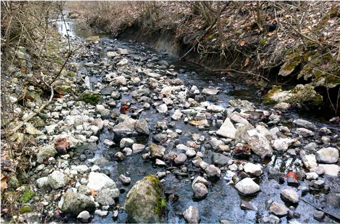
JMT17 - Jefferson Memorial Tributary channel clogged with concrete and other assorted rubble just downstream of its exit from a 700 foot culvert under a commercial district along Old Curry Hollow Road.
