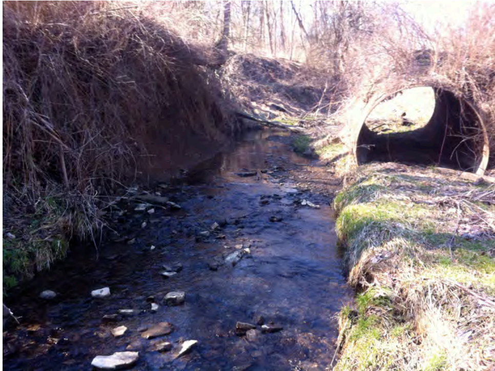
SH35 - Section of Sleepy Hollow Run near county park border has a severely eroding left ascending bank. Old piece of culvert along stream channel creates problems of its own.
