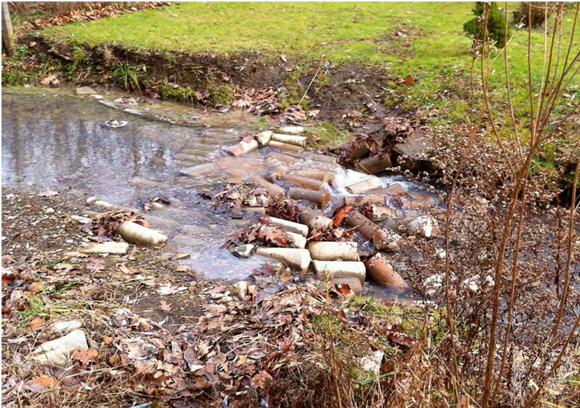
MRT08 - Homeowner attempt at a stream crossing of Mineral Run obstructs the stream channel, creates erosion issues, is eroding itself and should be removed.
