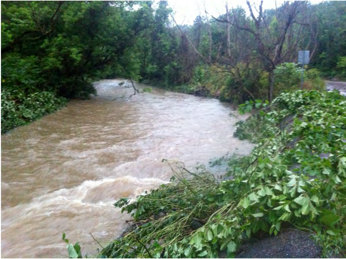
PCU021 – Peters Creek’s eroding right ascending bank consists of approximately 150 feet of gabioned rip-rap along Piney Fork Road in South Park Township just downstream of the Piney Fork confluence. The purpose of the rip-rap is to prevent the stream from undercutting the road. The stream is undercutting the rip-rap as the erosive force of the stream migrates upstream. Eddy currents downstream of the project are also eroding the right ascending bank downstream of the rip-rap. Asphalt was applied from the road to the rip-rap along this section. The purpose of this is unknown and most likely counterproductive. Japanese Knotweed has taken hold along this section of stream bank.
