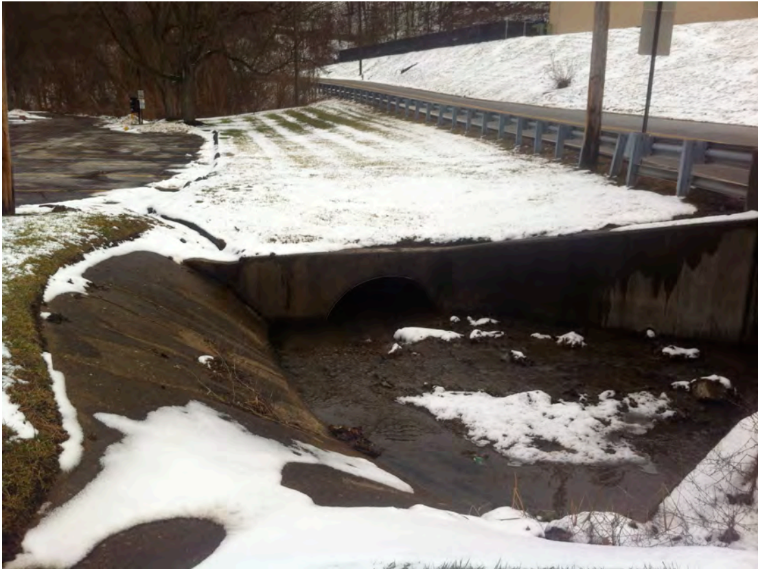
SCR03 - Scotia Run flows under Worthington Avenue and then is immediately culverted again for approximately 150 feet between Lesker's parking lot and Worthington Avenue. It then flows freely for a couple of hundred feet before being culverted again.
