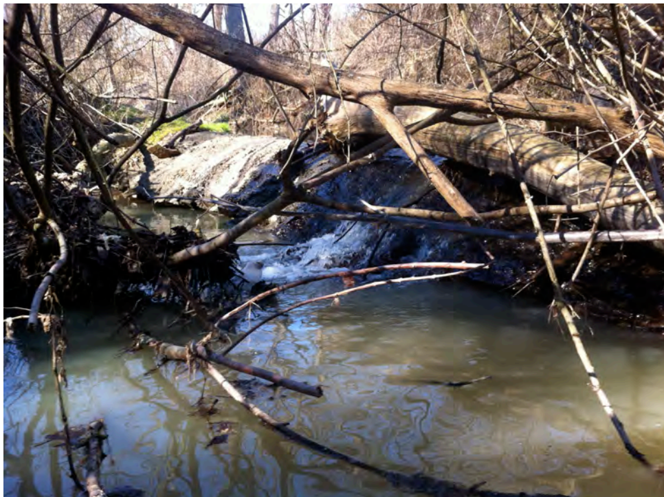
SH37 – A structure crossing Sleepy Hollow Run is being protected and reinforced by concrete. This structure creates a fish barrier and bank erosion at the site.
