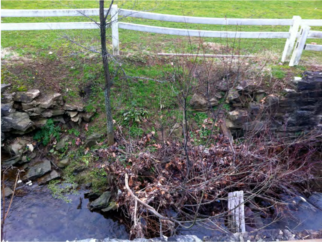
CR28 - Severe bank erosion along the channelized portion of Catfish Run at the fairgrounds has eroded away part of the retaining wall.
