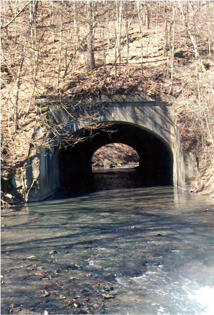
LR05 – Lick Run flows under the Wheeling & Lake Erie Railroad. A sewer manhole can be seen within the stream channel just upstream of the bridge.
