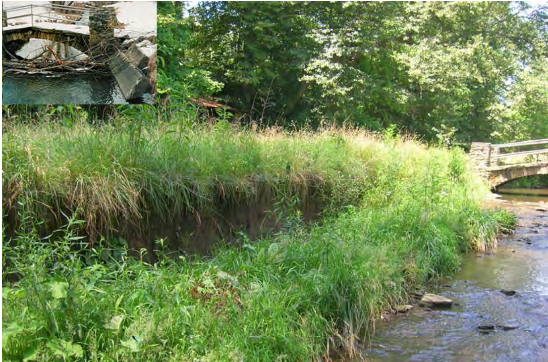
CR35 - Bank erosion downstream of a historically significant pedestrian bridge crossing Catfish Run between the soccer fields and Corrigan Dr. Catfish Run is effectively channelized along Corrigan Drive from the circle to the fairgrounds and is not permitted to meander as a stream normally would. Stream meanders dissipate energy during severe rain events and mitigate erosion. Inset shows bank erosion just upstream of the bridge.
