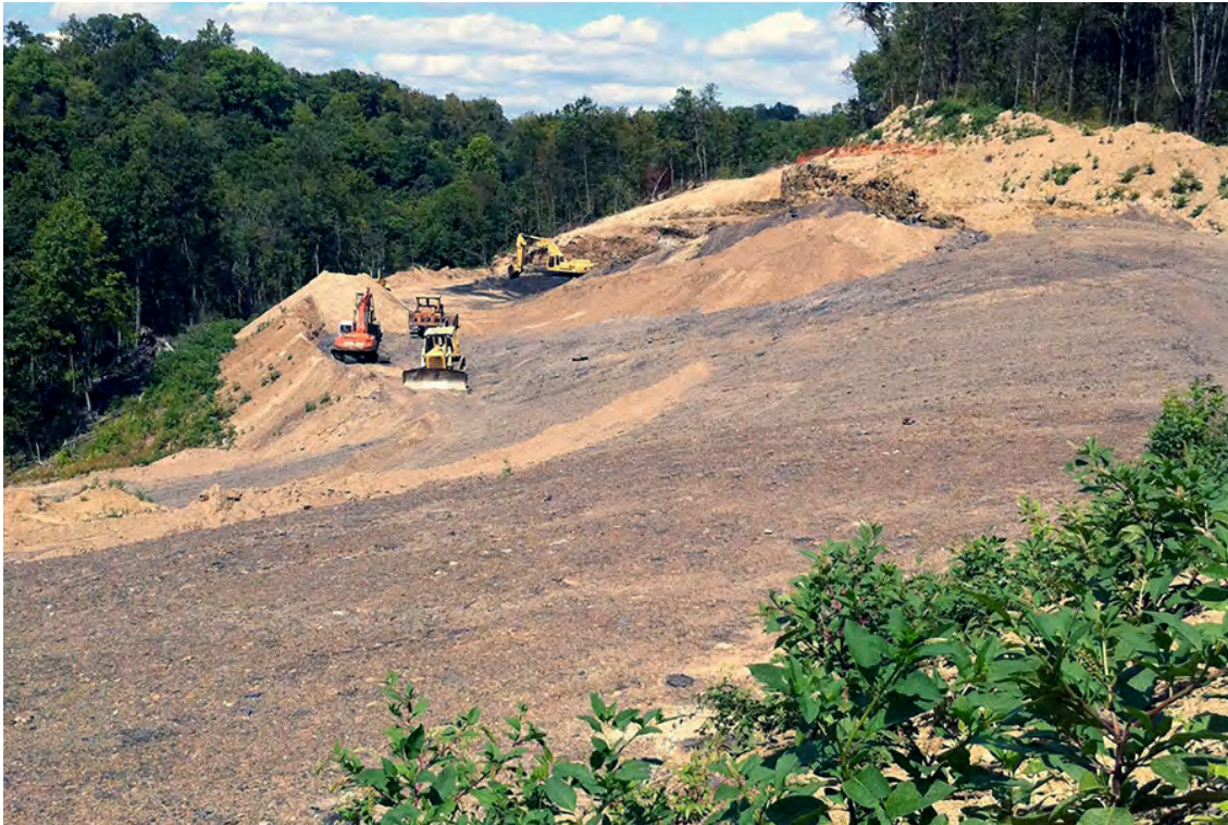
BR40 – Zora Mine Reclamation Project while in operation during 2010. Tributary 002034 to Beam Run flows in the bottom of the wooded section of the photo. This reclamation project was associated with Priority 3 abandoned mine lands (AML) and was financed via a Government Financed Construction Contract.
