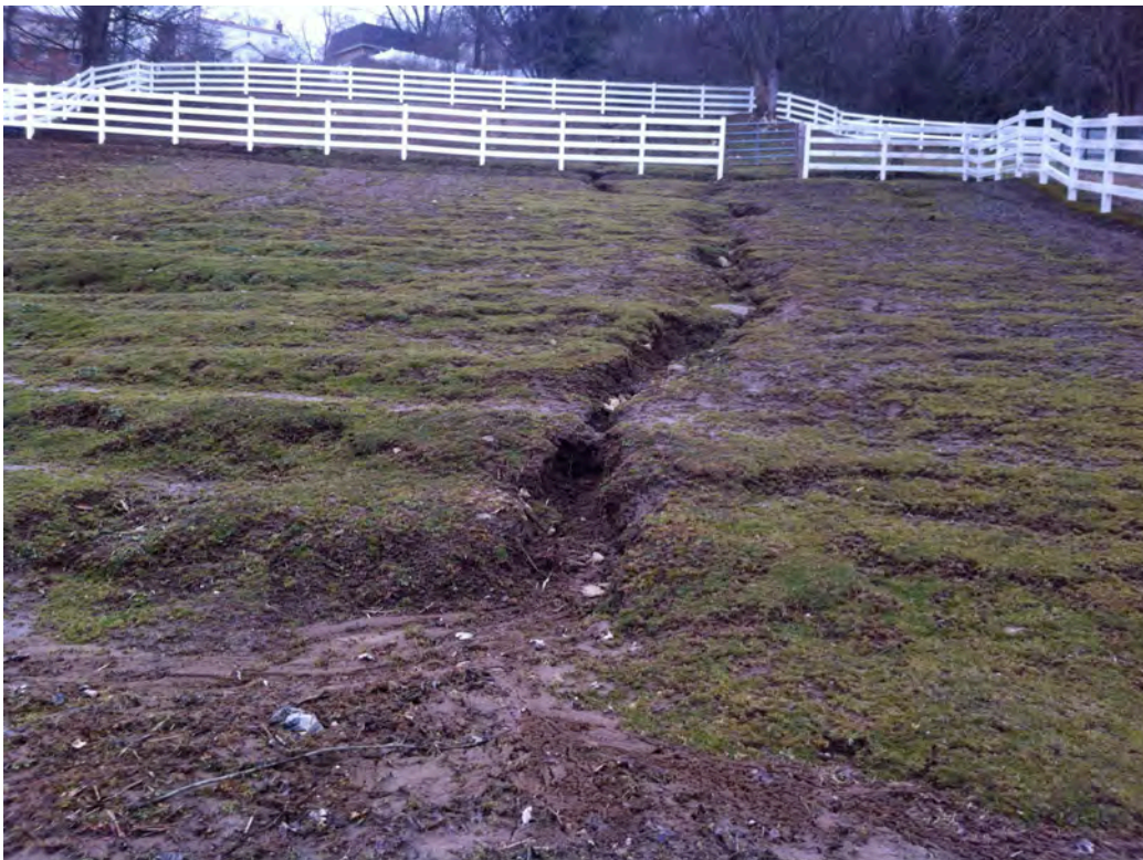
SH49 - Erosion in high use area of horse farm pasture along Stoltz Rd sends sediments and pollution to the creek.
