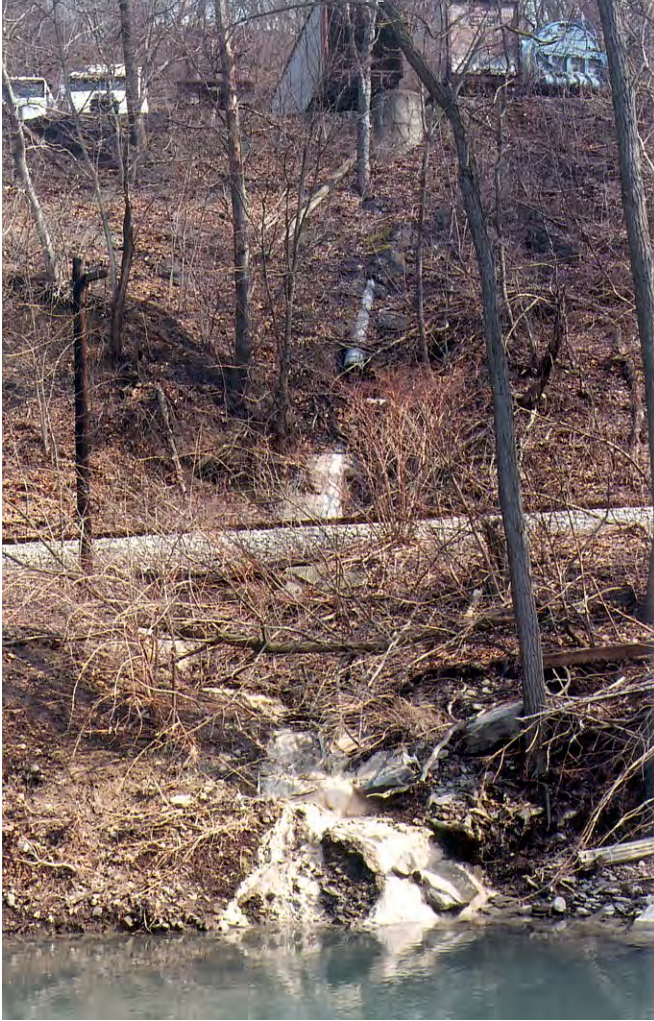
PCL38 – An alkaline discharge with pH of 11.5 enters Peters Creek’s left ascending bank across from the Large Park & Ride Lot. The discharge is culverted under a deck hockey facility off of Worthington Avenue and under the Wheeling & Lake Erie Railroad tracks prior to entry into Peters Creek.
