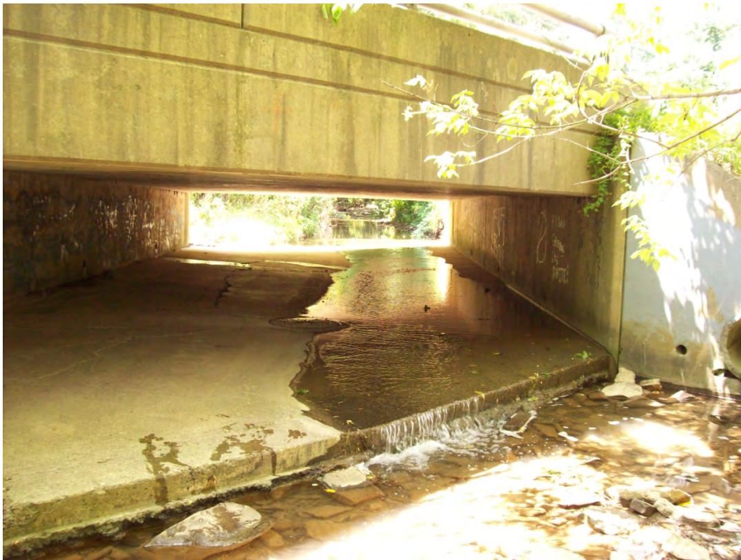
CRB16 – The Irishtown bridge over the Clifton Road branch of Piney Fork obstructs the stream channel and creates a fish impasse.
