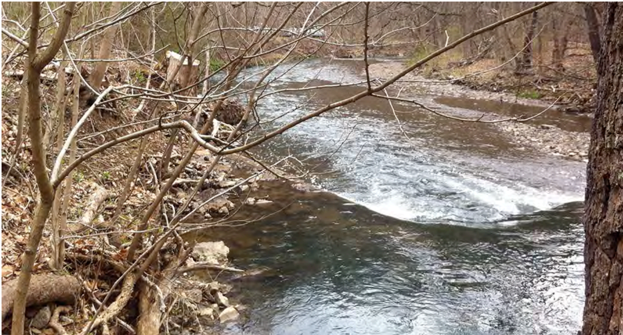
PCM42 – A log vane structure helps to direct the energy of the streams flow toward the center of the channel and away from the eroding bank along the road at Jefferson Hills Phase 2 Natural Stream Channel Design Restoration Project along Peters Creek Rd. A rootwad just downstream provides added protection to the stream bank.
