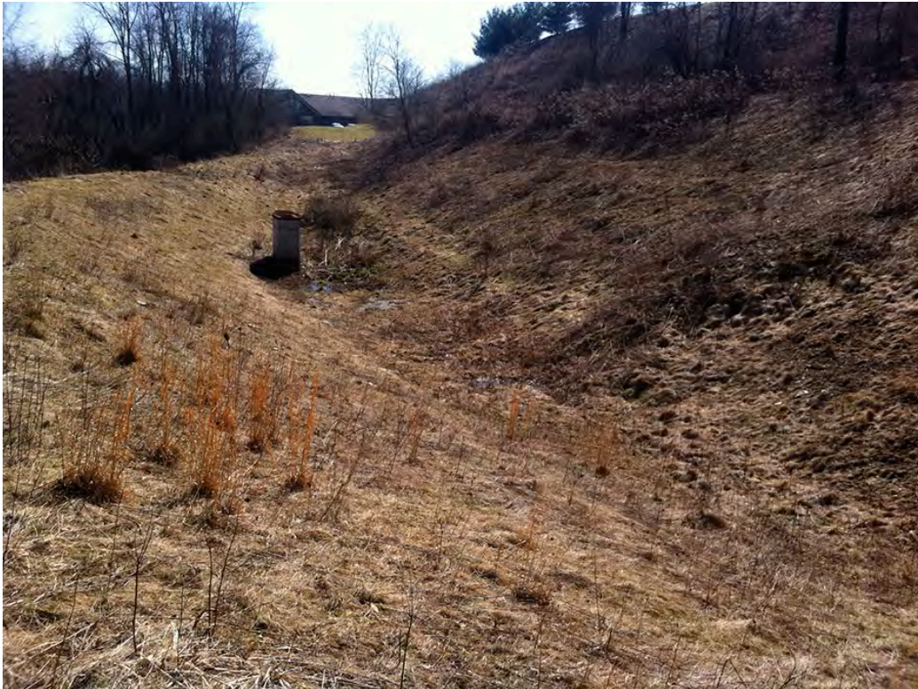
BR69 – Stormwater detention basin for the Jefferson Pointe residential townhome development of of Gill Hall Road.
