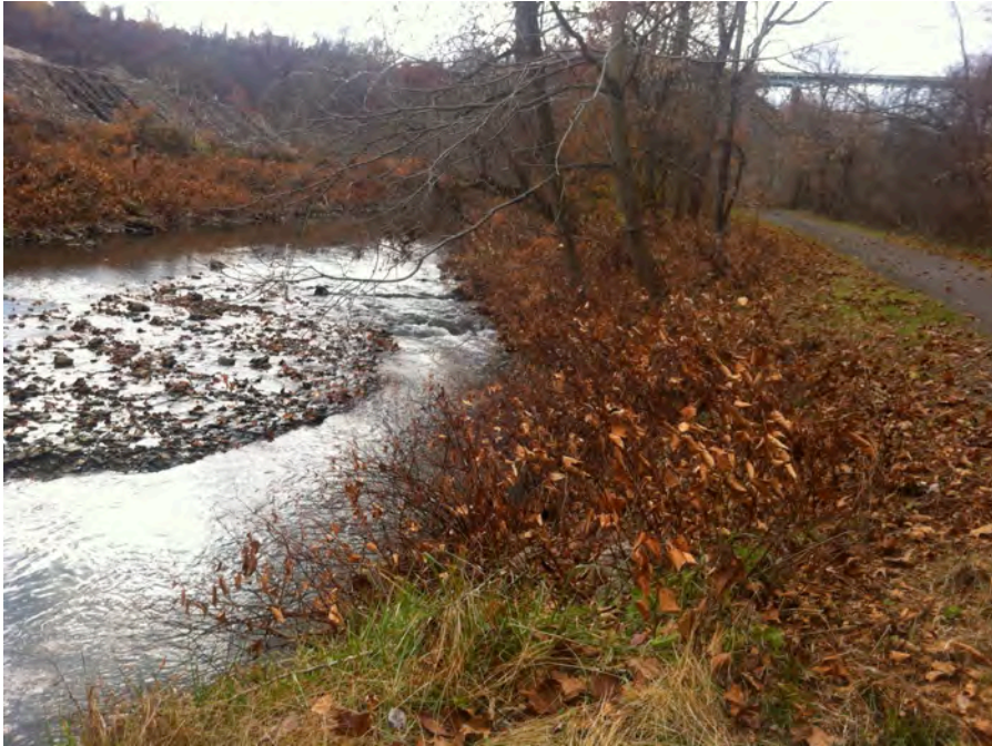
PCL14 - Large sediment build up in middle of channel alters flow pattern of Peters Creek downstream of Ravensburg Bridge crossing of the stream. The right ascending bank is experiencing increased erosion that is beginning to impact the Montour Trail. Knotweed covered banks downstream do little to stabilize the riparian zone.
