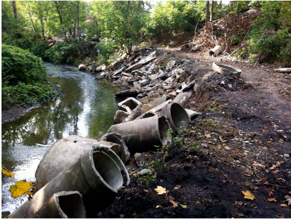
PF26 – The beginnings of a stream bank stabilization project along Piney Fork’s right ascending bank along the Montour Trail east of Triphammer Rd. This project appears to be as much about waste disposal as it does about streambank stabilization.
