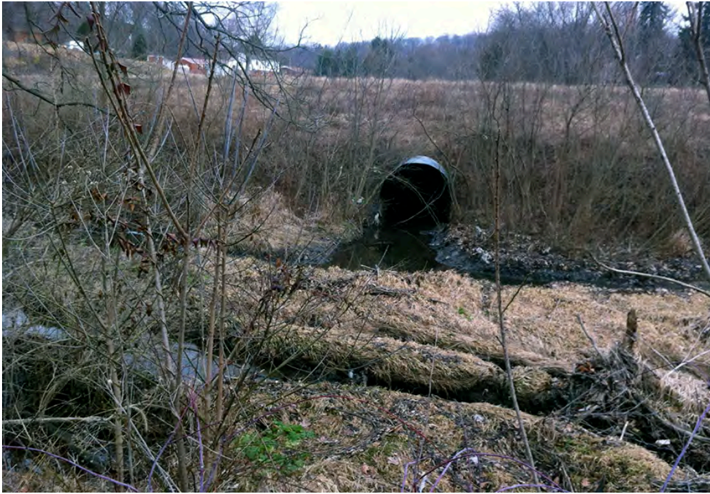
JMT11 – A culverted stream that accepts stormwater from a detention pond servicing Pleasant Hills residential neighborhoods west of West Bruceton Rd enters Jefferson Memorial Tributary's right ascending bank. The tributary channel is braided and eroded at this location. The stream appears to have been culverted and the area filled and graded in anticipation of additional commercial development along an extended Terence Drive.
