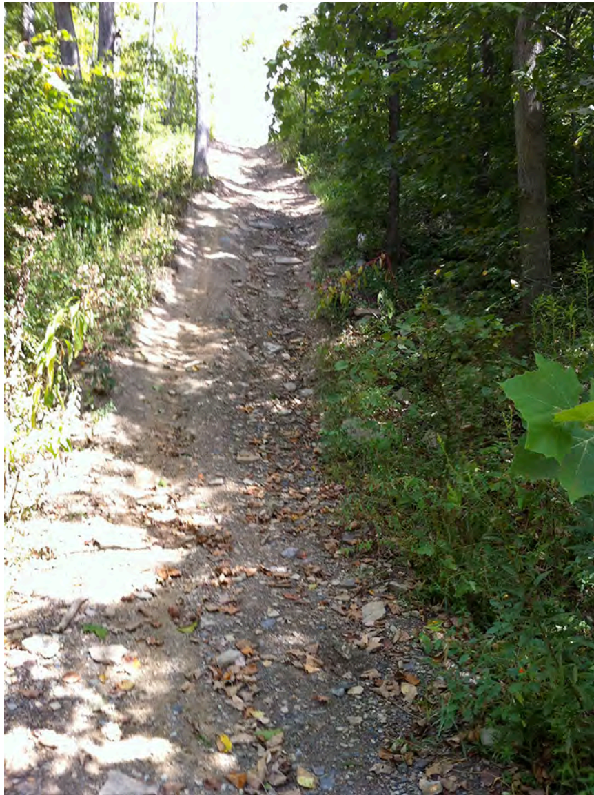
BR25 – Off-road trails ascending Beam Run’s steep valley slopes create stormwater runoff channels that alter drainage patterns, create excess erosion and add to Beam Runs siltation load.
