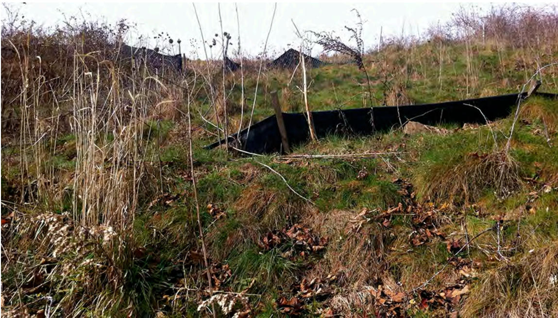
MRT06 – Unstable and eroding slope above Mineral Run's left ascending bank that was recently re-graded as part of the Hunters Field residential development along West Bruceton Rd in Jefferson Hills.
