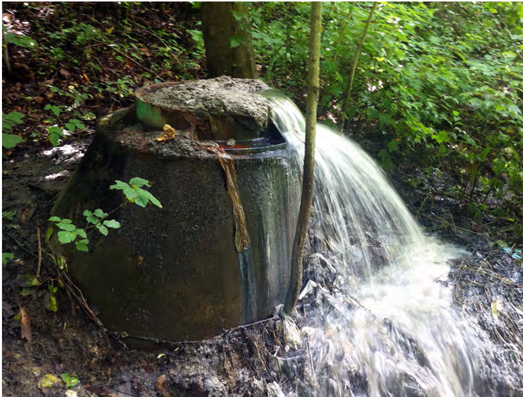
JHT04 – This overflowing sanitary sewer line along the Jefferson Hospital Tributary was dumping its contents directly into the tributary. Sanitary sewer lines often follow tributary valleys and in Jefferson Hills many are in fairly remote locations like this one. They also often end up within the stream channel due to the dynamic nature of streams. Malfunctioning sewers and those in stream channels contribute to the bacterial and nutrient load within Lewis Run.
