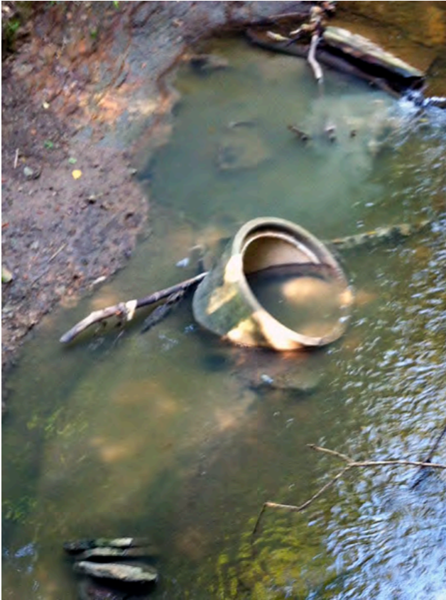
LR05 – Raw sewage enters Lick Run just upstream of the W&LE overpass as the result of a sanitary sewer manhole malfunction. Sewage infrastructure within the stream channel is often compromised by flooding and debris jams.
