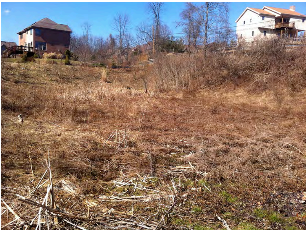
BR64 – Stormwater detention basin accepting stormwater from the Woods of Jefferson residential development along and off of Beam Run Road.
