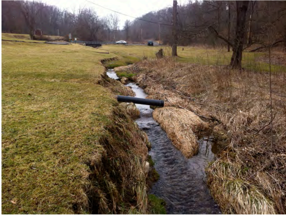
SH30 – Bank erosion and a floodplain detached from the stream along an approximately 400 ft reach within South Park County Park that has an inadequate riparian buffer. This section would benefit from a reforestation effort.
