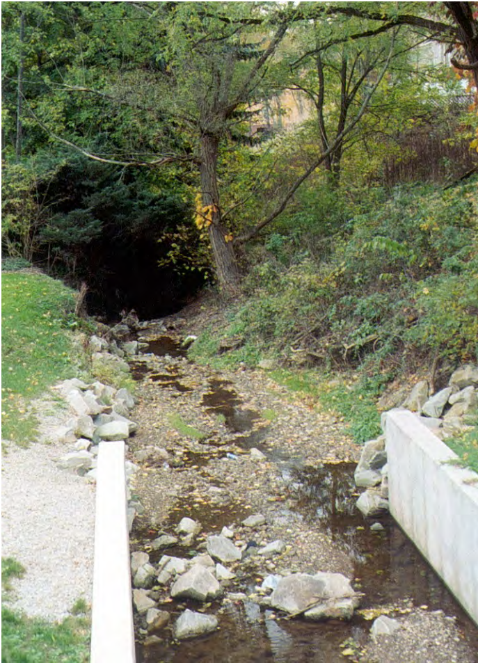
CRB28 – The Clifton Road branch of Piney Fork is channelized downstream of the culvert carrying Havengate Street over the stream. Severe erosion is occurring downstream of the channel and upstream of the culvert as well indicating that the culvert may be inadequately sized.
