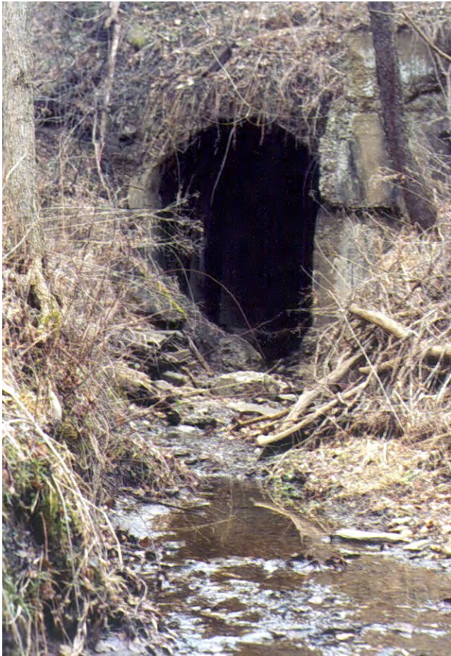
LR03 – A great deal of new development is taking place along the lower reaches of Lick Run. To the right is a view of another deeply incised and channelized tributary to Lick Run that accepts stormwater from the Patriot Pointe development along Gill Hall Road in Jefferson Hills. The tributary is seen exiting a culvert under the Wheeling & Lake Erie Railroad.
