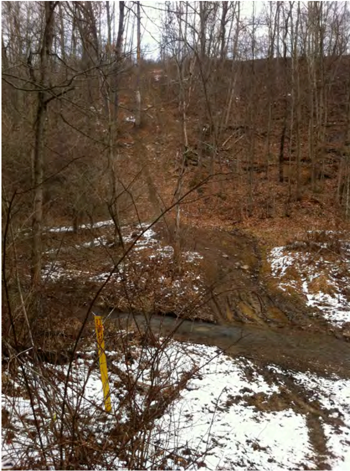
BR25 - Heavy off-road activity along a gas well access road has created a stormwater channel and increased stream sediment load. The road is no longer useable due to these severe erosion gullies.
