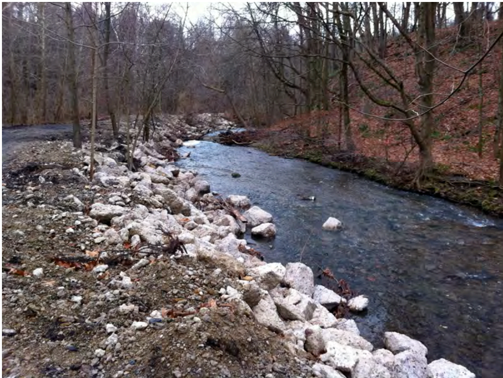
PF26 – Unsized rubble from a tunnel demolition project in Peters Township was thrown along approximately 800 feet of Piney Fork’s right ascending bank and at sites downstream. Little was done to protect trees along the bank and rubble ended up within the low flow stream channel and continues to slide into the channel during high water events. PA DEP Growing Greener Grants have been utilized successfully to implement Natural Stream Channel Design (NSCD) Projects along Peters Creek in Jefferson Hills. A stream stabilization project designed by an engineer trained in NSCD along this portion of Piney Fork would have maintained the natural integrity of the corridor and enhanced fish habitat along this stocked portion of Piney Fork while also achieving the necessary bank stabilization.
