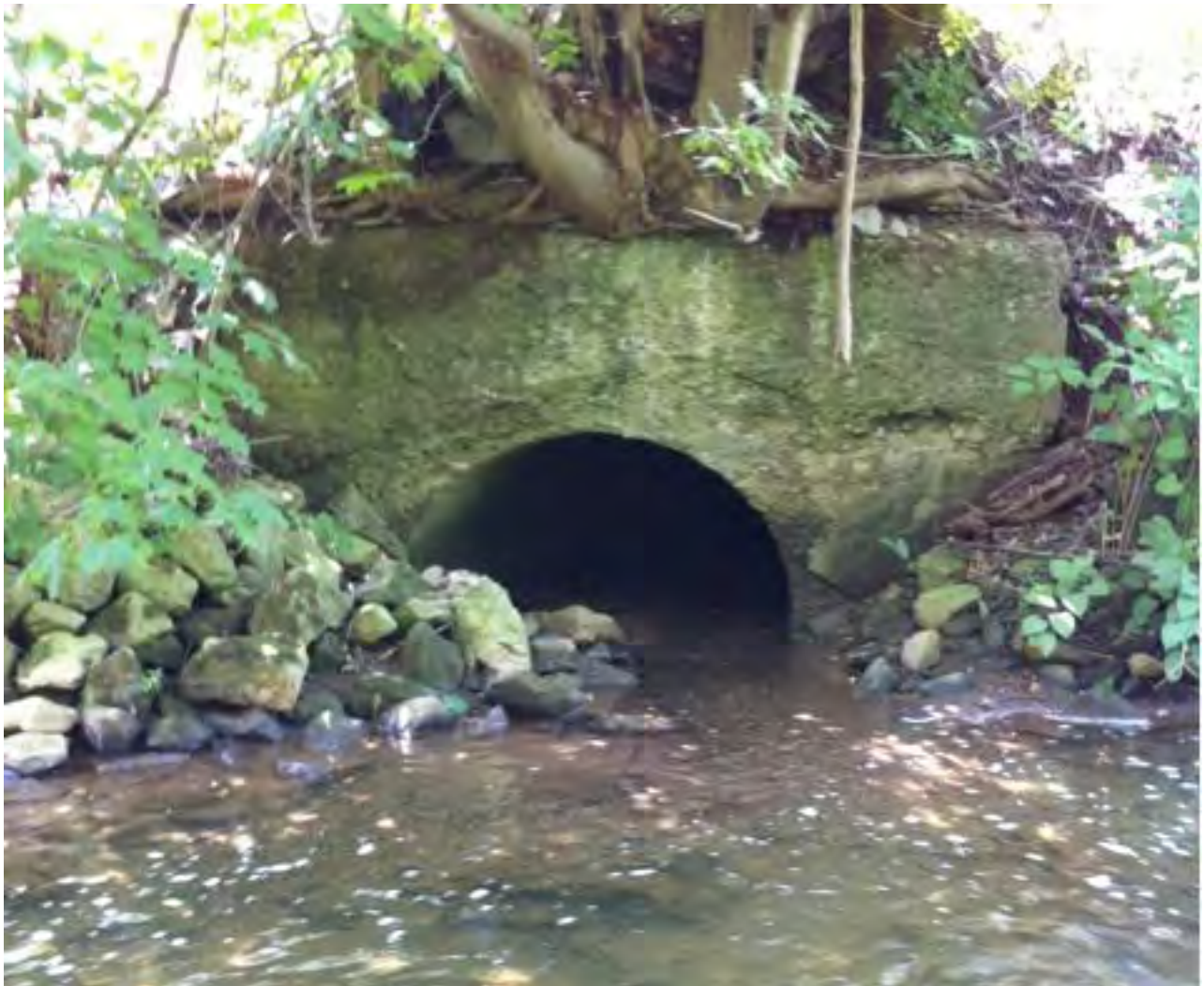
PCL41 – Scotia Run enters Peters Creek's left ascending bank after being culverted for approximately 250 feet under Kurt J. Lesker's back lot.
