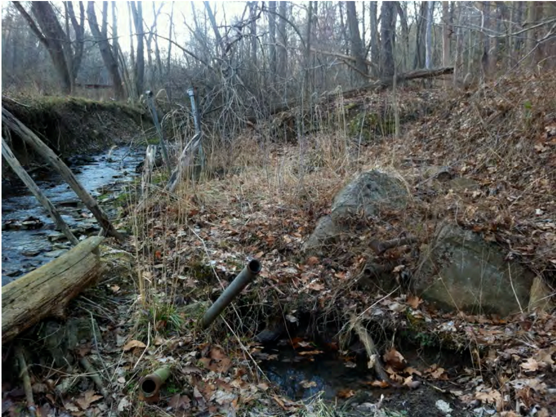
CRT16 - Remnants of an old concrete and metal structure along the right ascending bank of the East Branch of Catfish Run is creating bank erosion.
