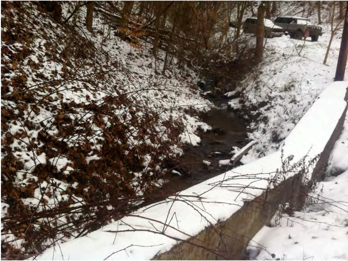
SCR15 – The tributary that drains the valley to the southeast of Scotia Run with headwaters near Ridge Rd and flowing along the commercial district along Century Dr is culverted under McGrew Rd and enters Scotia Run's left ascending bank.
