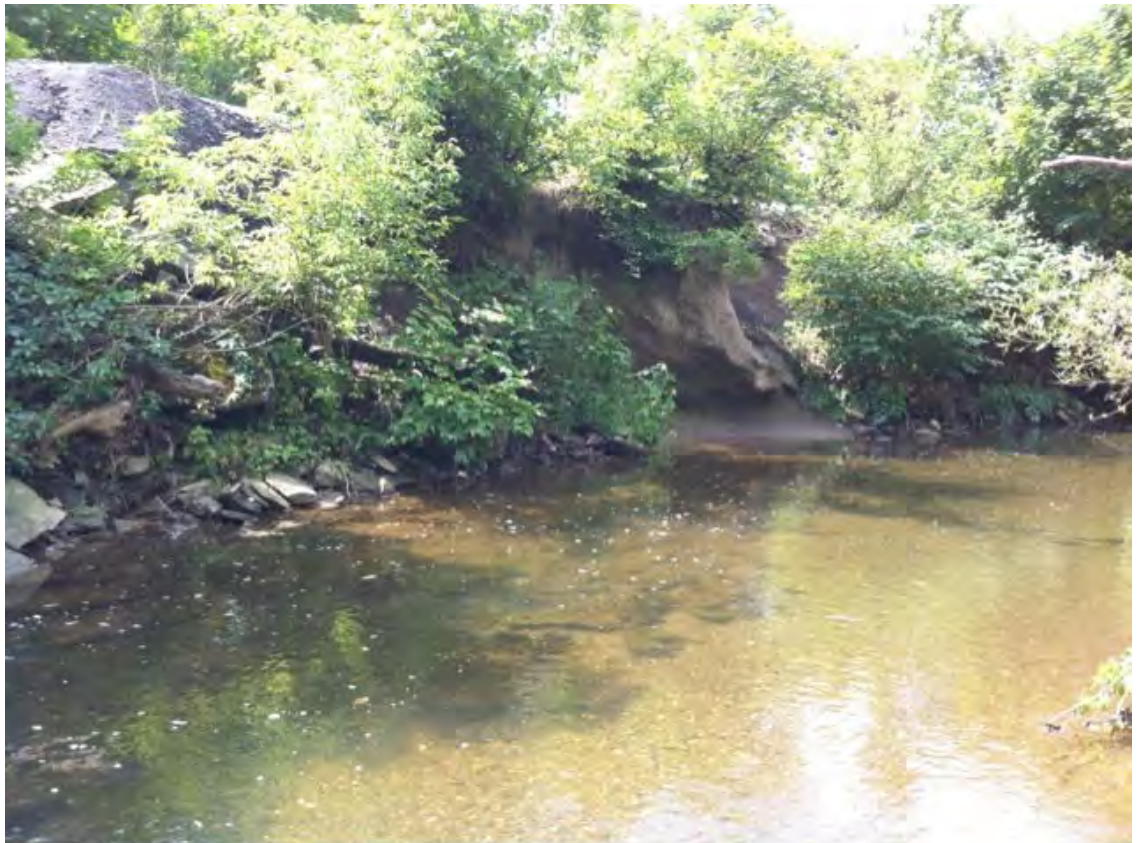
PCL39 - Peters Creek's left ascending bank is being severely undercut just downstream of the pedestrian bridge crossing from Leskers to the Large Park & Ride Lot. The Wheeling & Lake Erie Railroad tracks run immediately adjacent to the left ascending bank from State Route 51 to the Ravensburg Tunnel.
