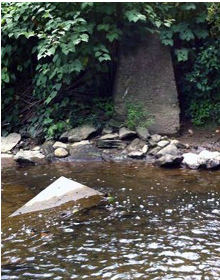
PCM06 - An abutment for what appears to be an old bridge crossing of Peters Creek encroaches on the left ascending bank. Concrete debris within the stream channel and knotweed infesting the bank.
