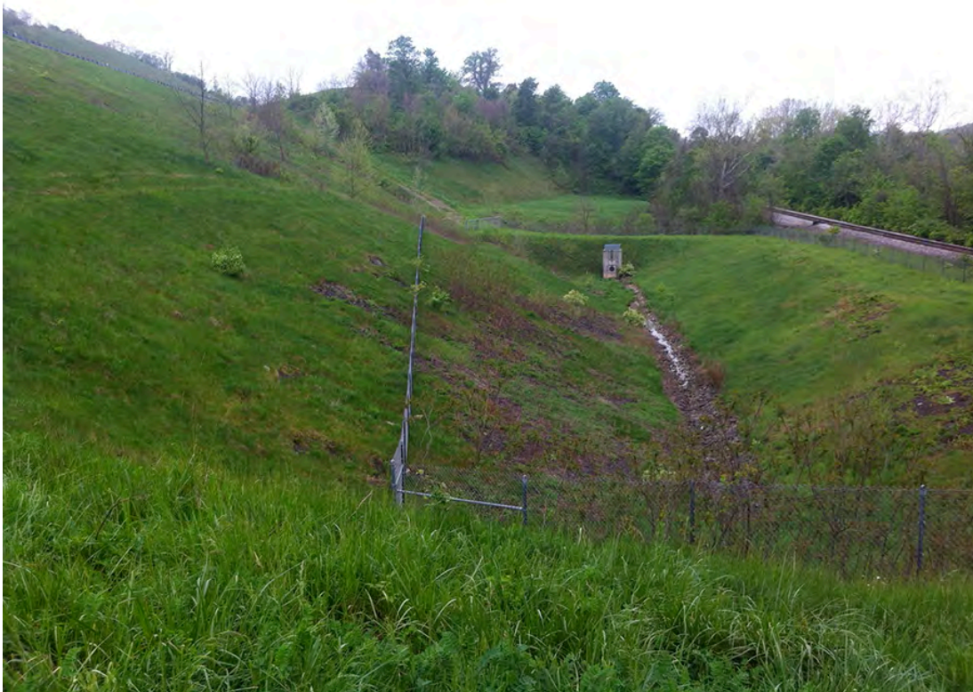
PCU019 – Stormwater detention basin accepting stormwater from the Mon-Fayette Expressway and conveying it to Peters Creek near Snowden in South Park Township.
