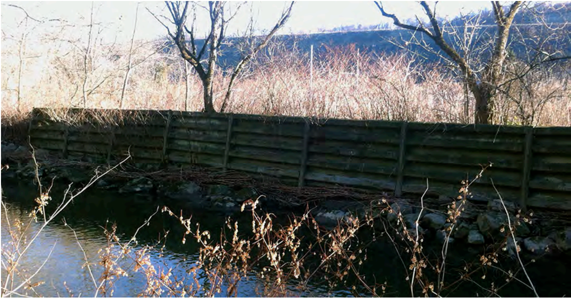
PCM23 – A metal retaining wall at the former National Strategic Mineral Stockpile site supported large piles of strategic minerals up until about 2005. The constructed hillside carrying the Mon-Fayette Expressway can be seen in the background.
