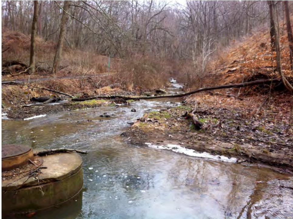
SH08 - Sewer manhole in stream channel. Creates excess erosion, widening of channel and debris jams. Sewage enters stream during heavy rain events.
