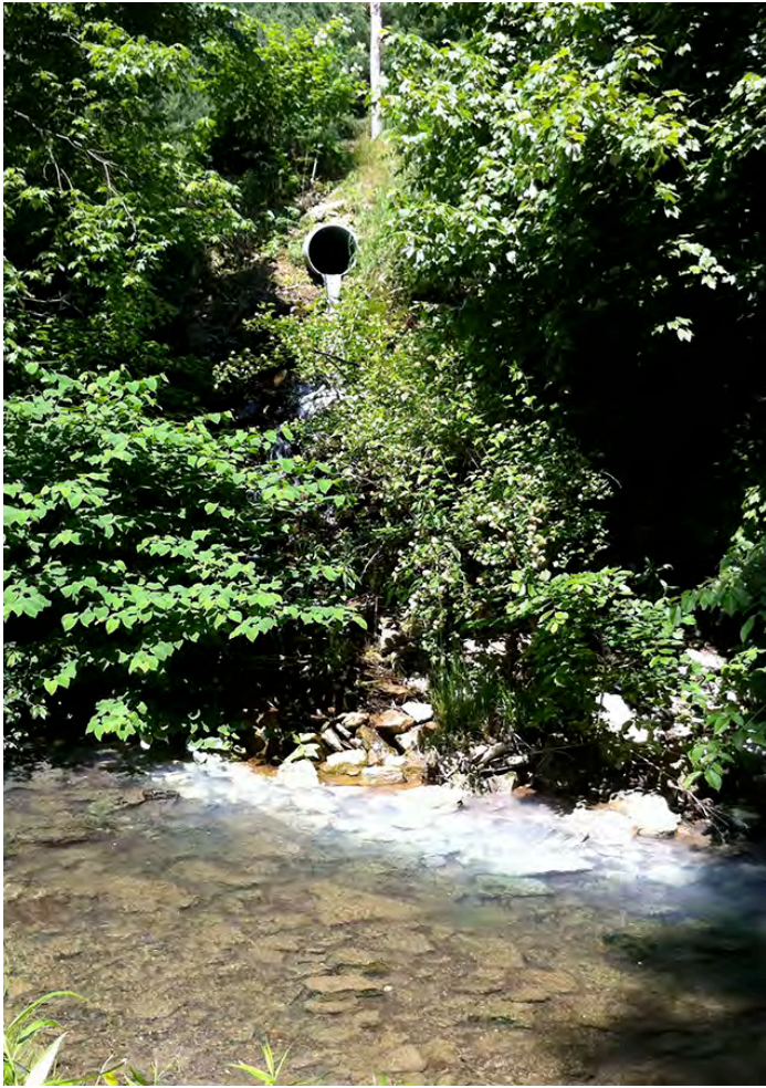
PCU048 – Culverted AMD discharge heavy with aluminum enters Peters Creek just east of Gastonville.
