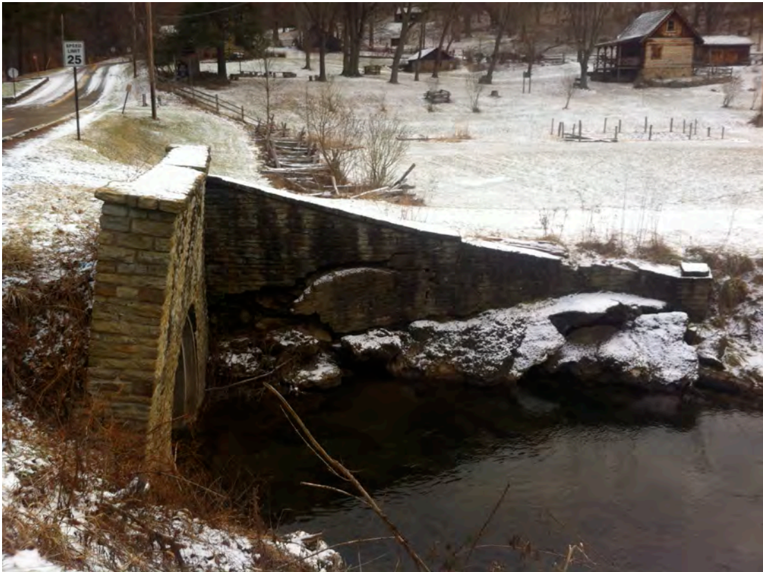
CR48 - Inadequate control of storm water leads to excess erosion downstream and damage to infrastructure such as this culvert headwall and wing wall at Stone Manse Drive.
