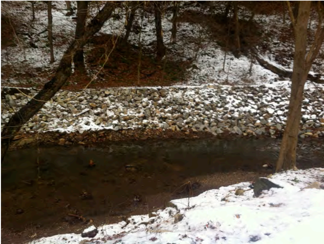
PF27 – An eroding section of Piney Fork’s left ascending bank just downstream of the Montour Trail bridge just east of Triphammer Rd is riprapped to protect it and a sewer line from further erosion.
