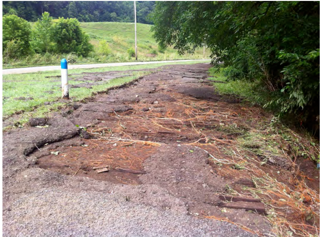
PCL33 – Damage to the Montour Trail due to Peters Creek exceeding its banks during flooding in July of 2013.
