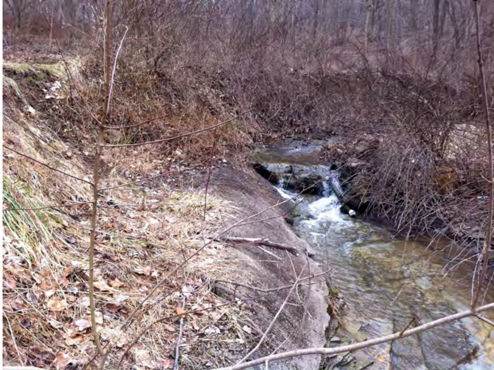
SH09 - Severe erosion on left ascending bank adjacent to trail. There is a 2-3 ft drop here onto a bedrock slide. Attempts are being made to stabilize bank with concrete.
