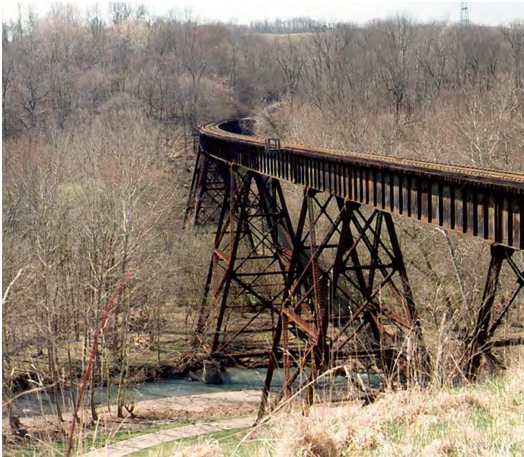
PCU006 – The Wheeling & Lake Erie Connellsville Branch Railroad Trestle abutment is within Peters Creeks channel and causes stream bank erosion at and downstream of the trestle crossing.
