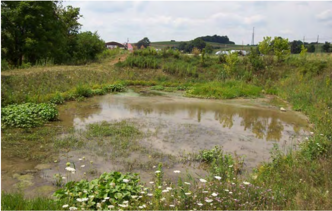
TFT45 – Stormwater detention pond along the Trax Farm Tributary just downstream of Trax Farm Market. The detention pond is filling with sediment which diminishes the basins capacity. Stormwater detention ponds require regular maintenance in order to perform the function they were intended for.
