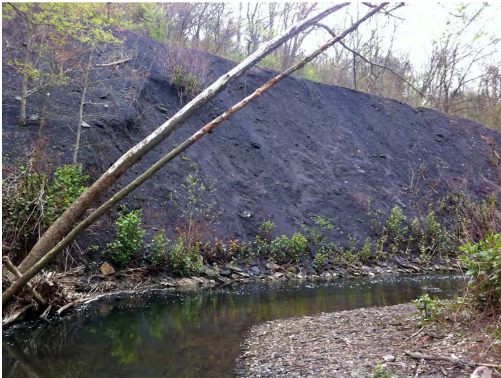
PCU005 – Coal waste pile from old Thompson Mine (circa. 1910–1915) forms left ascending bank of Peters Creek and is eroding into Peters Creek. Little will grow on steep embankment though Japanese Knotweed is attempting to establish on lower slope.
