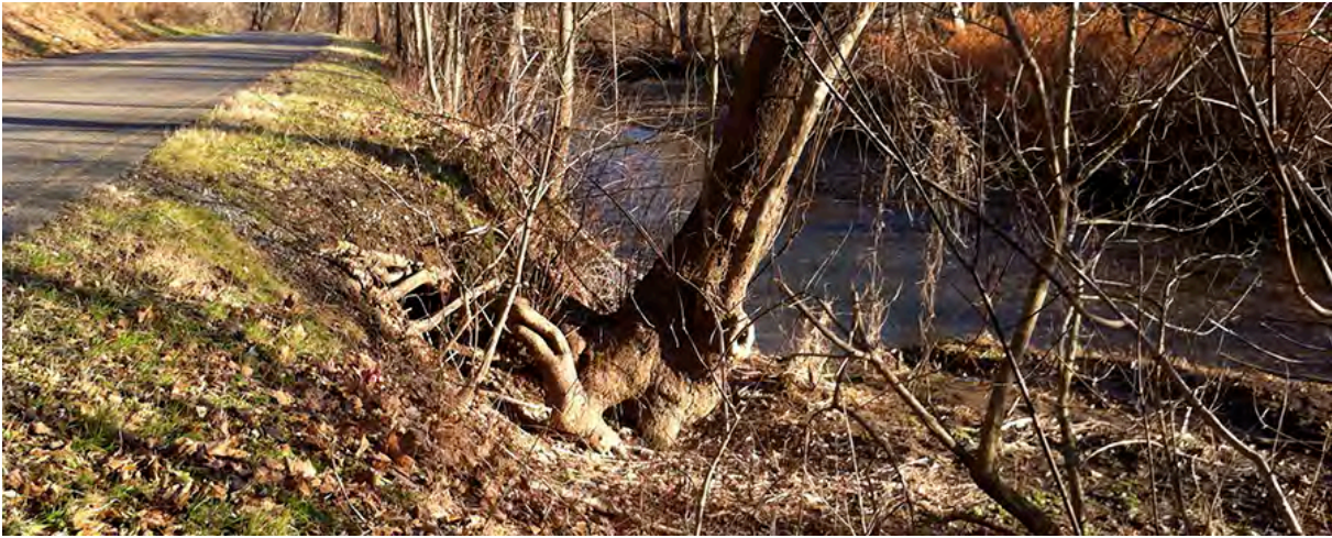
PCM22 – Severe stream bank erosion along Peters Creek Rd just upstream of the Iron Bridge and downstream of a retaining wall along Peters Creek at the now closed National Strategic Minerals Site. The streams energy is directed at Peters Creek Rd and is eroding tree roots and beginning to compromise the road. Jefferson Hills recently received a PA DEP Growing Greener Grant to address this problem with a best management practices solution.
