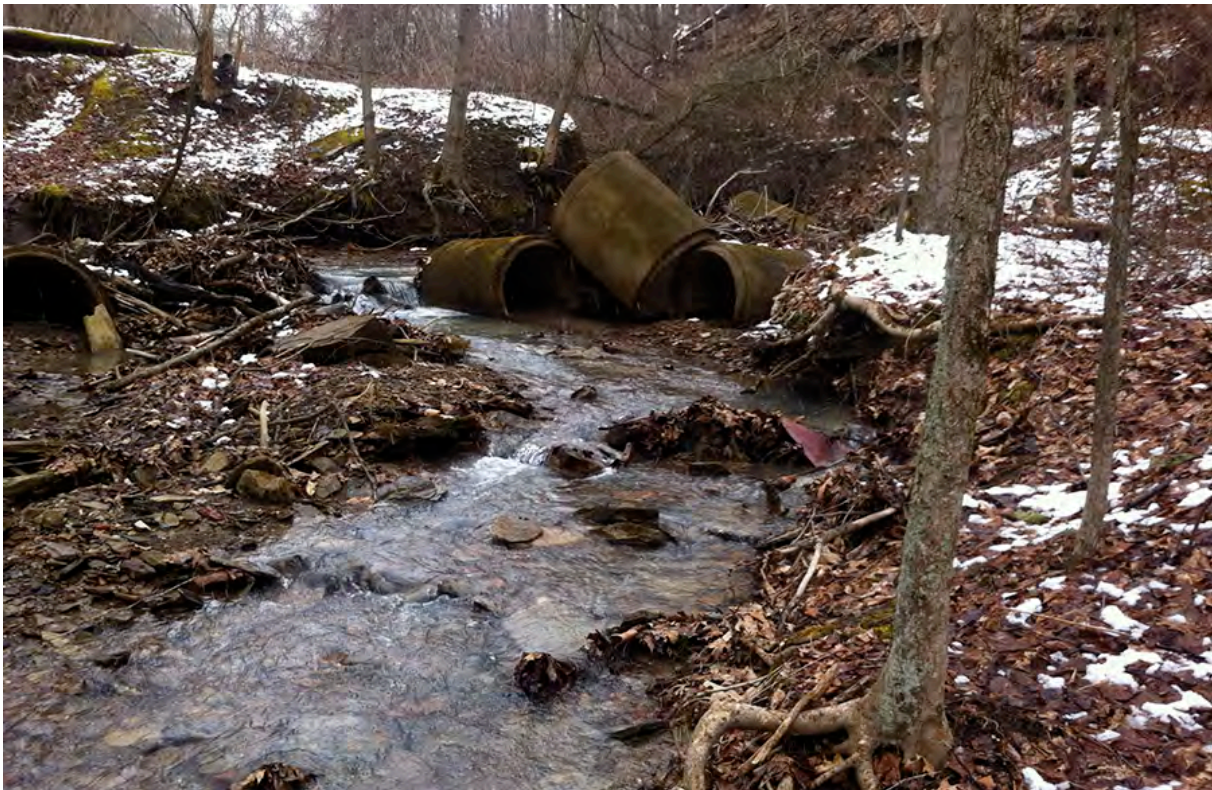
BR37 – A number of sanitary sewer sections encroach on Beam Run's channel and create alteration of flow pattern and erosion.
