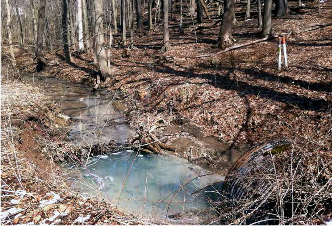
BR57 – A gas line crossing of the stream creates an obstruction and an old culverted undeveloped road crossing encroaches on the channel. The stream is also impacted by abandoned mine drainage at this location.
