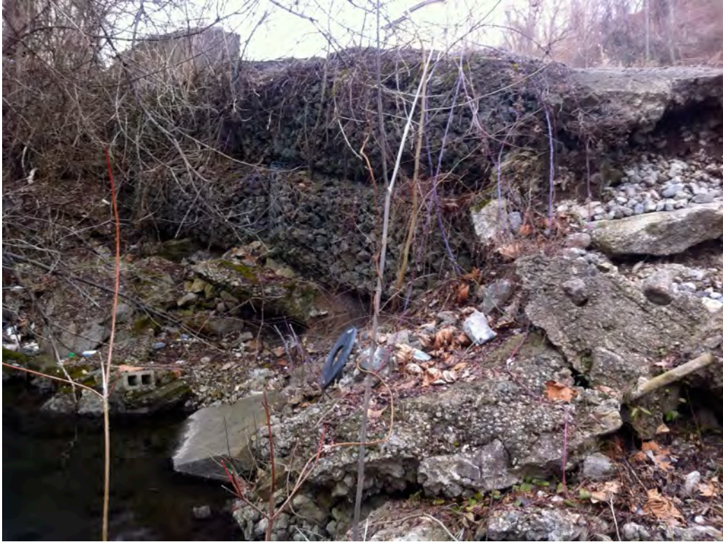
JMT17 – Severely eroding right ascending bank of Jefferson Memorial Tributary just downstream of the streams exit from an approximately 700 foot culvert under a commercial district along Old Curry Hollow Rd. Attempts to stabilize this bank have not been successful.
