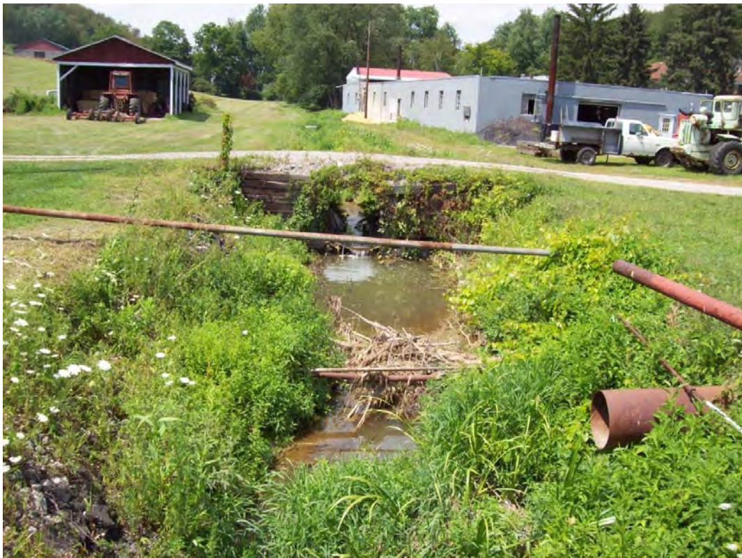
TFT38 – Inadequately sized culvert on a private drive creates erosion downstream of culvert. Piping running across the channel creates a debris jam. Stream mowed right up to stream. Upstream structures built within feet of the stream encroach on the stream.
