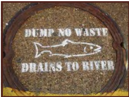
Storm Drain Cover
