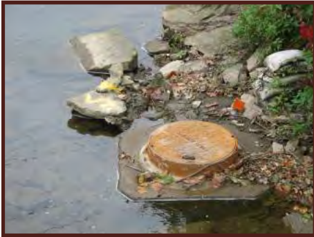
Sanitary Sewer located within Main Stem Pine Creek channel
