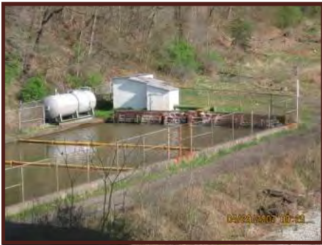
AMD Treatment System Willow Run
