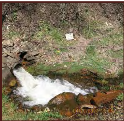
AMD Treatment System Outflow
