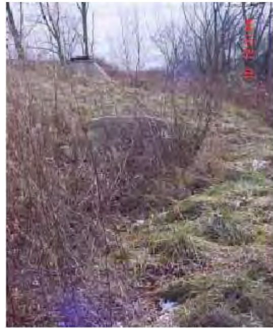
This trench has a subsurface energy dissipator to reduce the velocity of entering stormwater.
