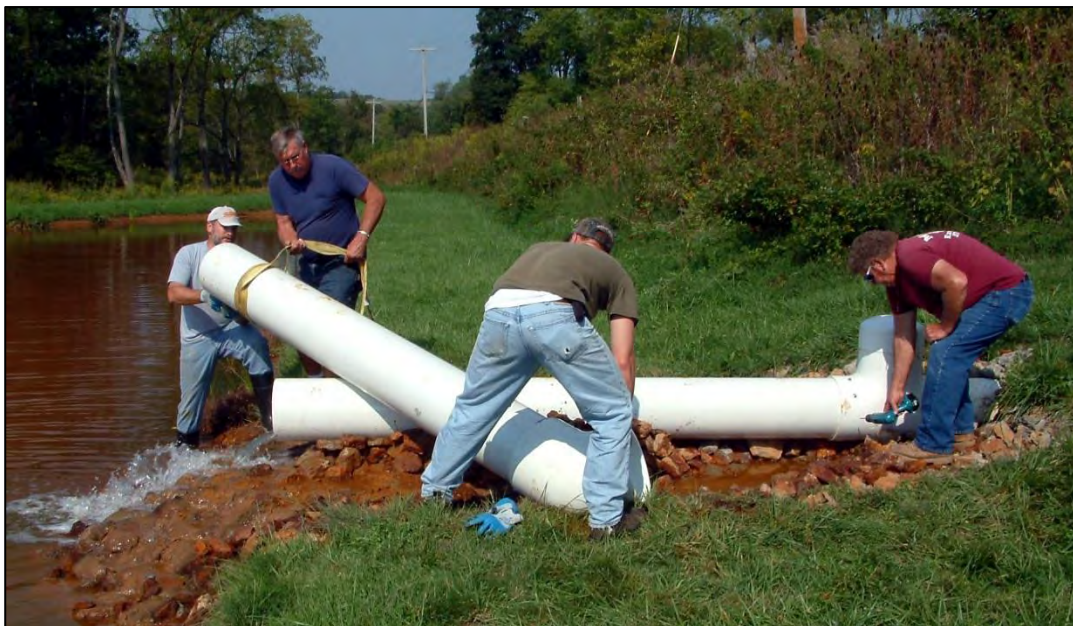
Figure 8.3: Gary Stokum, John Davidson, Jeremy Matinko and Al Moran wrestle with 12" PVC pipe to build an odor-control structure at JB2's lower treatment pond, 9/8/2005.
