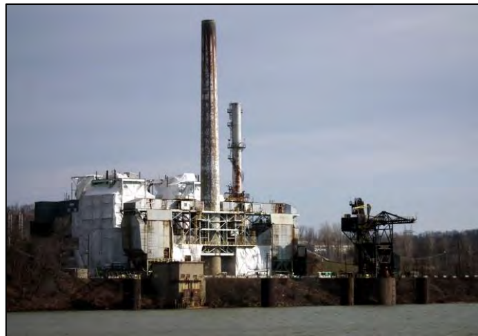
Figure 1.30: The power plant at Horsehead Corporation is being demolished to make way for a petrochemical plant proposed by Royal Dutch Shell. 4/10/2014.
