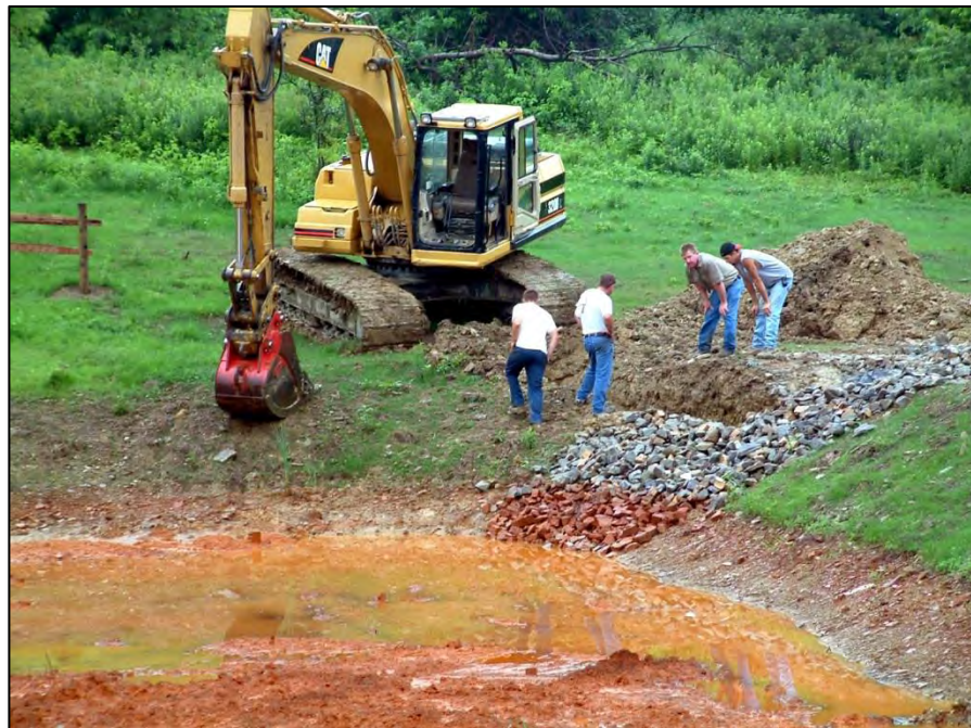
Figure 8.5: A crew from BKG Industries evaluates the need to install a French drain around the eastern side of the Hamilton AMD Treatment System, 7/22/2003. L to R: Michael Kisow, Bill Kisow, Gary Kisow and Jeremy Kapaldo.
