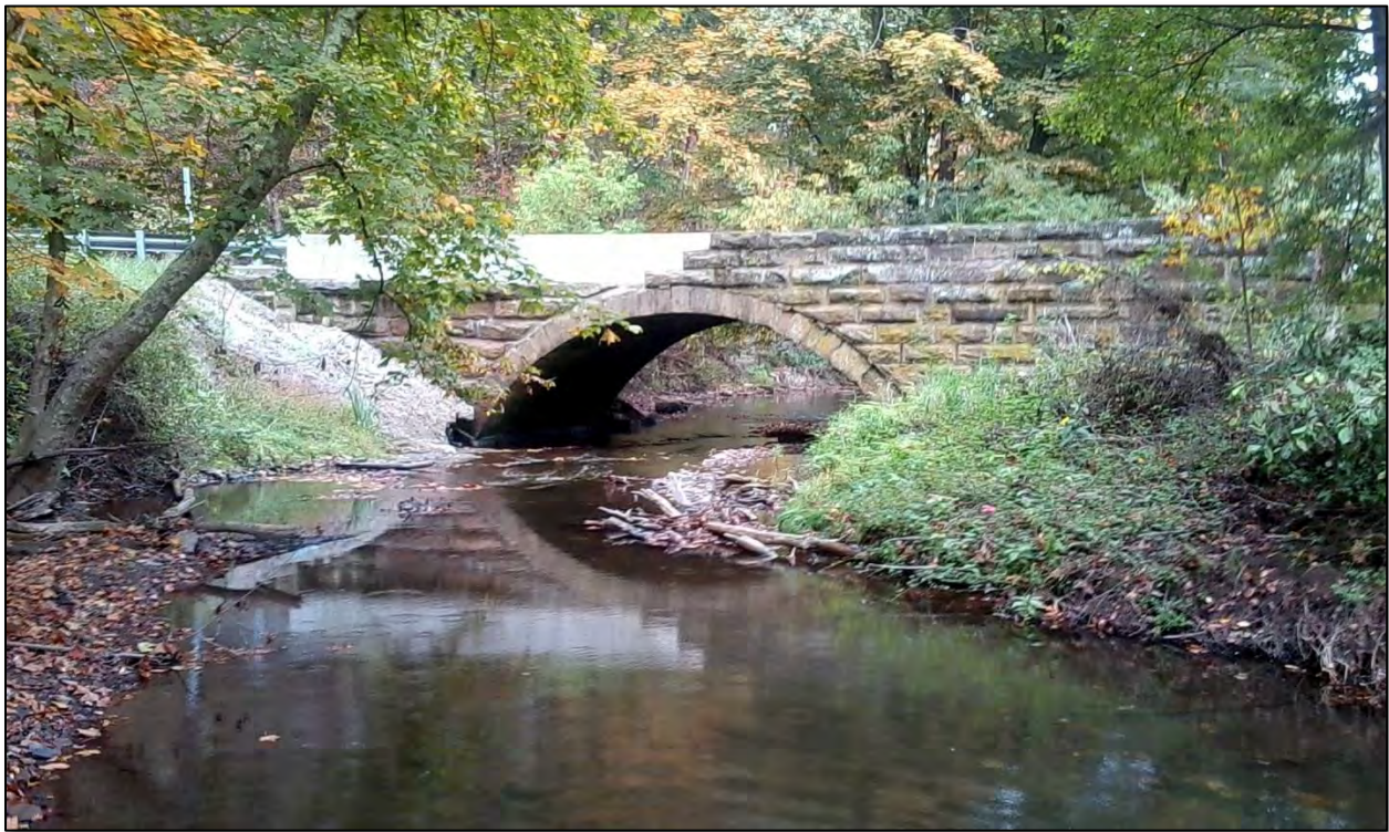
Figure 6.43: A stone arch bridge built in 1936 carries Clinton-Frankfort Road over Potato Garden Run in Independence Township near the Beaver-Allegheny-Washington County lines. Photo 10/3/2013, courtesy of Washington County Conservation District.
