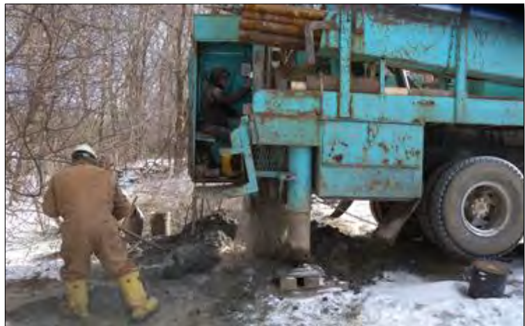
Figure 8.6: Randy McKay and John Rigger of McKay and Gould drill test site EW1 (Erie Mine), hole #4, 1/28/2010. Photo courtesy of BioMost, Inc.
