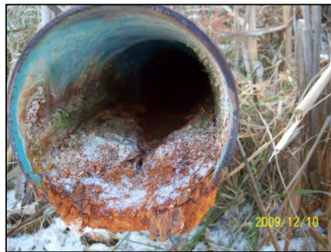
Figure 4.14: A look into the inlet pipe at the Langeloth Bore Hole Passive Treatment System in Langeloth, 12/10/2009. Photo courtesy of BioMost, Inc.
