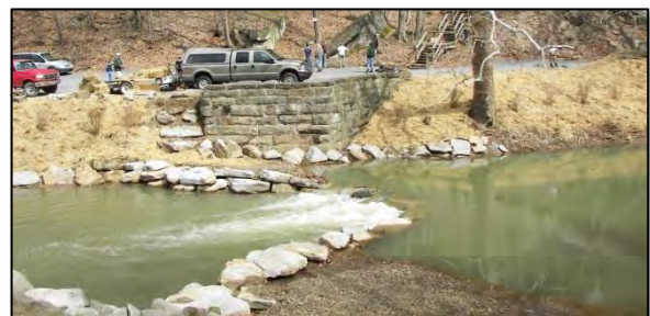
Figure 6.16: Volunteers plant native trees and shrubs near a newly-completed rock cross-vane below the Meadowcroft Rockshelter, winter 2005. Photo courtesy of Washington Co. Watershed Alliance.
