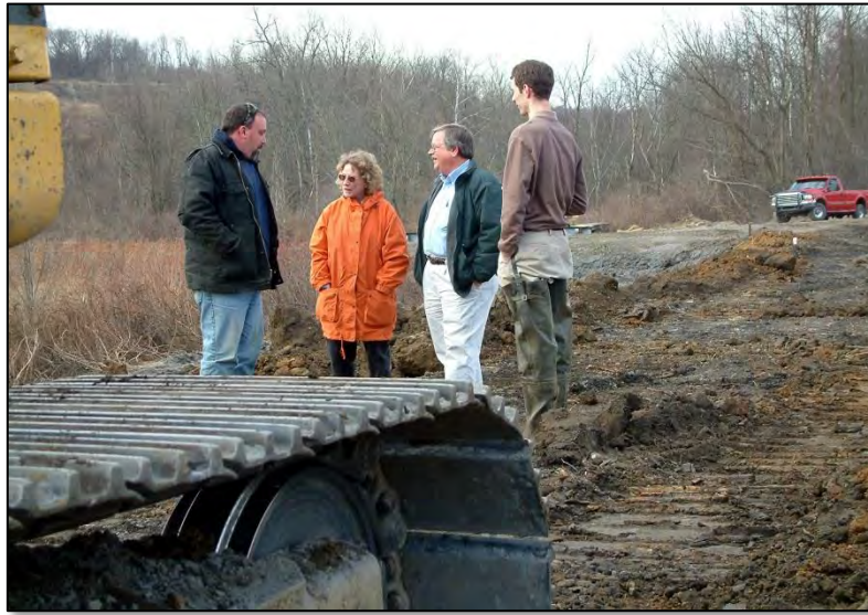
Figure 4.20: Former DEP Secretary David Hess (second from right) tours the JB1 Passive Treatment System under construction near Slak Lane in Smith Twp. L to R: Wayne Fuchs of Quality Aggregates, Margaret Dunn of Stream Restoration Inc., Hess, and Shaun Busler, also of SRI. Photo 12/12/2006.
