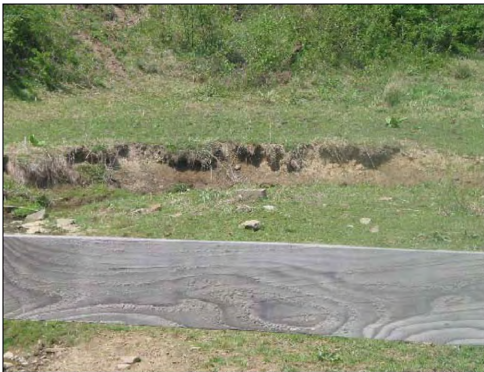
Figure 25. Downstream streambanks are being undercut, and erosion
