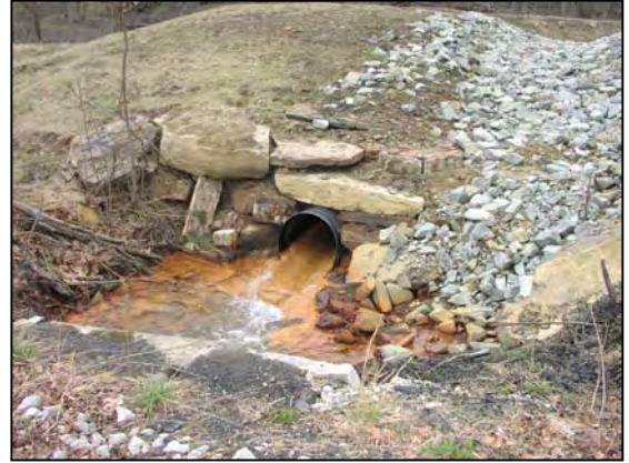
Mine discharge at the Lowber site (Source: WPC 2002)
