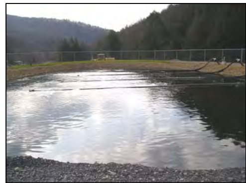
Example of a community sewage treatment system in Broad Top Township, Bedford County, PA
