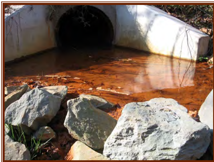
AMD problem with sulfur smell (MR-10 Photo 8)
