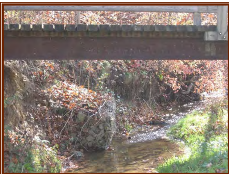
Golf Course Road Bridge; note failing gabion basket (CR-3 Photo 25)
