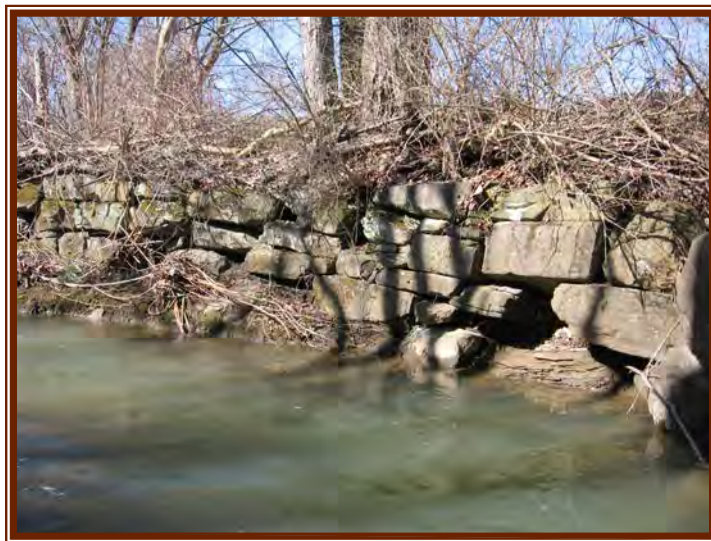
Retaining wall in poor condition (RR-5 Photo 5)
