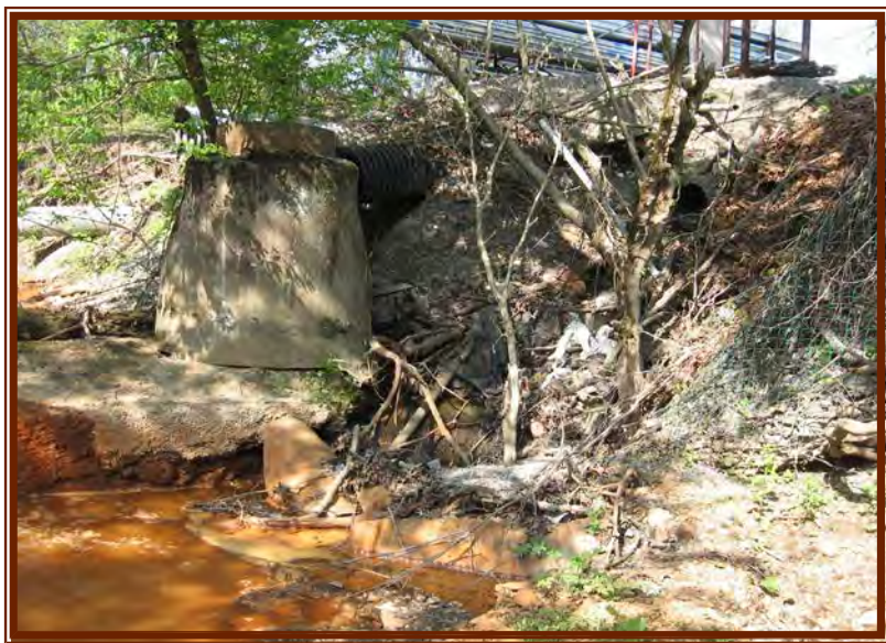
Severe erosion compromising bank stability and CSO System (CR-7 Photo 4)
