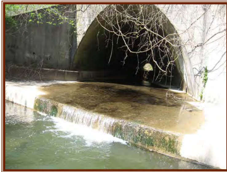
Interstate 79 crossing over Coal Run; note the concrete bottom barrier (CR-8 Photo 4)
