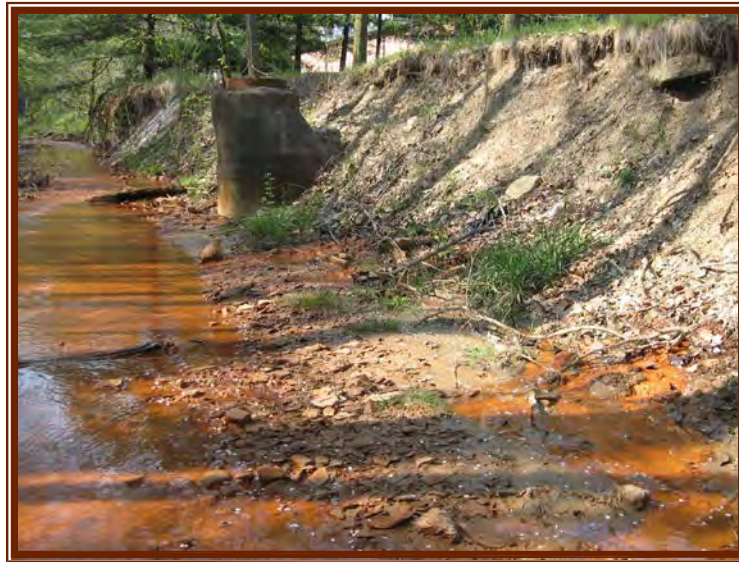
Severe erosion causing bank instability and compromising CSO system lines (CR-7 Photo 6)
