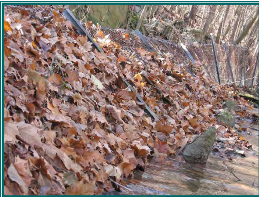
Failing fence (CR-1 Photo 5)
