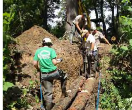
18 Hemlock trees and 5 root wads were used in the completion of 8 structures for this project. Rebar and stone secure the logs in place.
