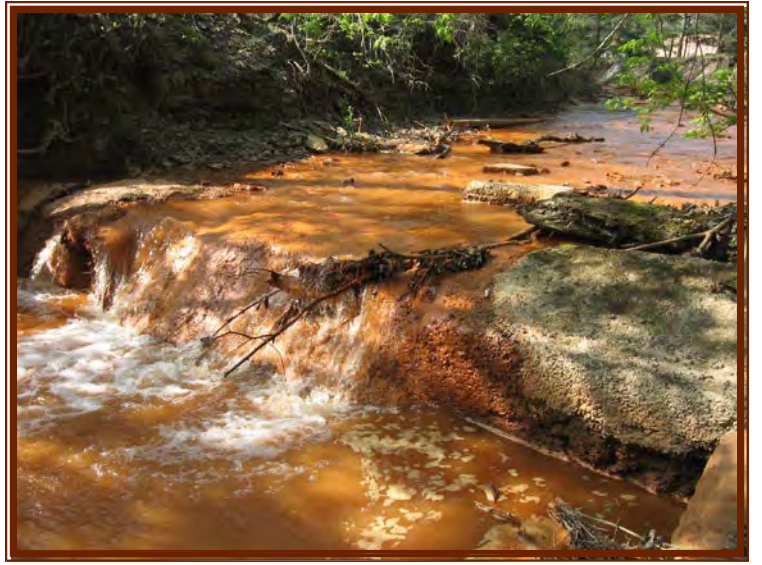
CSO pipe crossing; concrete encased causing barrier to fish passage (CR-7 Photo 5)
