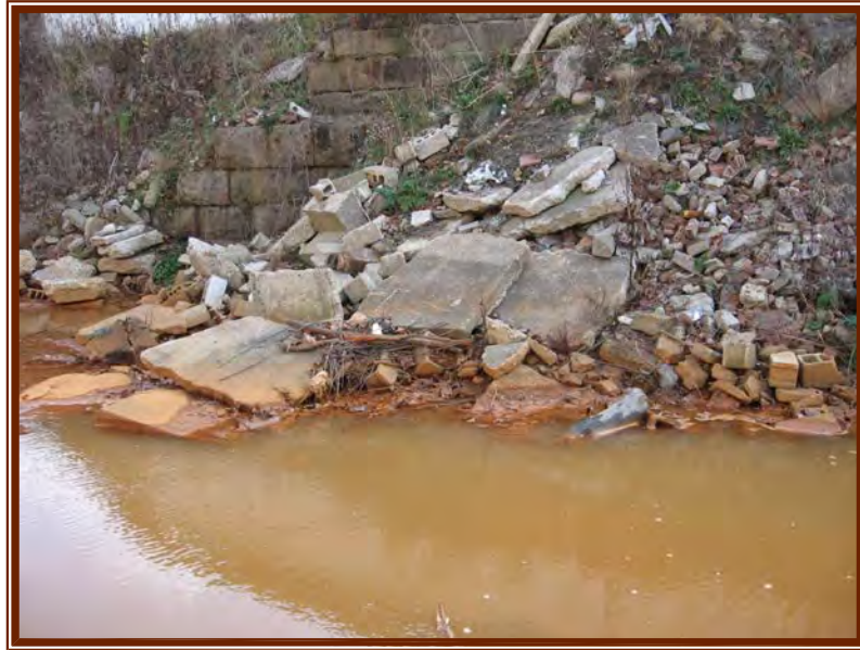
Unstable banks (MR-8 Photo 10)
