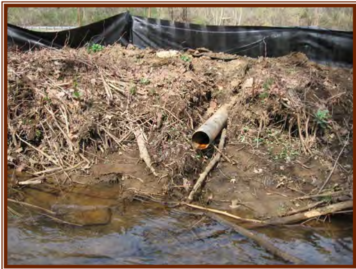
Drainage (RR-8 Photo 5)
