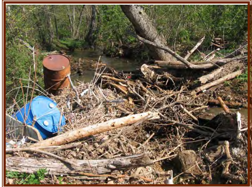
Major obstruction (RR-9 Photo 3)
