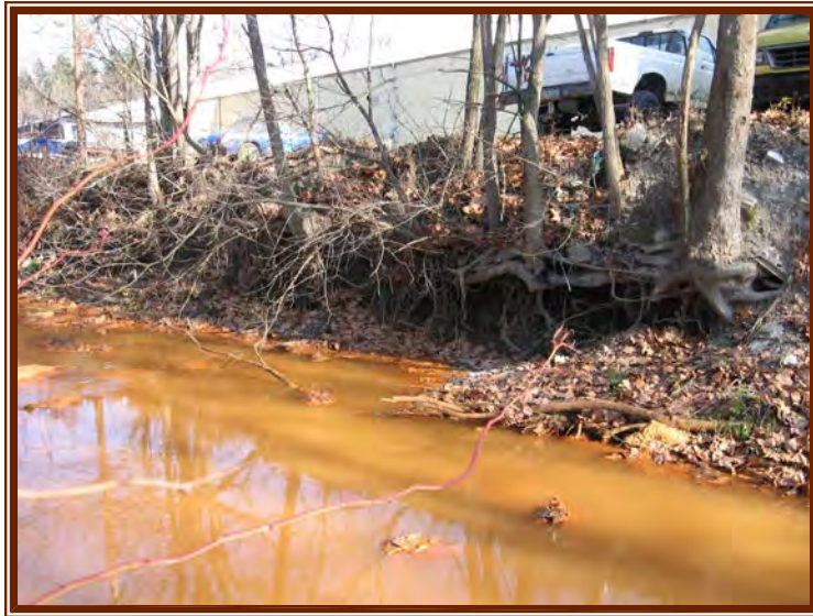
Severe erosion (MR-10 Photo 18)
