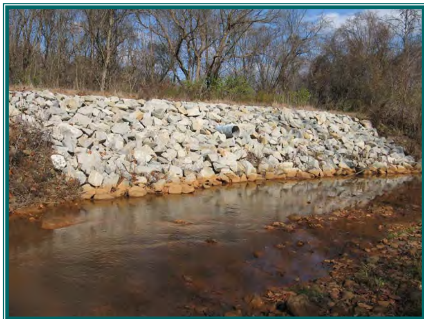
Rip rap and AMD staining (MR-2 Photo 3)
