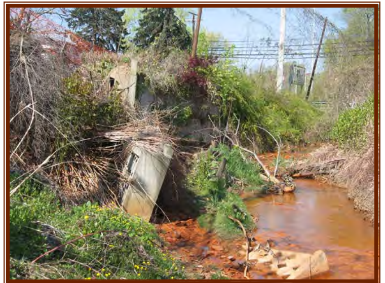
Collapsing retaining wall (CR-7 Photo 13)
