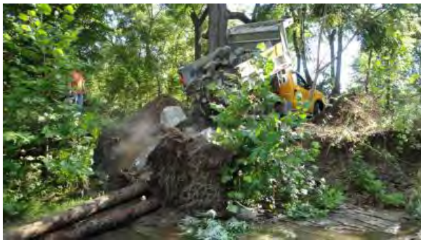
Approximately 120 tons of rock were used over the 3 days that it took to construct the deflectors.
