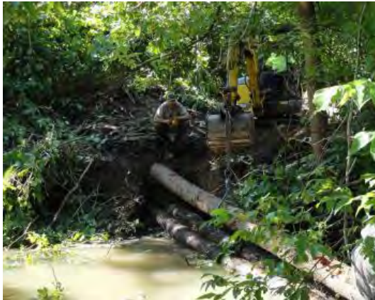
Logs are precisely placed to direct the flow away from the stream bank. Root wads are also sometimes used to create deflectors. 18 Hemlock trees and 5 root wads were used in the
