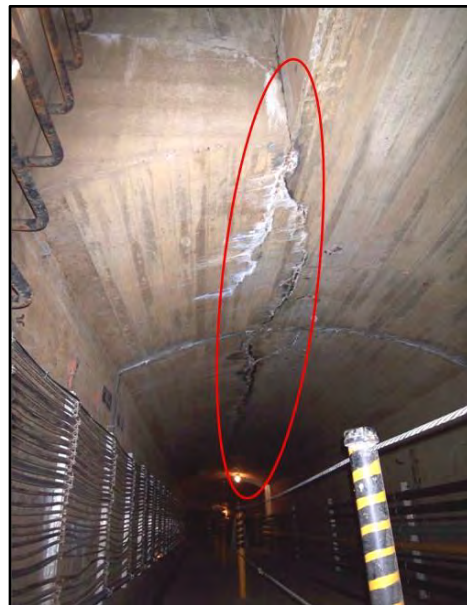
FIGURE ES-9 Montgomery Middle Lock Wall longitudinal cracking
