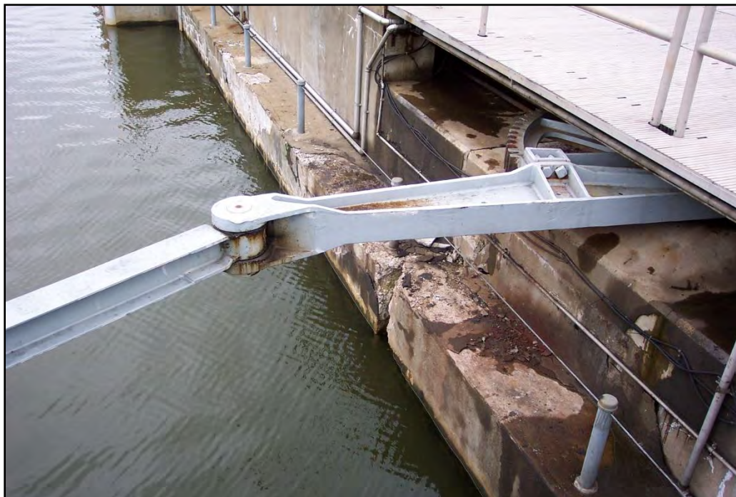
Photo 4-5: Miter Lock Gate Machinery (Arm)
