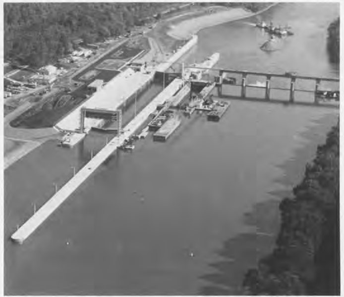
The new lock project under construction at Point Marion Lock and Dam, Monongahela River.
