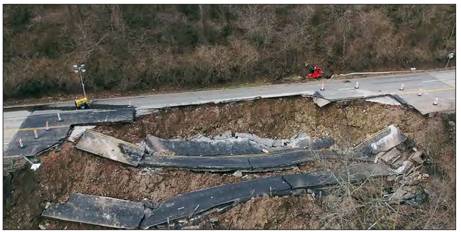
Recent landslide on Route 30, East Pittsburgh
