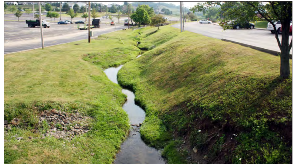
Impaired stream corridor before restoration, Westmoreland County Community College (WCCC), near Youngwood.
