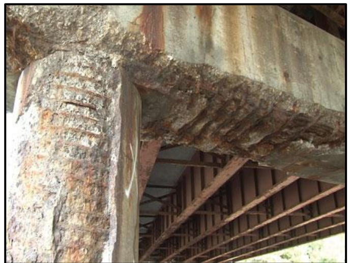
Figure 4: Significant damage from many years of salt and deicing chemical use from a leaking expansion joint. Source: Bridge retrofit using fiber reinforced polymer, cenews.com
