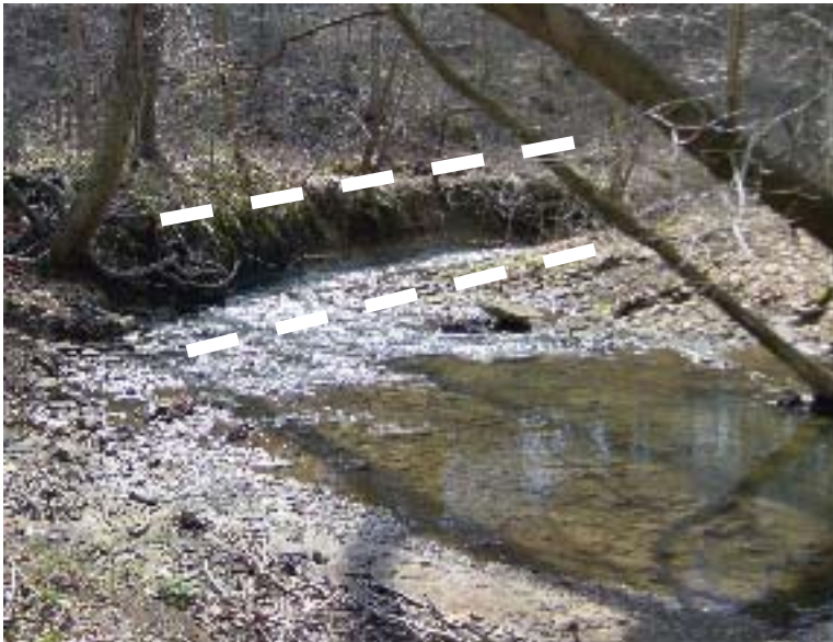
Stream Bank Erosion as a Result of Undersized Culvert
