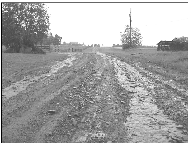
NO GRADE BREAK – Water flows on road causing excess erosion and aggregate loss.
