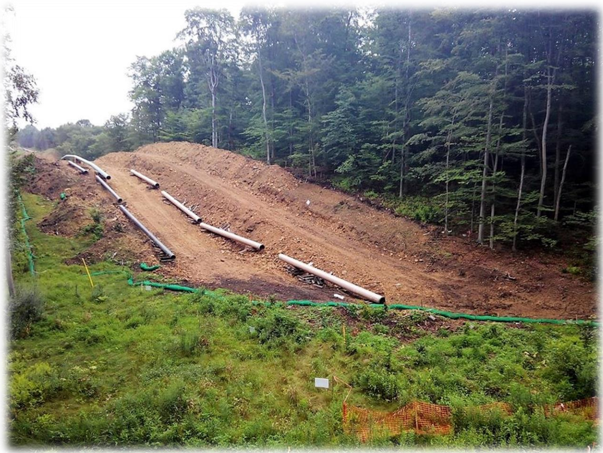
Figure 21 – Sunoco’s Mariner East pipeline crosses the Kiski-Conemaugh River Basin
