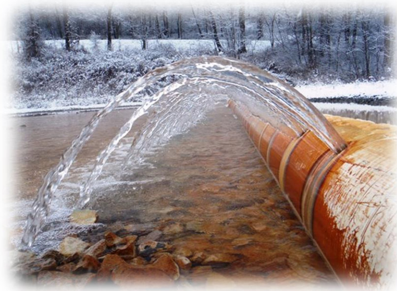
Figure 169 – The influent of the Big Run #2 AMD treatment system forms arches
