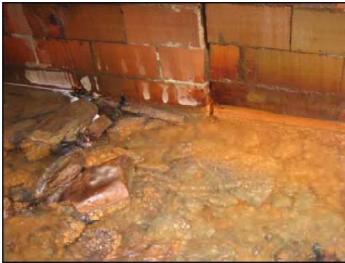
AMD discharges from crack in Route 879 Bridge pier on Bilger Run.
