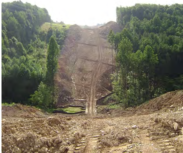
Figure 68. Installation of the REX pipeline in the South Fork subwatershed near New Castle.
