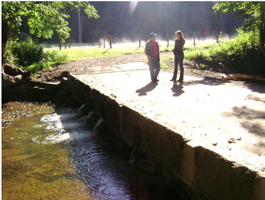
Figure 133. Submarine bridge through Crabapple Creek (RM 3.3). Photo source: Belmont Soil & Water Conservation District, 2013.
