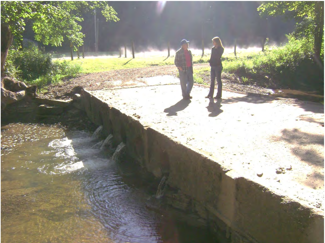
Photo 1 Washington Township Road 84 submarine bridge on Crabapple Creek. Notice the culverts and the water level of the stream.
