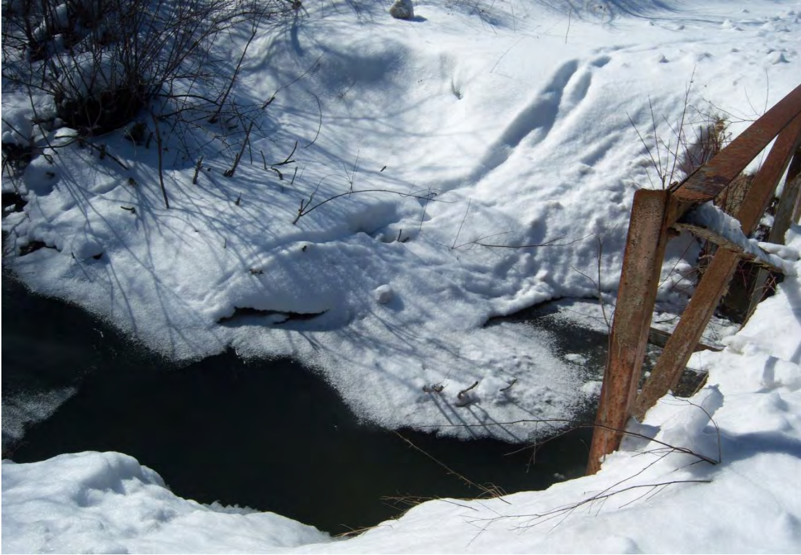
Figure 87. – Close up view of slumping bank; alder growing out of sediment hummocks, mid section of the headwaters tributary of Chest Creek (looking upstream)
