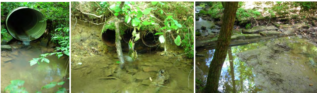
5823: Perched culvert outlet, relic undersized pipes, relic log dam (separate locations on 5823).
