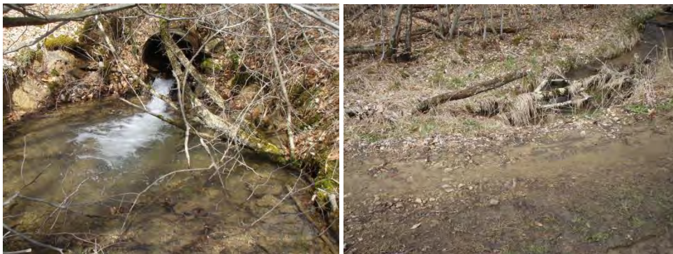
6041: Several undersized/perched culverts for multiple sinuous DGR crossings. Outlet on the left and clogged inlet on the right.
