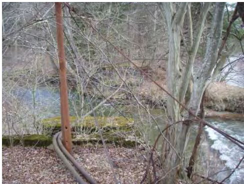
6049: Relic bridge abutments and a pipeline form a constriction and low potential AOP barrier.
