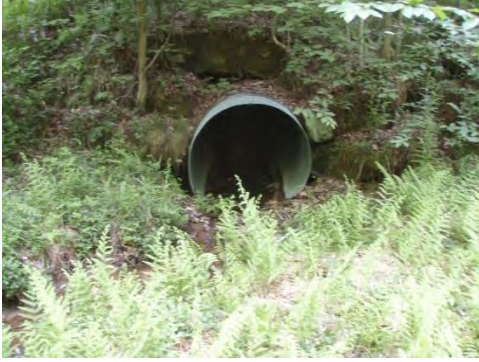
6164: Undersized culvert on Forest Road 462A.
