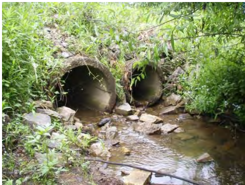
6079: One set of double culverts at their outlet. Permission and logistics prevented further survey of the 5+ other AOP barriers on this segment. (Future endeavors may reap different results).
