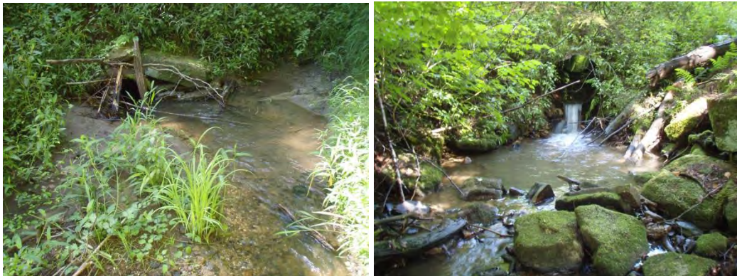
5816: Culvert inlet (left) and outlet (right) posing an AOP barrier. Culvert is perched and clogged.
