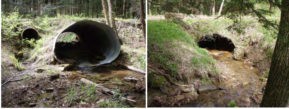
6052: Recently replaced culvert is perched with substrate falling short of pipe outlet (left). Erosion near inlet (right).
