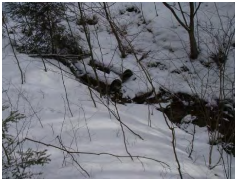
7202: Two dilapidated culverts on a gasline right of way.
