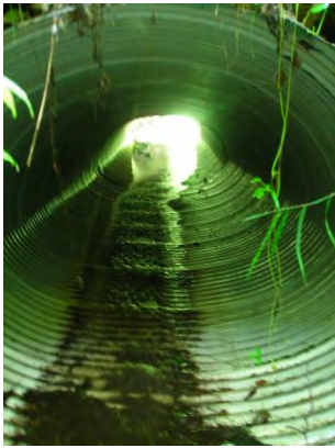
5806: Culvert posing an AOP barrier. Culvert lacks suitable substrate for AOP passage.
