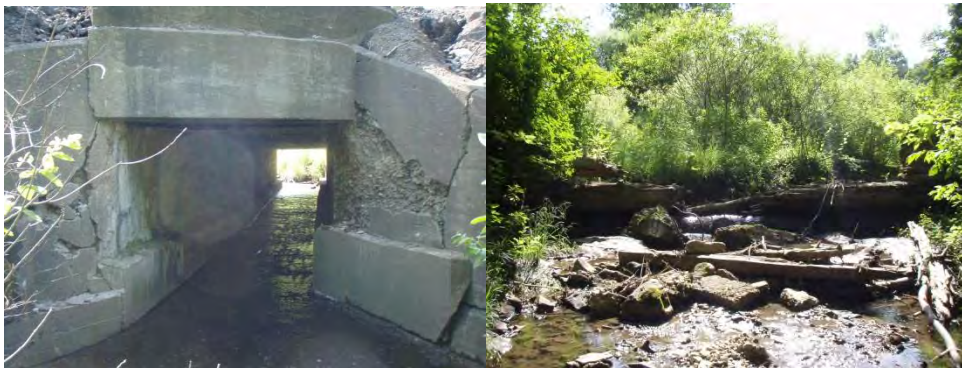
6099: Undersized box culvert under State Route 66 (left); old, breached dam (right).
