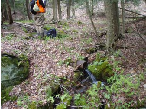
5978: Perched culvert outlet, 1 of 3 channels on this UNT at this inactive pipeline crossing.
