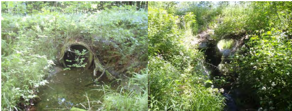
6142: Undersized culvert on intermittent section of stream in headwaters (left), undersized squash pipe at Forest Road 473 crossing (right).
