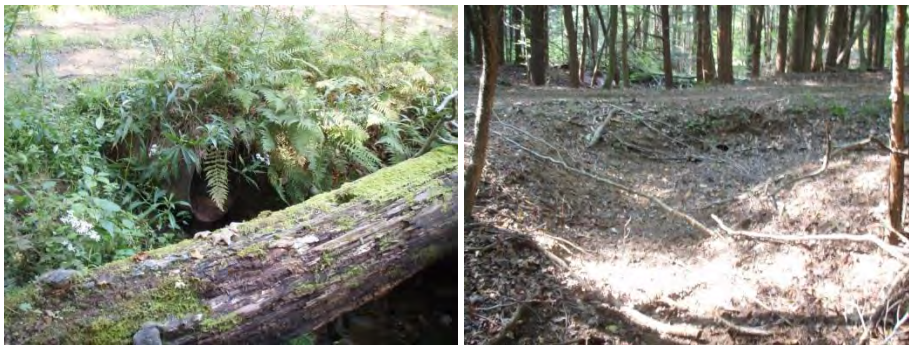
5869: Perched culverts downstream (left) and upstream (right, near ephemeral point of stream)
