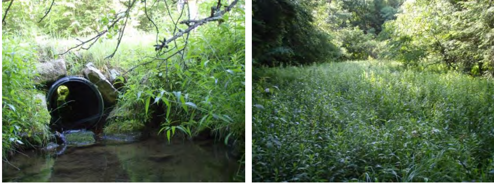
6110: Undersized culvert at West Kane Road (left); sedimented basin of relic log pond (right).
