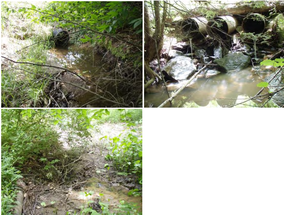
6114: Clockwise from bottom left: Inlet to underground section; outlet of undersized culvert on Pennsylvania Avenue, three undersized pipes on private gas road crossing.
