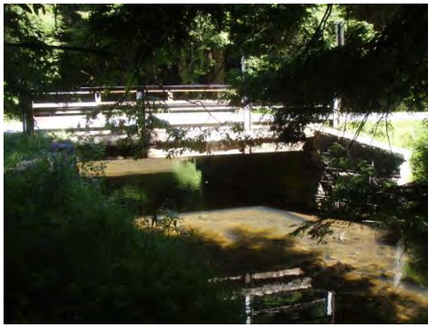
6141: Potential AOP barrier due to narrowness and lack of floodplain beneath bridge.
