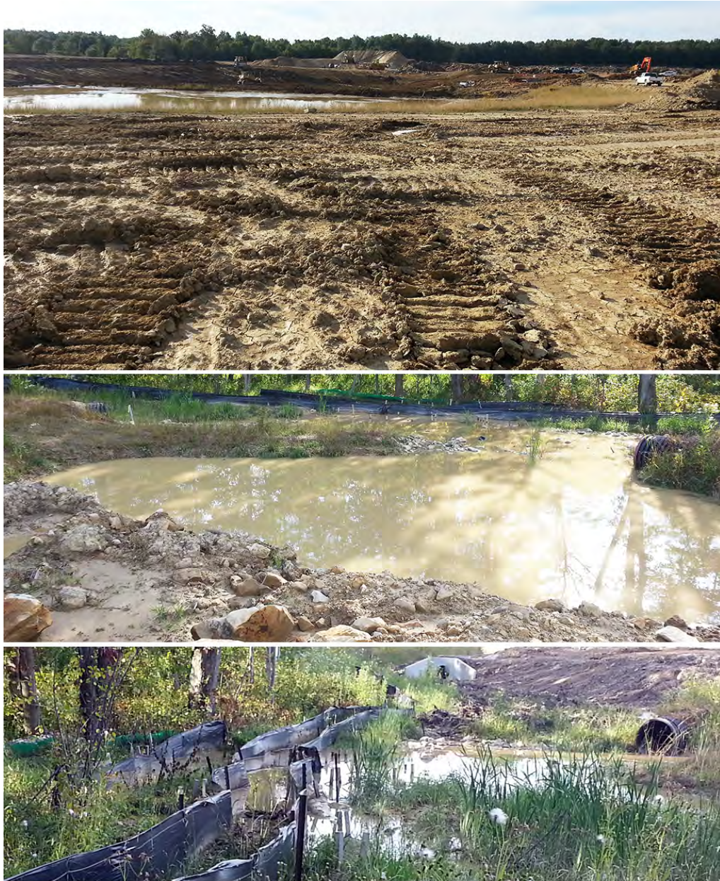
Figure 25 — The Mahoning Valley Race Course construction site, September 2013. Turbidity in Fourmile Run and the Mahoning River were attributed to this location. A day before the photographs were taken, the large basin in the upper photo had been pumped out, overtopping the silt fence in the lower photos.
