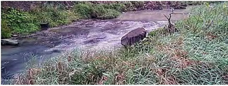
Figure 24 — Fourmile Run upstream from Salt Springs Rd. (RM 0.7) September 2013. Perpetual turbidity emanating from the Mahoning Valley Race Course construction site degraded habitat quality in Fourmile Run and in the Mahoning River.
