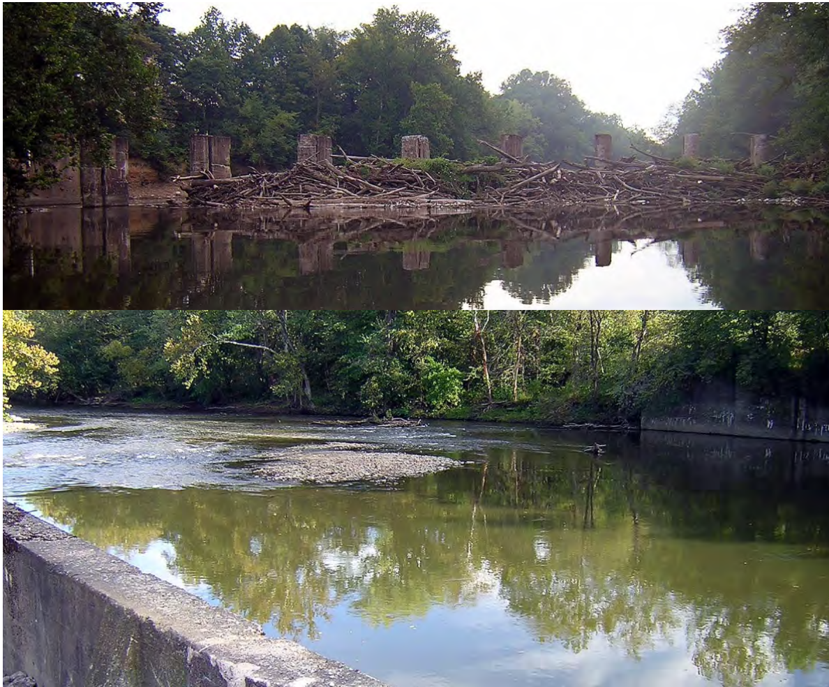
Figure 22 — In 2013, the First Energy Corporation removed 12 concrete bridge piers, logs and trash in the Mahoning River downstream from Lowellville (upper photo). The site near the OH/PA state line is now safer for recreational boating and exhibits improved stream hydrology (lower photo).
