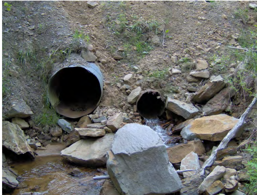
Culvert pipes under Rock Run Road. Note the lack of vegetation to stabilize area.
