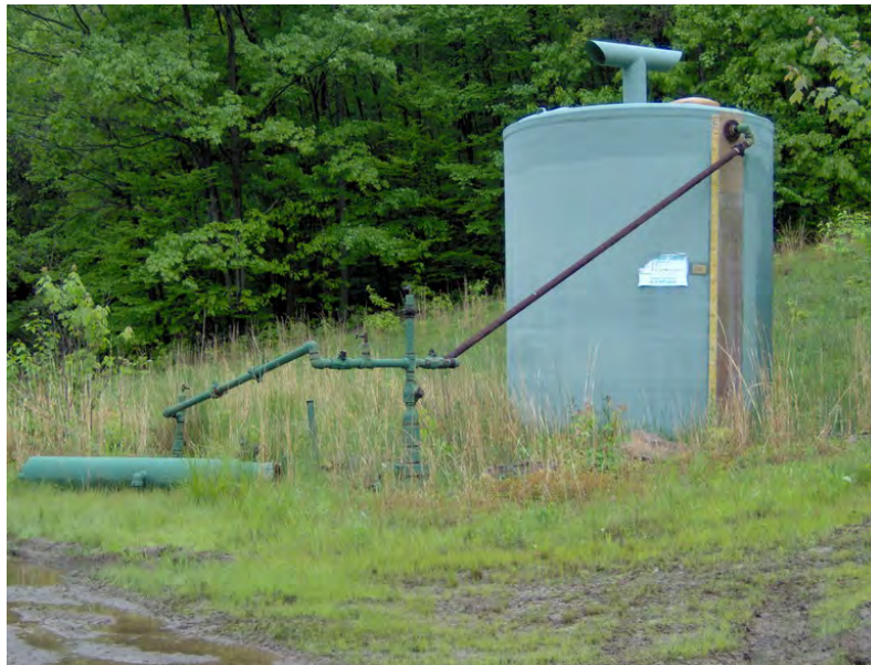
Gas well located along Bad Tributary
