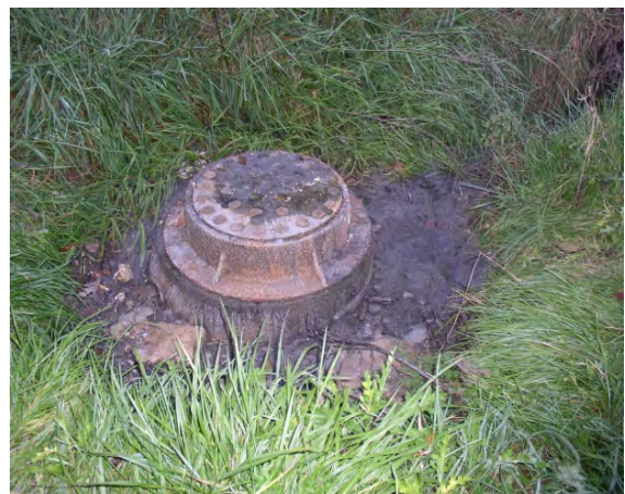
Figure 13. Manhole overflow due to high flows, near Liming Creek.
