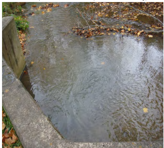
Figure 14. Solids discharge from the Cadiz WWTP outfall 001, Sally Buffalo Creek.
