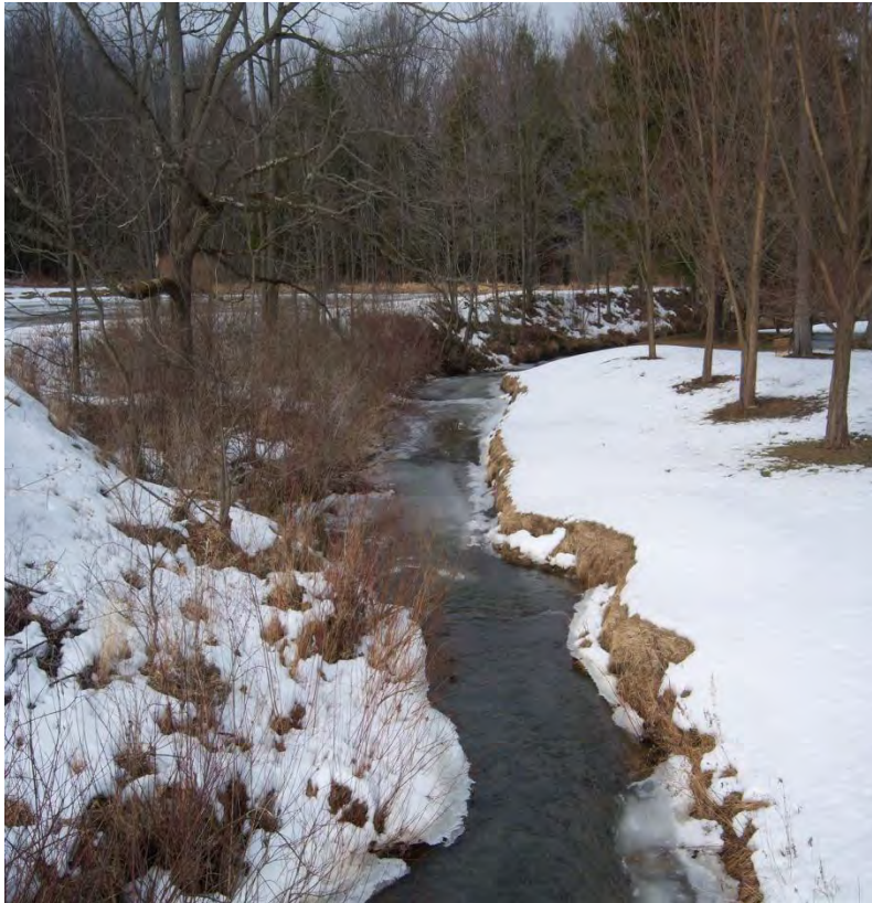
Figure 44. – Bank slumping and high prone area for erosion, above mouth of Slate Lick Run and confluence of Burgoon Run (looking downstream)
