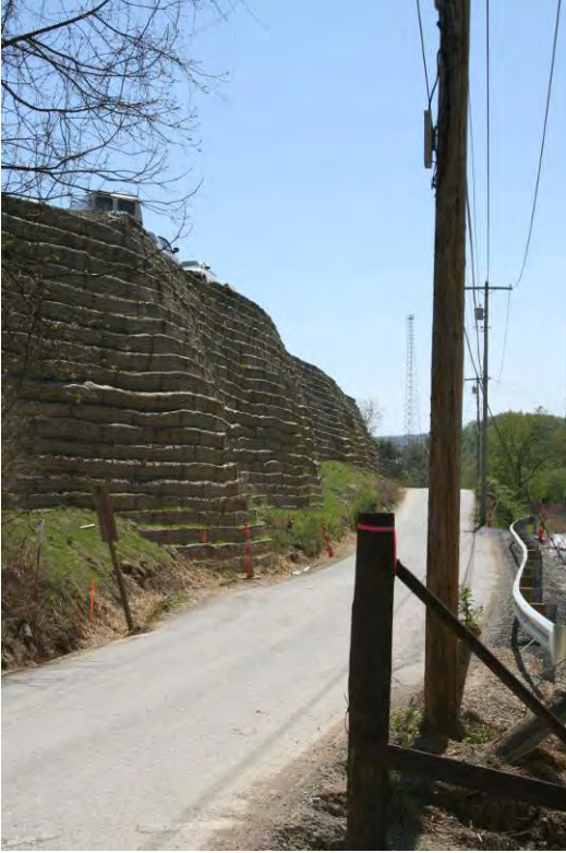
Figure 25: This photograph shows a poorly constructed retaining wall along West Run.
