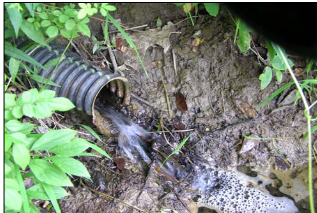
BR1 Discharge after Treatment System
