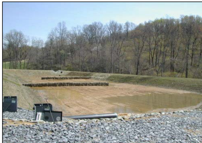
Big Run #2 Treatment System
