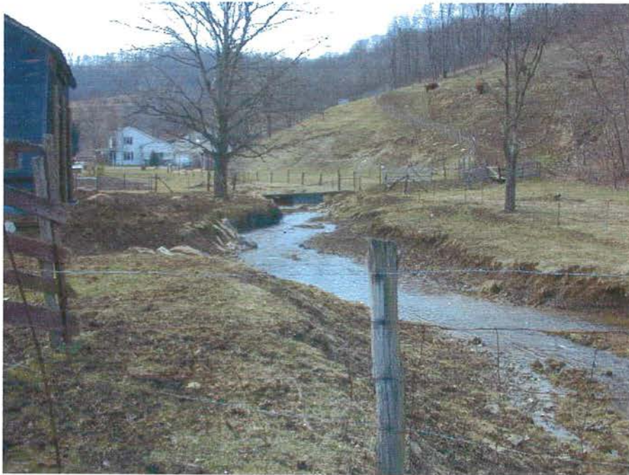
Figure 10. Another example of bank erosion in a pastured area on Rudolph Run.
