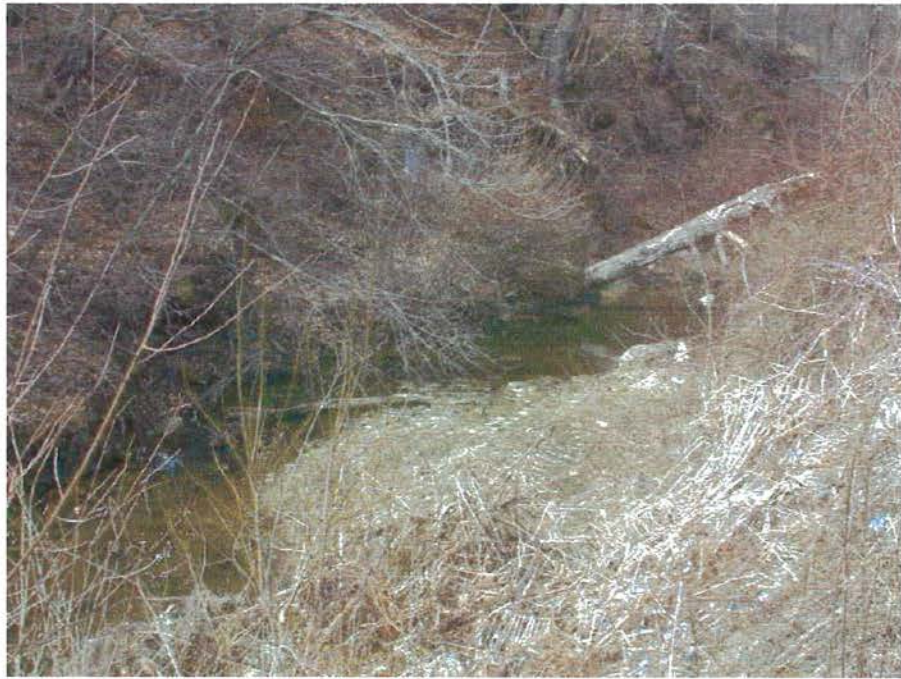
Figure 8. Obstructions in the Rudolph Run stream channel could cause flooding behind accumulated debris.
