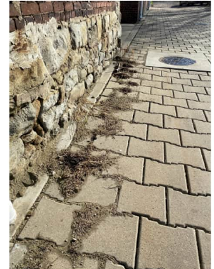
Pavers clogged with silt, weeds growing
