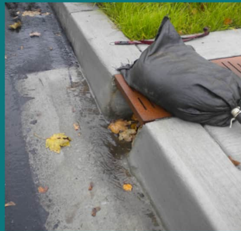
Apron not depressed enough – bypass!
