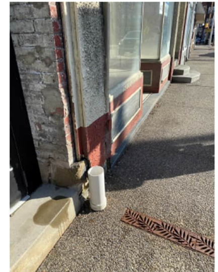
Disconnected roof leader
