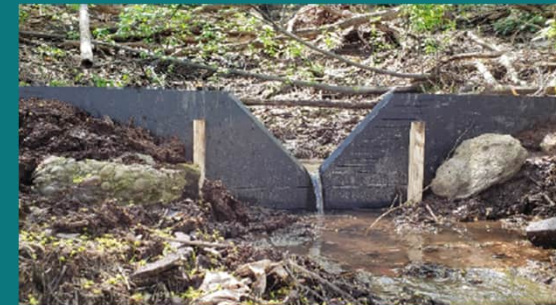
V-notch weir facilitates flow measurements in an irregular channel (image: PWSA)
